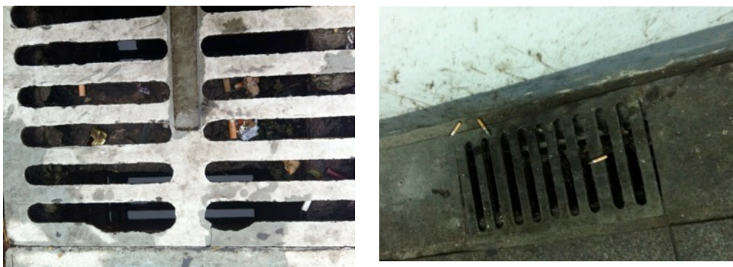
Figure 7.9 Photos of drains exposed to passengers on West Square (left) and Connection Tunnel (right) in Wuchang
