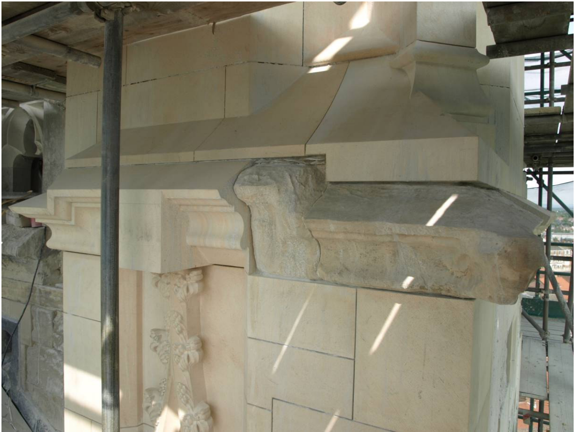
Figure 468: East Front, south butterss, Level G after renewals
