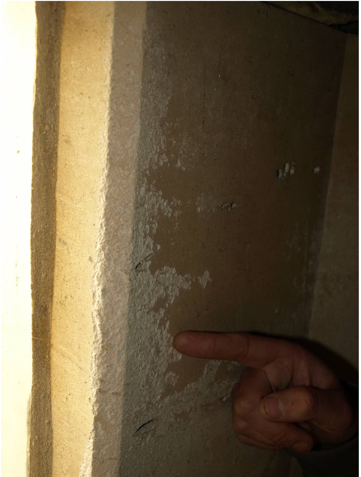
Figure 438: Surface decay of new magnesian limestone indents, Howden Minster Chapter House
