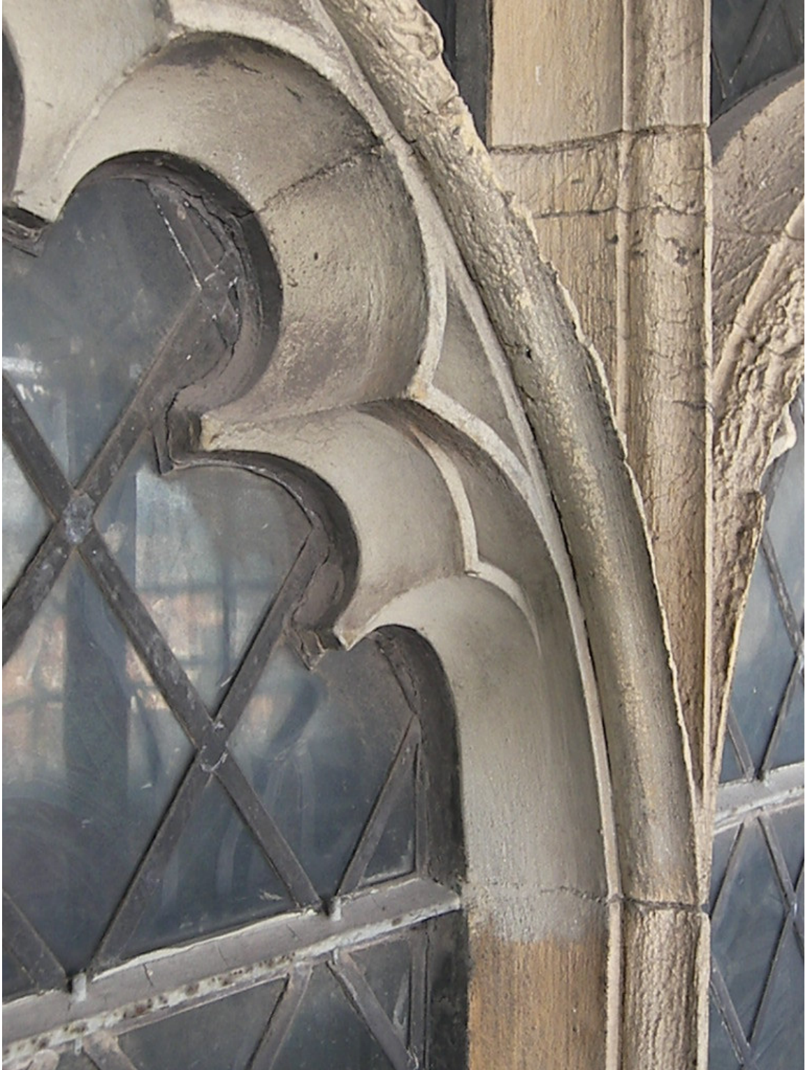
Figure 153: Great East Window masonry bearing grey-green mineral paint
