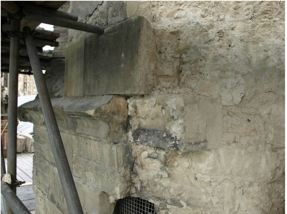
Figure 284: East Front, south buttress-turret Level G during dismantling showing indented nineteenth-century stringcourse
