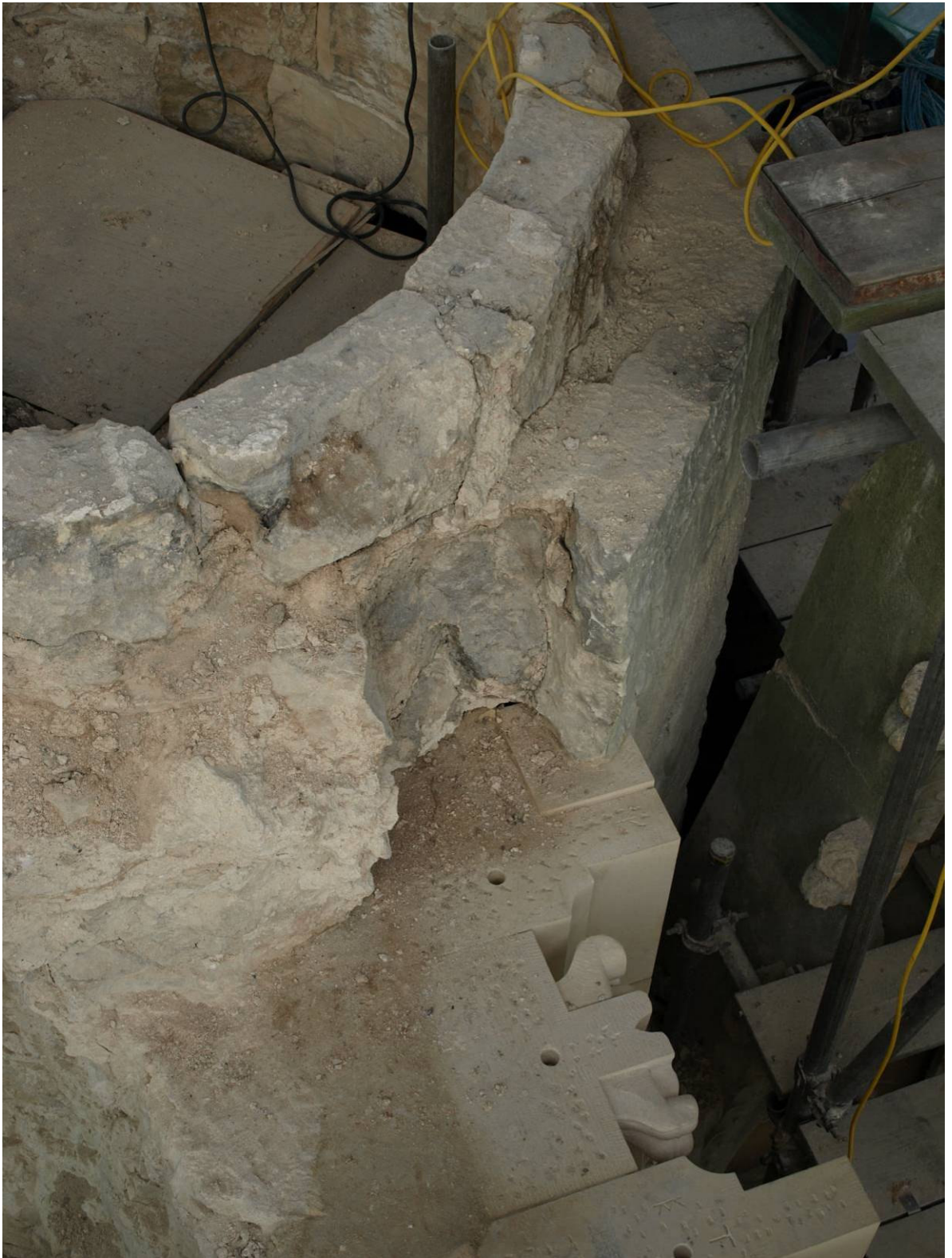
Figure 283: East Front, Level H of south buttress during rebuilding showing medieval broach on inner skin with re-clad exterior
