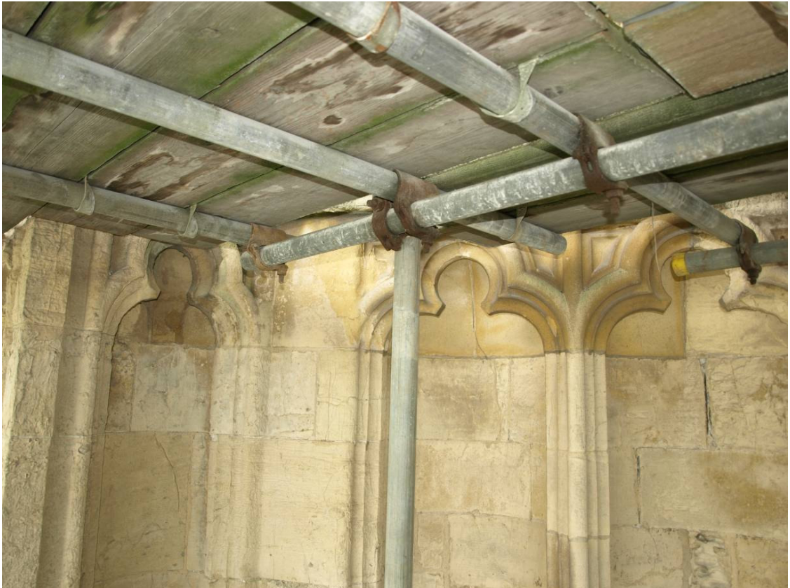
Figure 224: East Front, junction between south-east turret and masonry above south aisle, Level C
