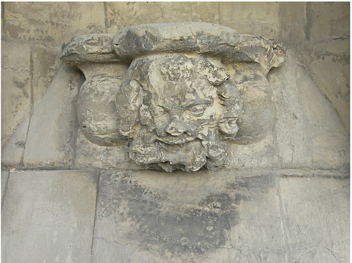
Figure 434: East Front, niche-base before cleaning trials
