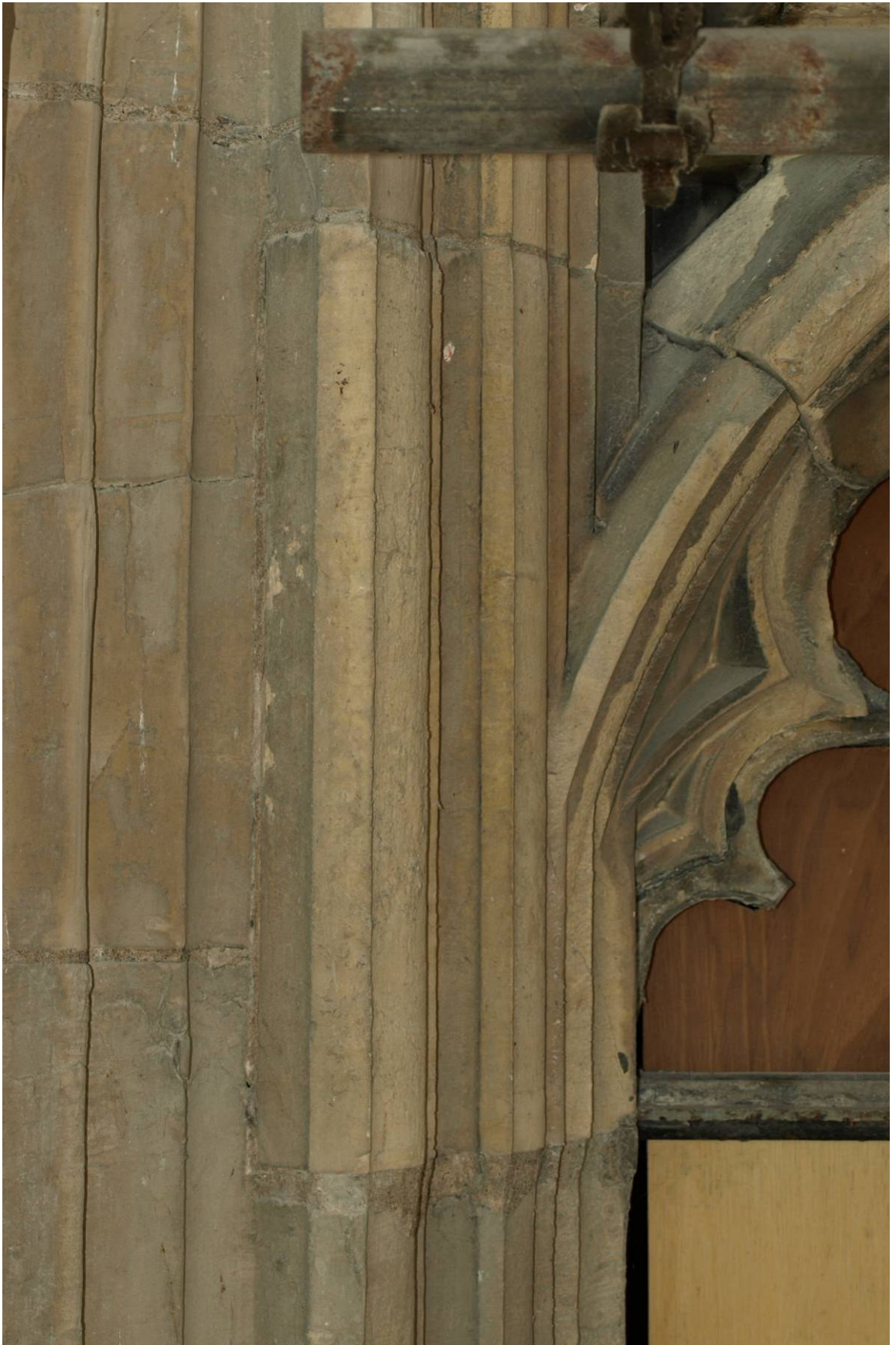
Figure 328: East Front, Great East Window exterior, detail showing relationship between upper transom and jamb, south side
