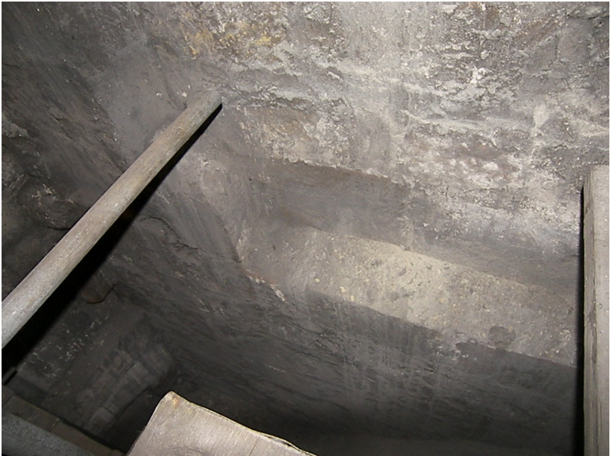
Figure 239: Thoresby's east end, south-aisle roof space looking to rear of East Front and off-setting in aisle wall
