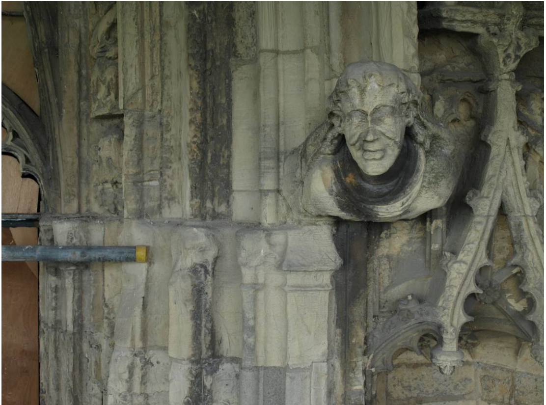
Figure 94: Great East Window exterior, north side of arch at springing level showing moulding change
