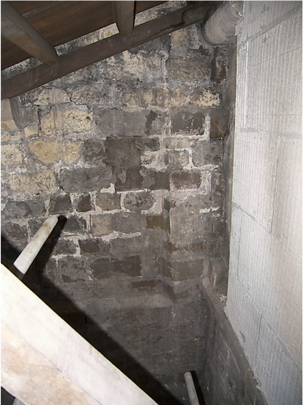
Figure 238: Thoresby's east end, north-aisle roof space looking to rear of East Front and tothing joint within angle between aisle wall and triforium
