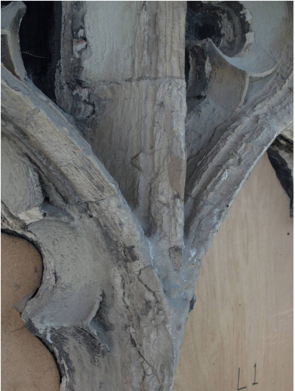
Figure 308: East Front, Great East Window exterior, medieval tracery detail showing typical weathering patterns, surface repairs and protective coatings
