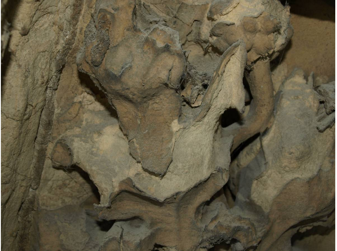
Figure 431: Great East Window, exterior voussoirs, detail of decay
