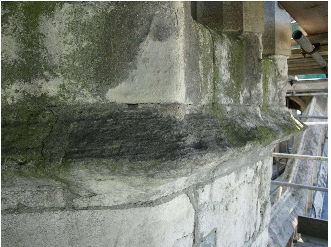
Figure 288: East Front, west face of north buttress showing introduced stooling beneath corona
