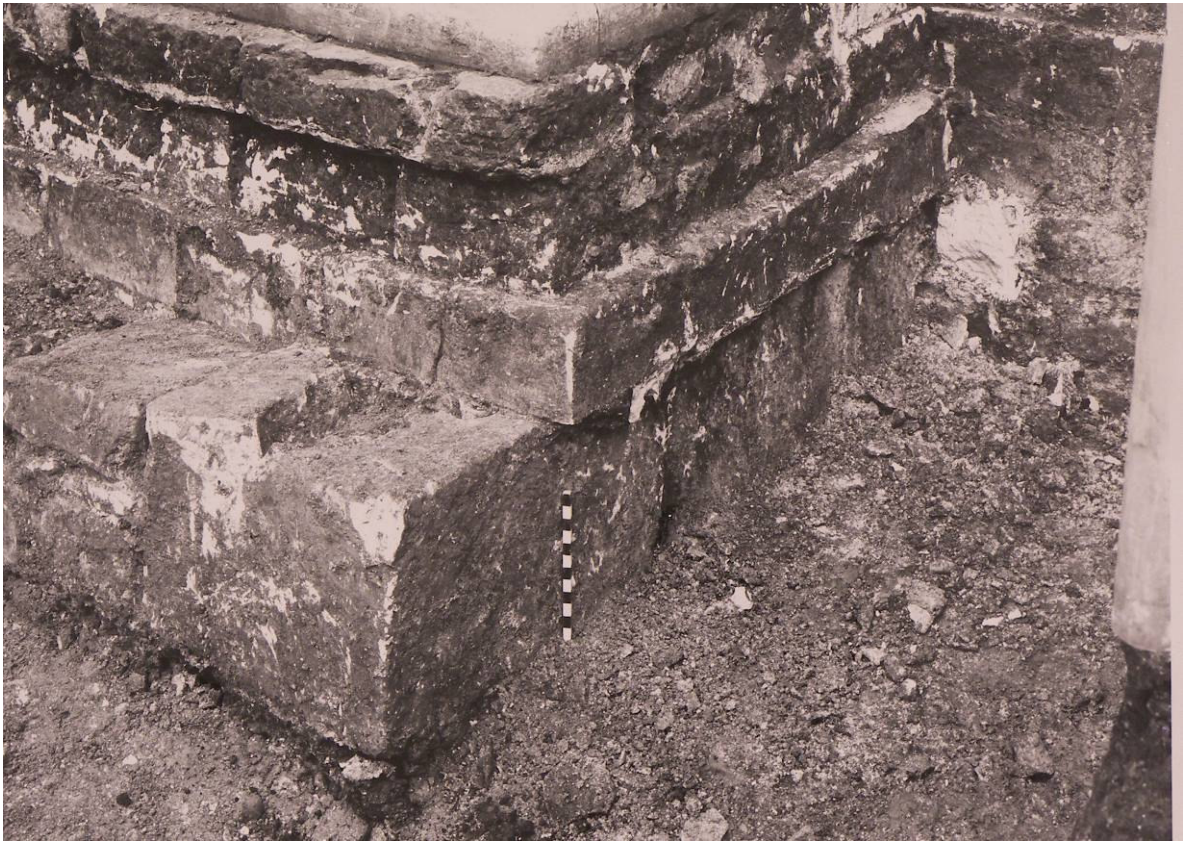
Figure 156: Outside east end, foundations of first buttress west of north-east corner of East Front looking south-east, 1969 (YML/YMEX/6479)
