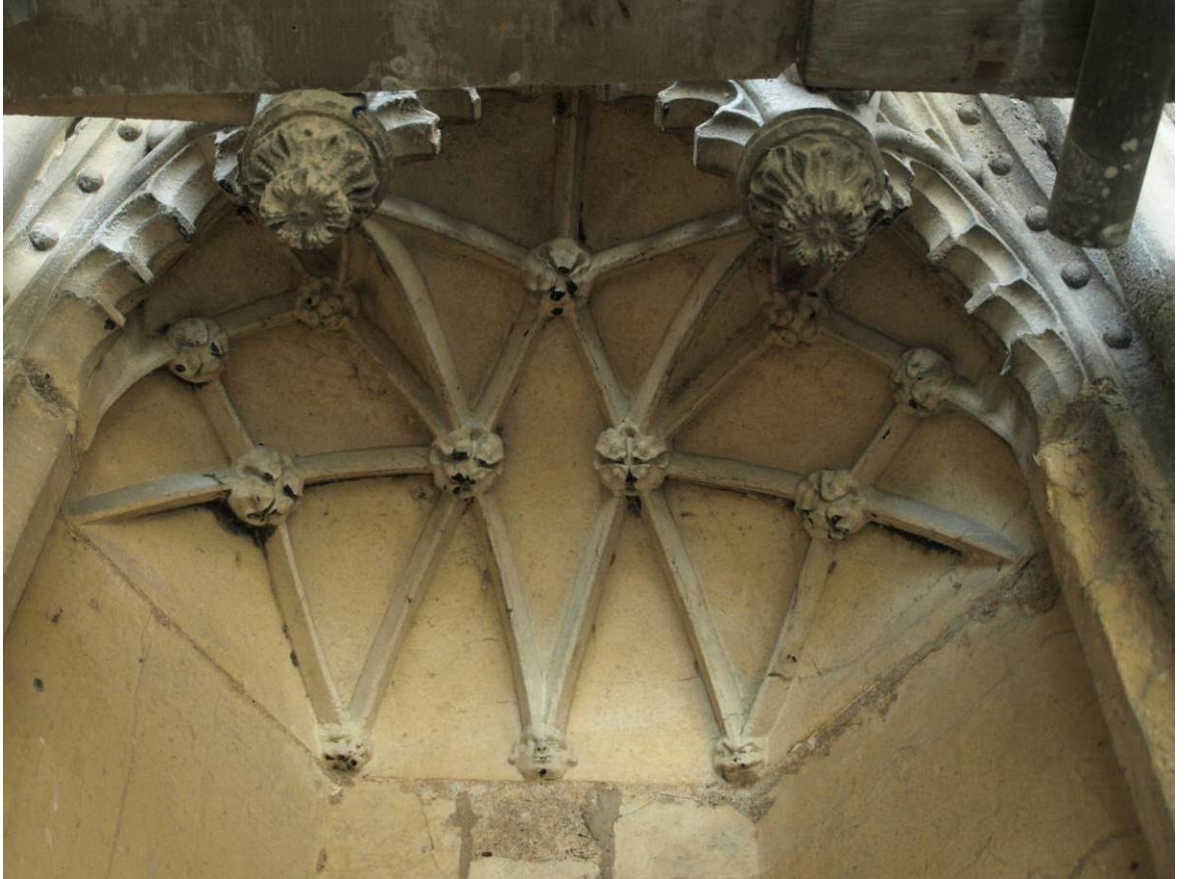
Figure 198: East Front, detail of canopy above niche to south of Great East Window, Level A
