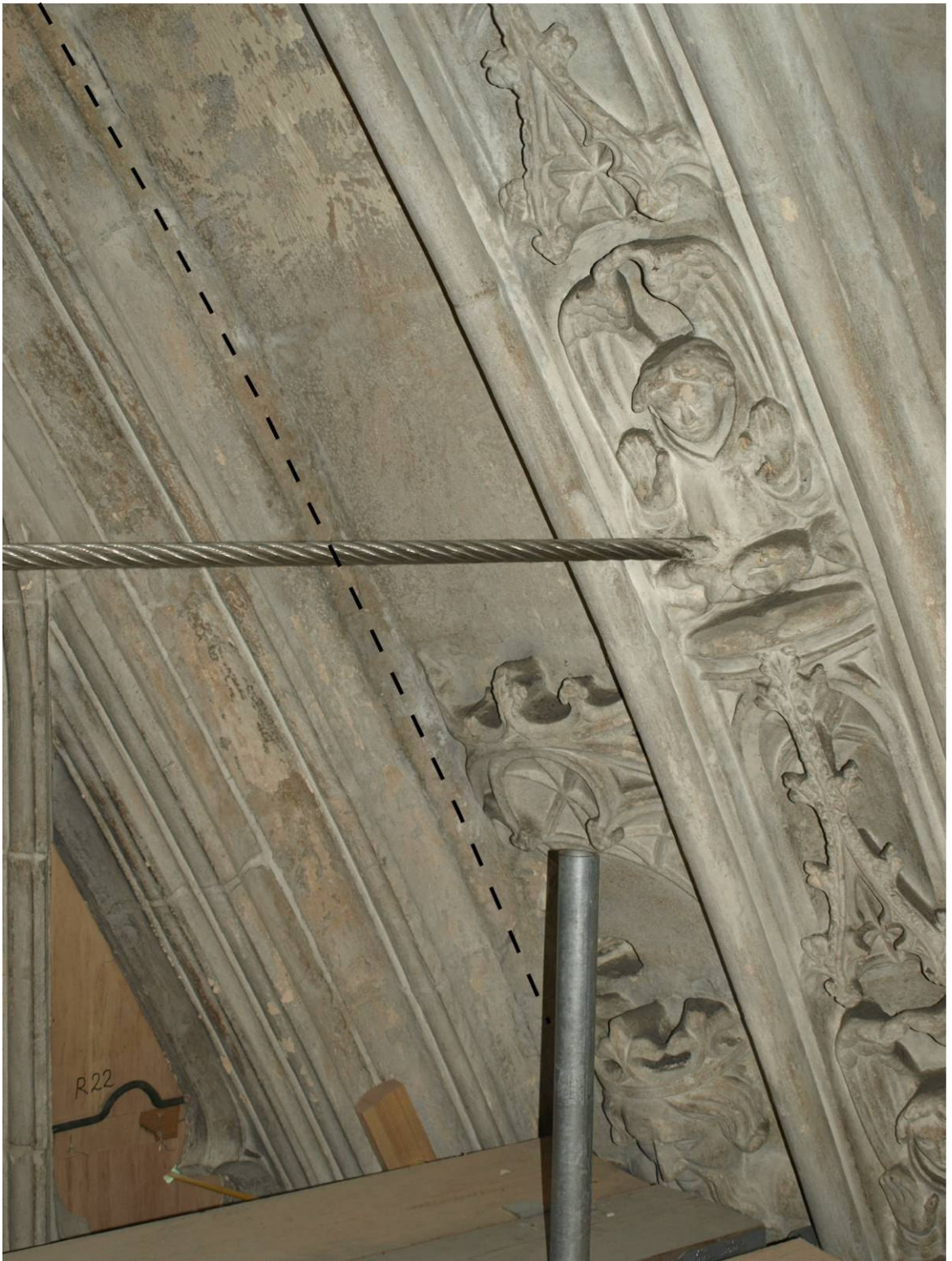
Figure 338: Great East Window interior, south side of arch showing relationship between interior and exterior masonry; dashed line marks mortar infill
