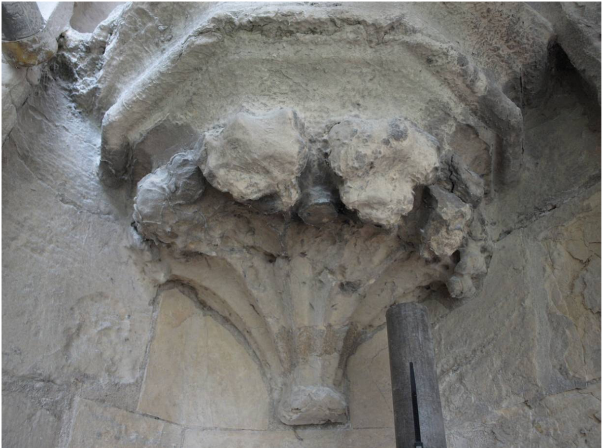
Figure 270: East Front, fourteenth-century niche-pedestal with later repairs, south side of Great East Window, Level D
