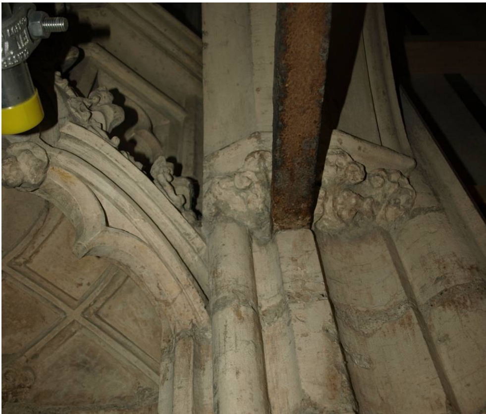
Figure 330: Great East Window interior, detail showing relationship between inner screenwork and iron reinforcement and window aperture, lower transom south side
