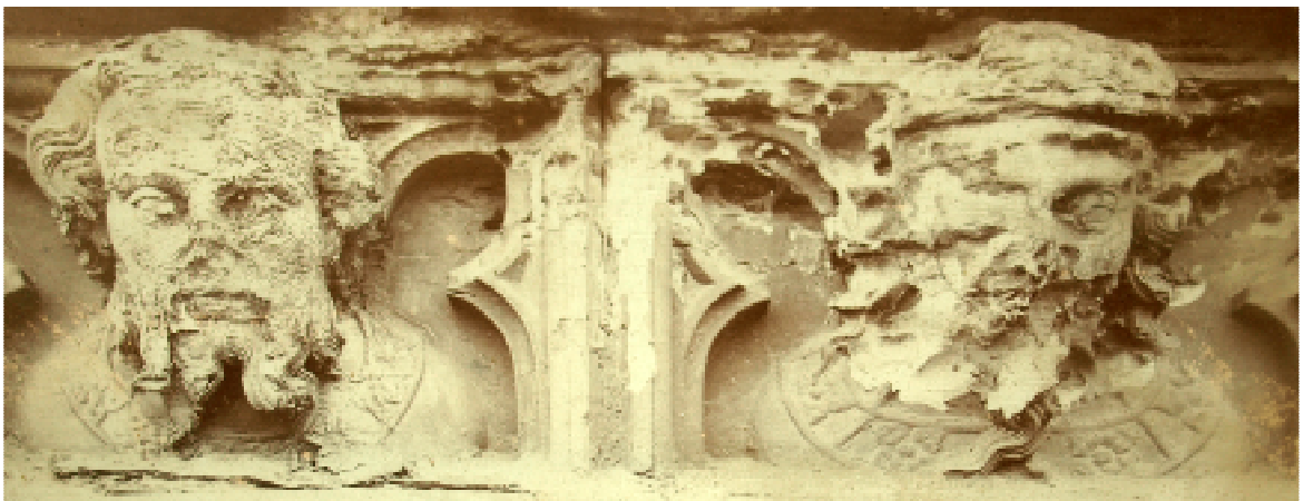
Figure 59: Sill carvings beneath Great East Window before renewals, Nos. 11-12 (YM Stoneyard)
