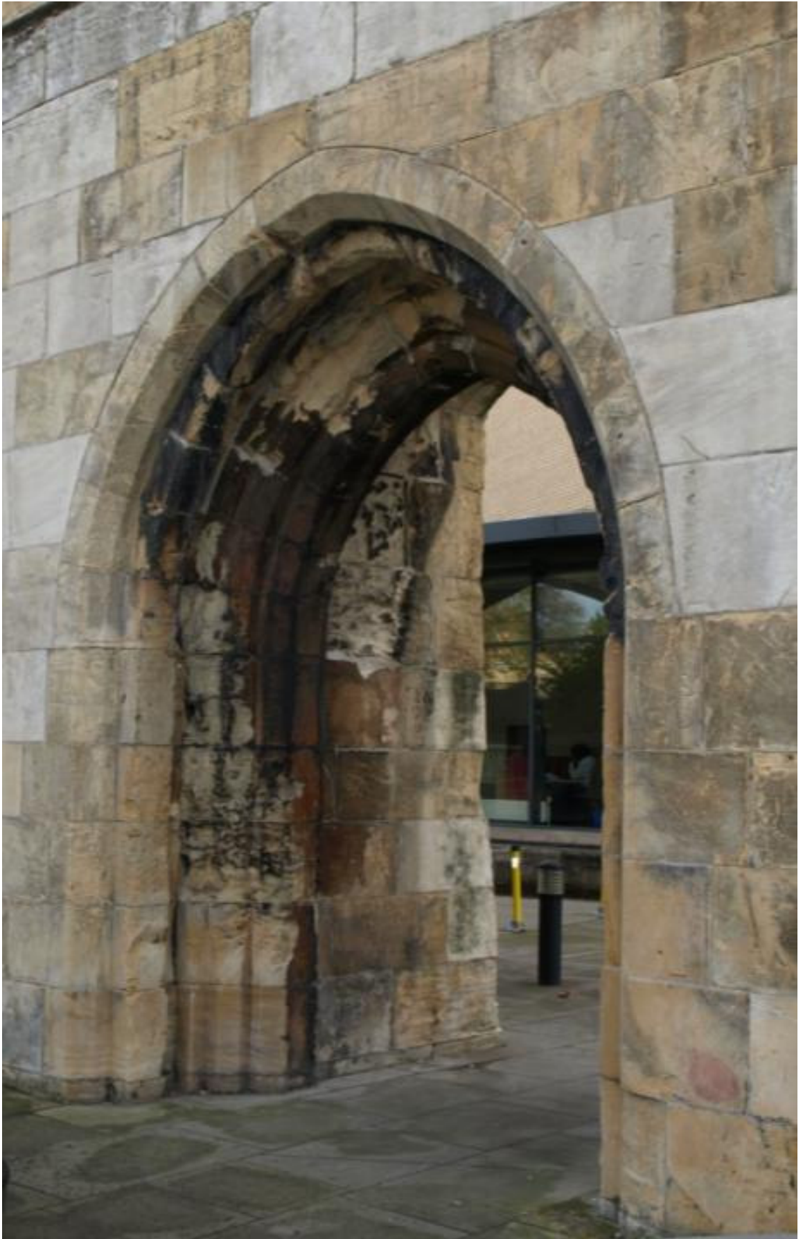
Figure 5: Example of sheltered decay of magnesian limestone, the City Walls, York
