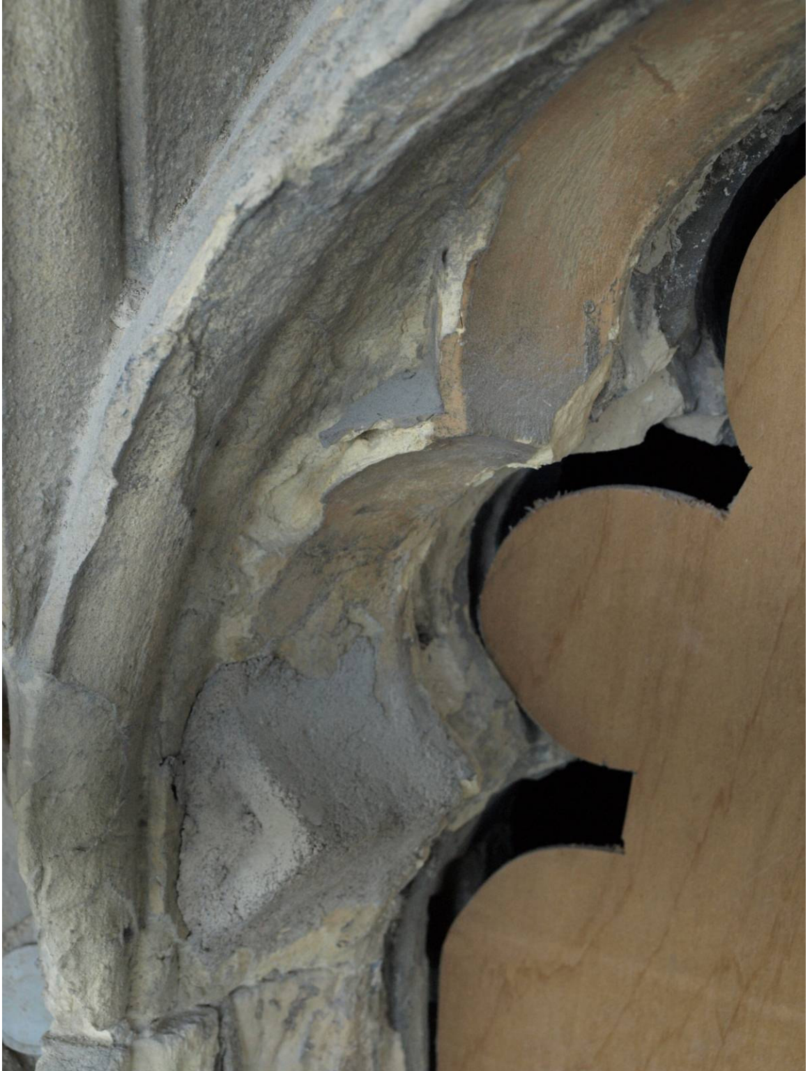
Figure 321: East Front, Great East Window exterior, detail of previous surface repairs and coatings
