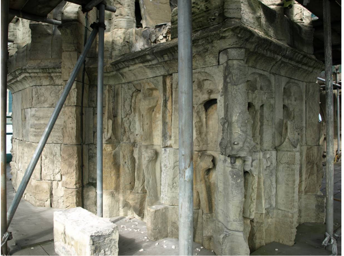
Figure 292: East Front, upper section of south buttress before repair, Level F (south-east faces)
