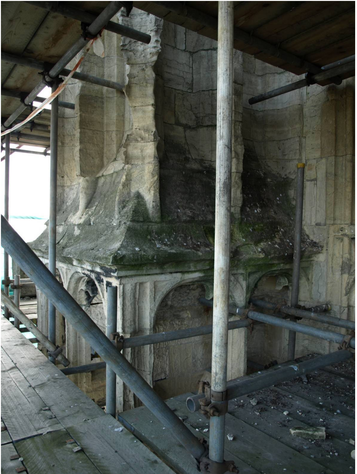
Figure 299: East Front, south buttress before repair, Levels E-F, north-east side
