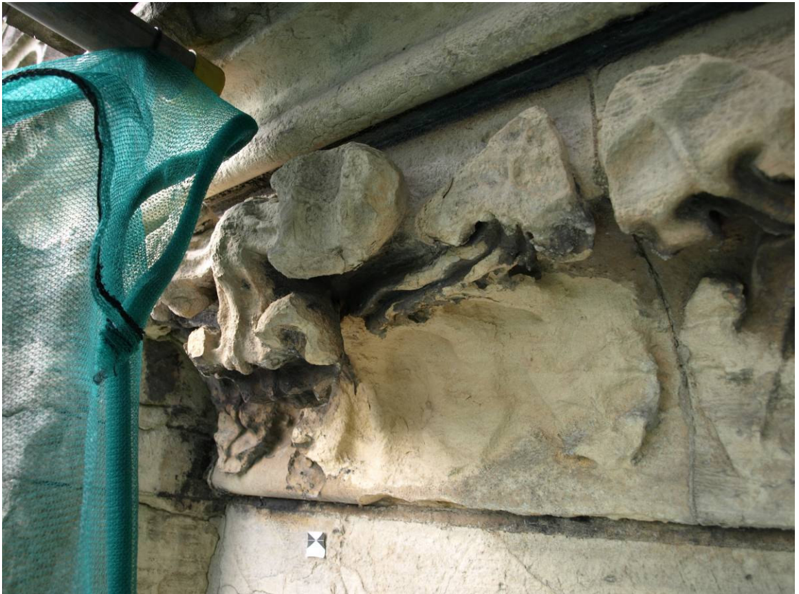
Figure 432: South-clerestory cornice, example of cavitation upon stones previously treated with linseed oil
