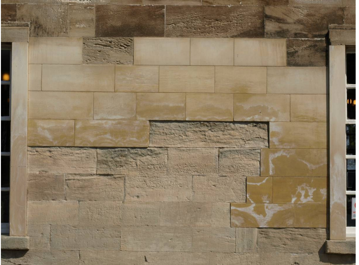
Figure 439: Cusworth Hall, South Yorkshire. Detail of salt damage to new magnesian-limestone masonry
