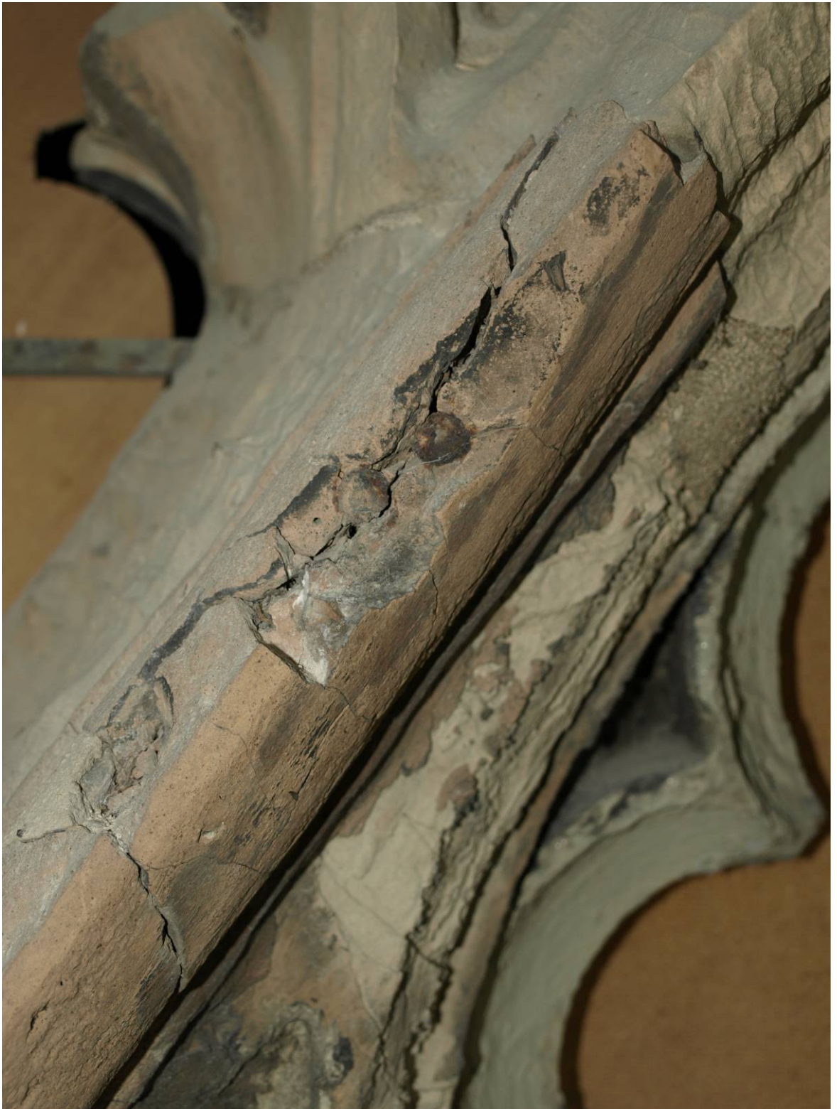
Figure 322: East Front, Great East Window exterior, detail showing Roman Cement repair reinforced with iron nails
