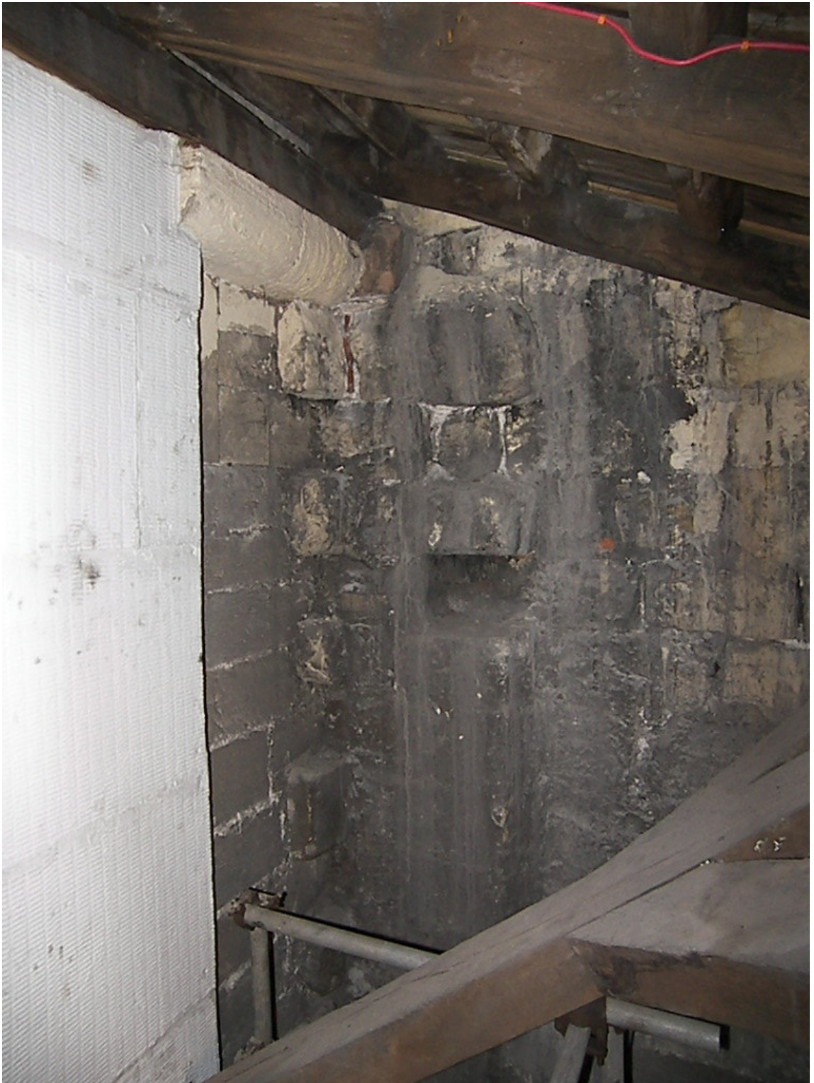
Figure 237: Thoresby's east end, south-aisle roof space looking to rear of East Front and tothing joint within angle between aisle wall and triforium
