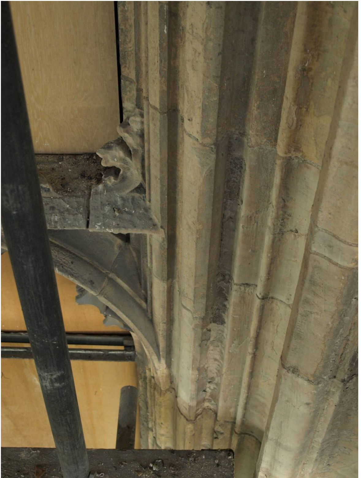
Figure 327: East Front, Great East Window exterior, detail showing relationship between lower transom and jambs, north side
