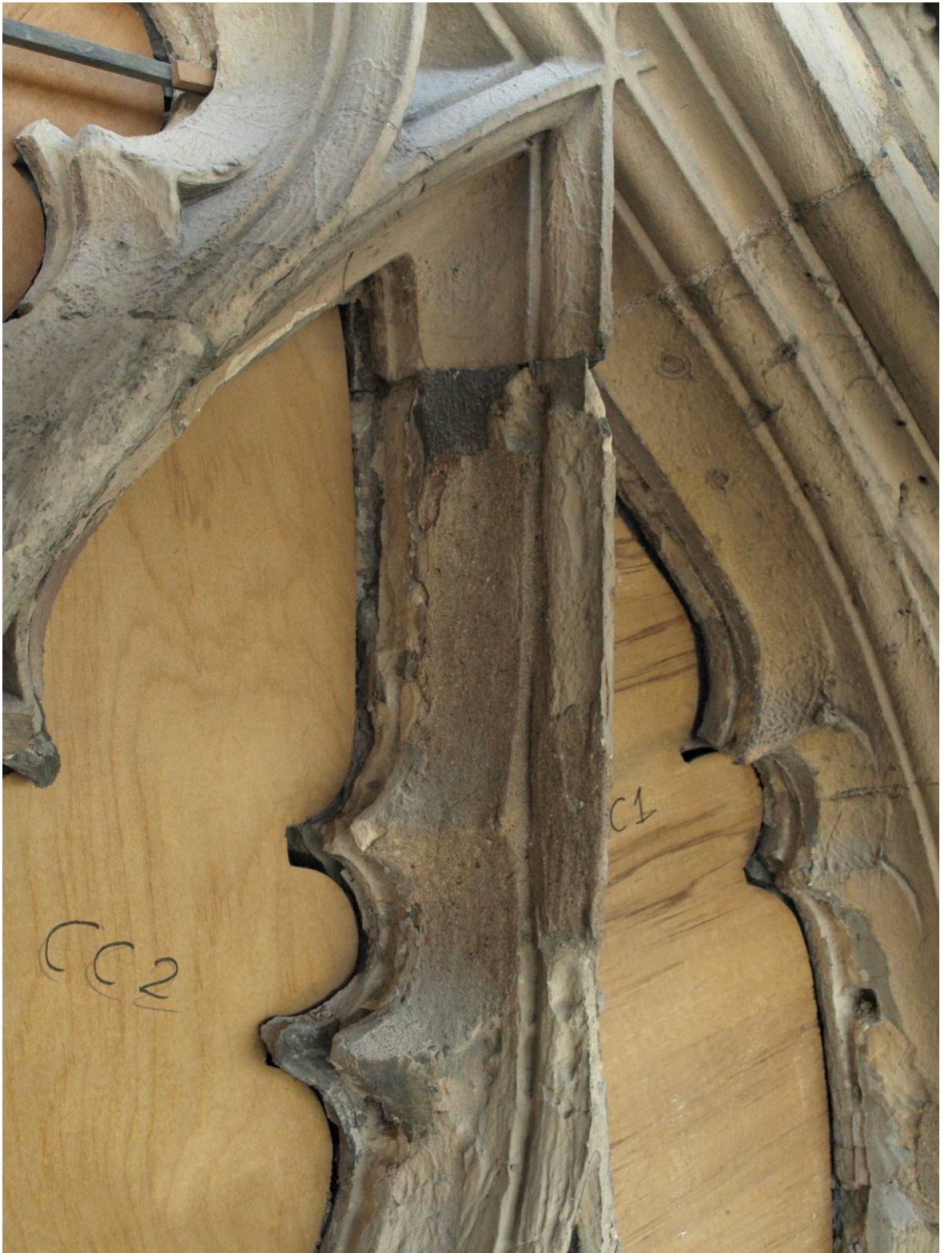
Figure 320: East Front, Great East Window exterior, detail of previous lime-based repairs
