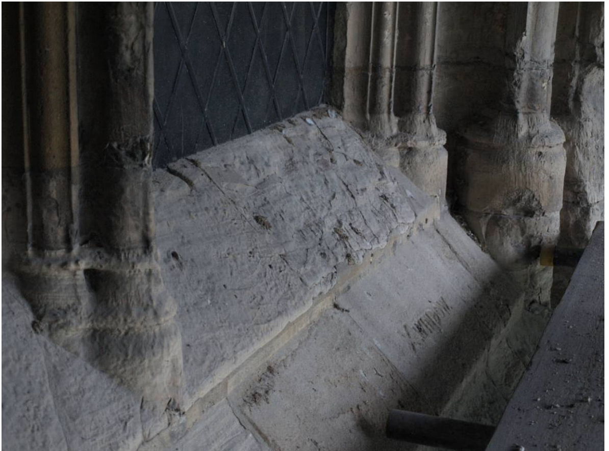
Figure 172: East Front, east window of south aisle, stonework and sill detail, Level A
