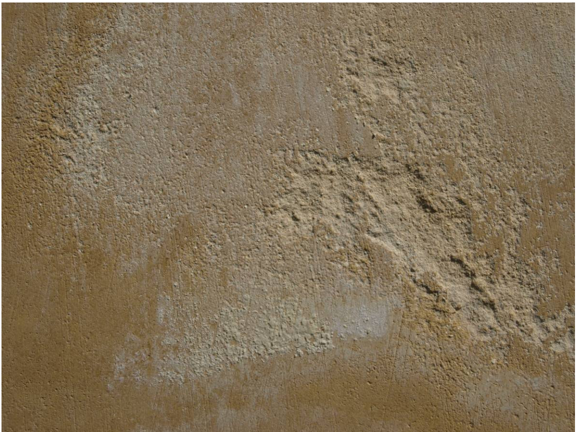
Figure 440: Cusworth Hall, detail of surface decay to new magnesian-limestone masonry
