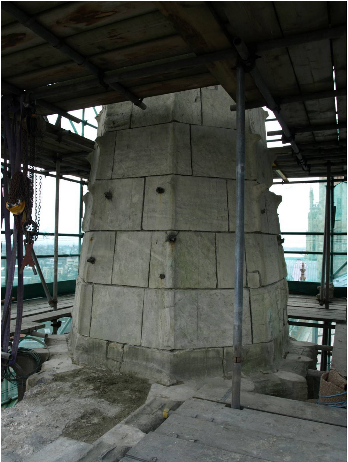
Figure 282: East Front, Levels H and I of south buttress during dismantling showing eighteenth-century spirelet upon medieval broach stones
