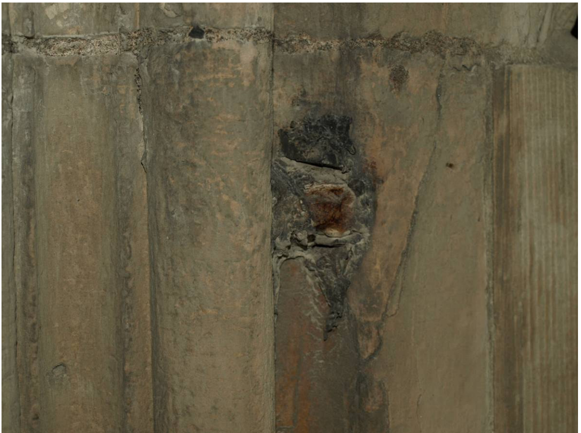
Figure 195: East Front, detail of metal fixing for statuary in right-hand jamb of niche in south-east turret, Level A
