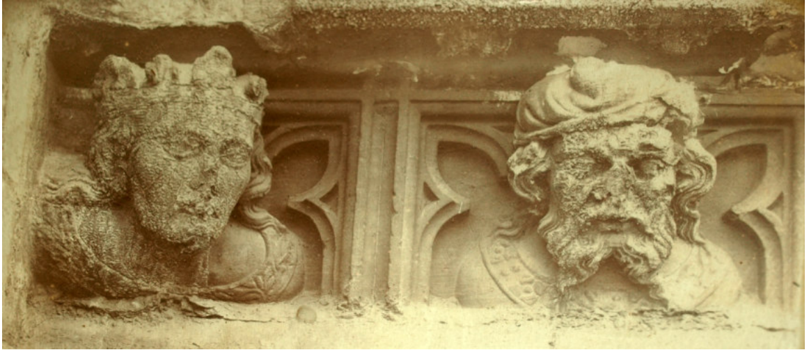
Figure 54: Sill carvings beneath Great East Window before renewals, Nos. 1-2 (YM Stoneyard)
