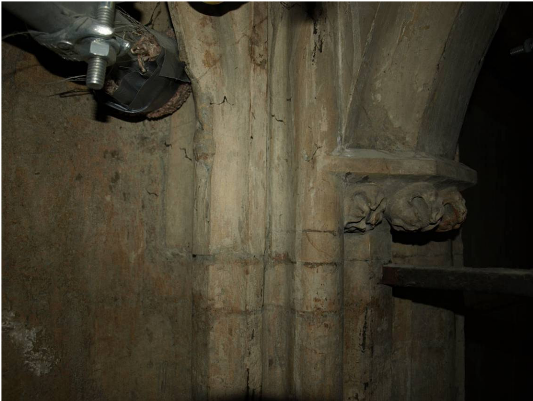
Figure 331: Great East Window interior, detail showing relationship between inner screenwork and iron reinforcement and window aperture, upper transom/walkway north side (screenwork masonry is 1820s work)
