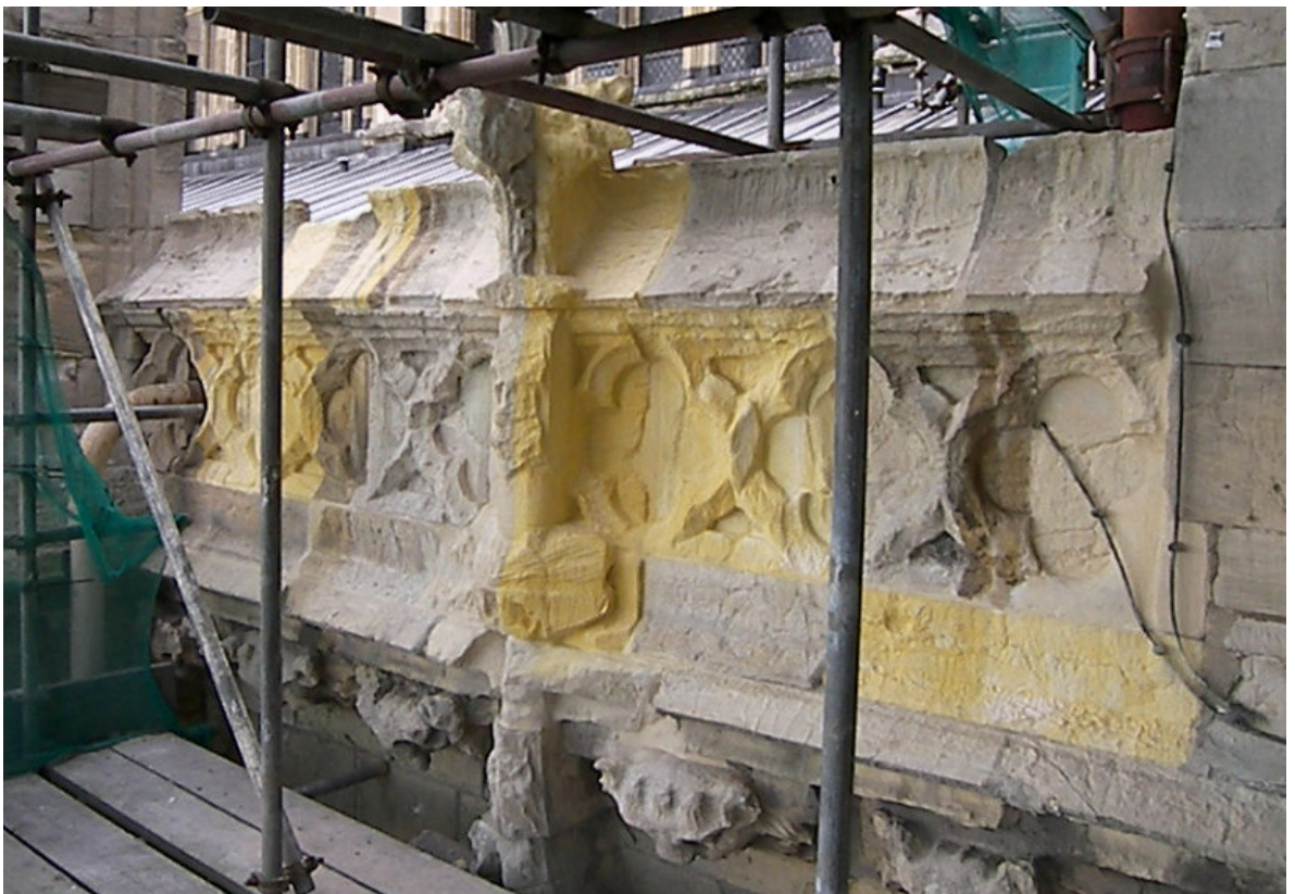
Figure 454: York Minster, south-aisle parapet, easternmost bay after mortar consolidation and application of surface treatments, July 2007
