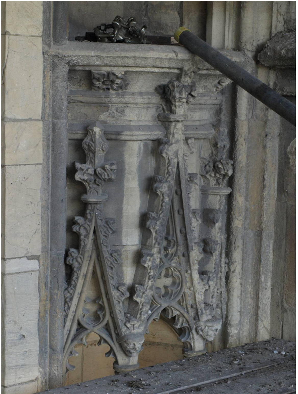
Figure 200: East Front, canopy above niche to north of Great East Window, Level A
