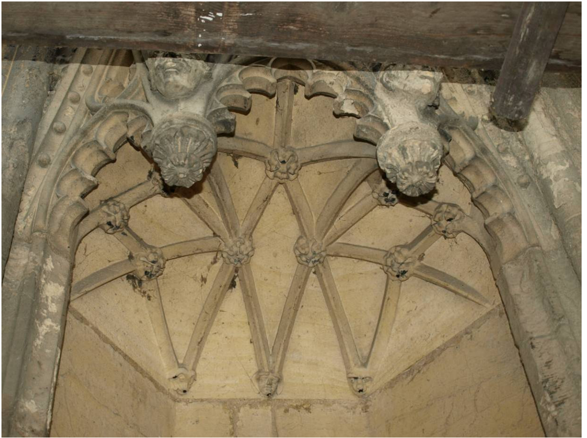
Figure 201: East Front, canopy above niche to north of Great East Window, Level A
