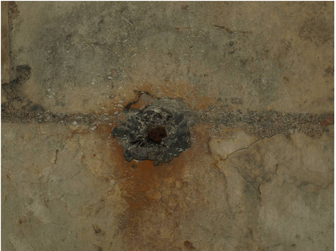
Figure 194: East Front, detail of metal fixing for statuary in rear of niche in south-east turret, Level A
