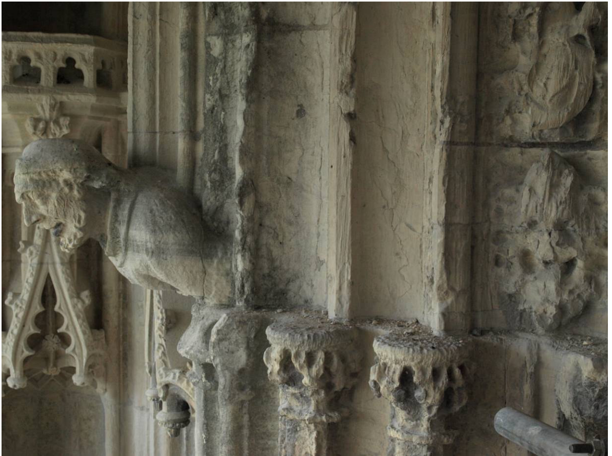
Figure 93: Great East Window exterior, south side of arch at springing level showing moulding change
