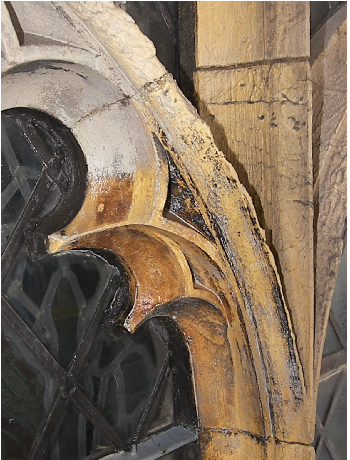
Figure 437: Great East Window, exterior mullions and transom masonry after cleaning trials. Note removal of 1960s paint but retention of historic patination
