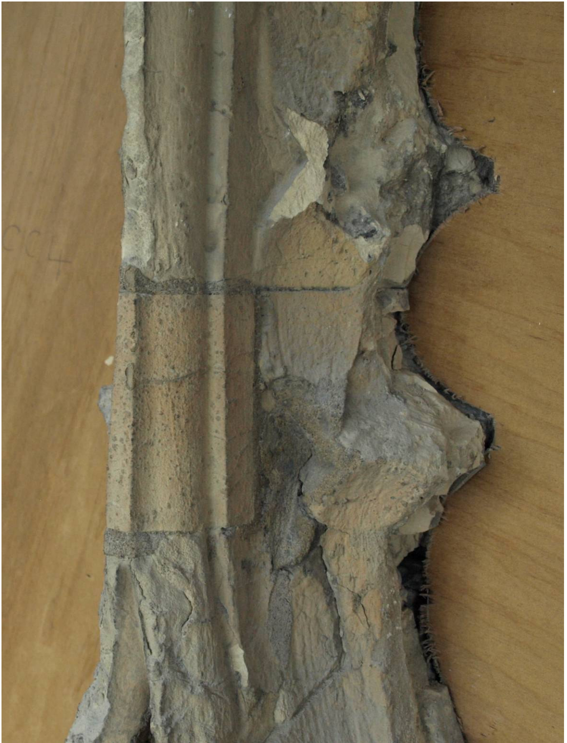
Figure 309: Great East Window exterior, tracery detail showing 1820s shallow indent
