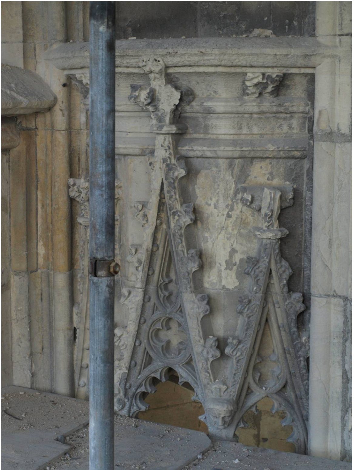
Figure 197: East Front, canopy above niche to south of Great East Window, Level A
