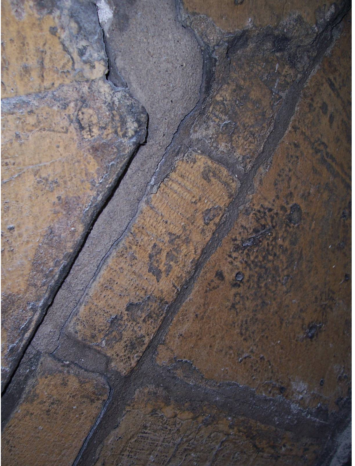
Figure 253: Thoresby's east end, easternmost bay, ?medieval infill to separated masonry with later 1950s cement patching
