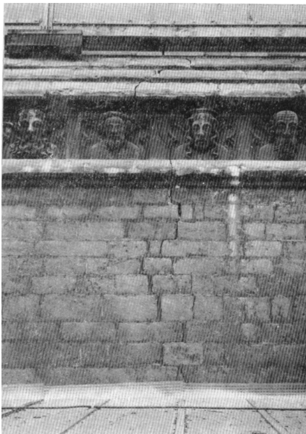
Figure 85: Sill carvings beneath Great East Window showing dark sulphation and structural cracking (Feilden 1976, 89)
