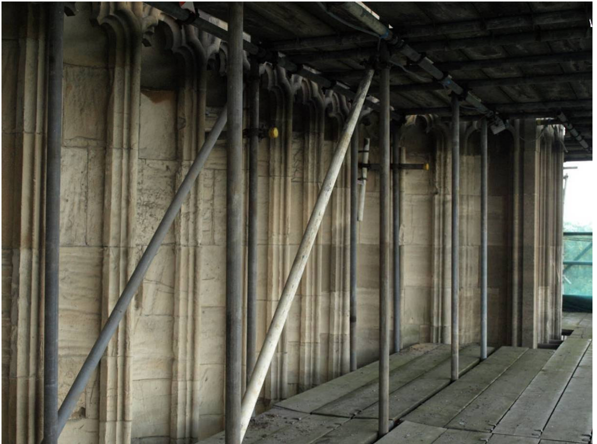
Figure 223: East Front, cusped niches in north-east turret and masonry above north aisle, Level C
