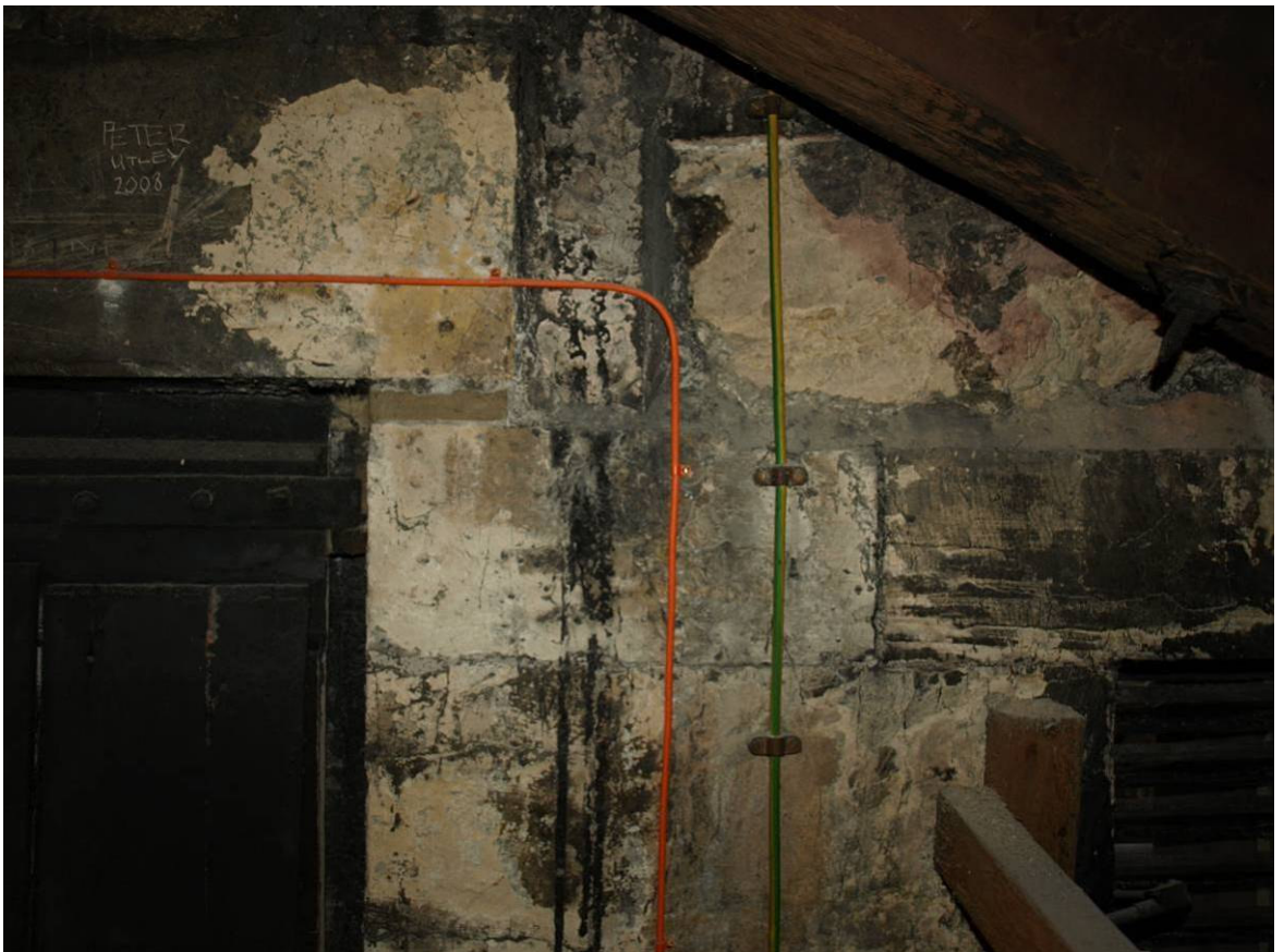
Figure 277: Roof space, Thoresby's east end; interior face of East Front illustrating fire damage adjacent to nineteenth-century replacement ashlar
