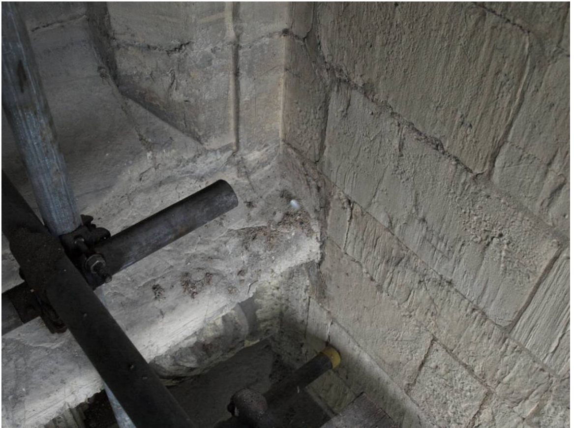
Figure 205: East Front, carved heads beneath sill of Great East Window showing bond between north carving and north buttress, Level A
