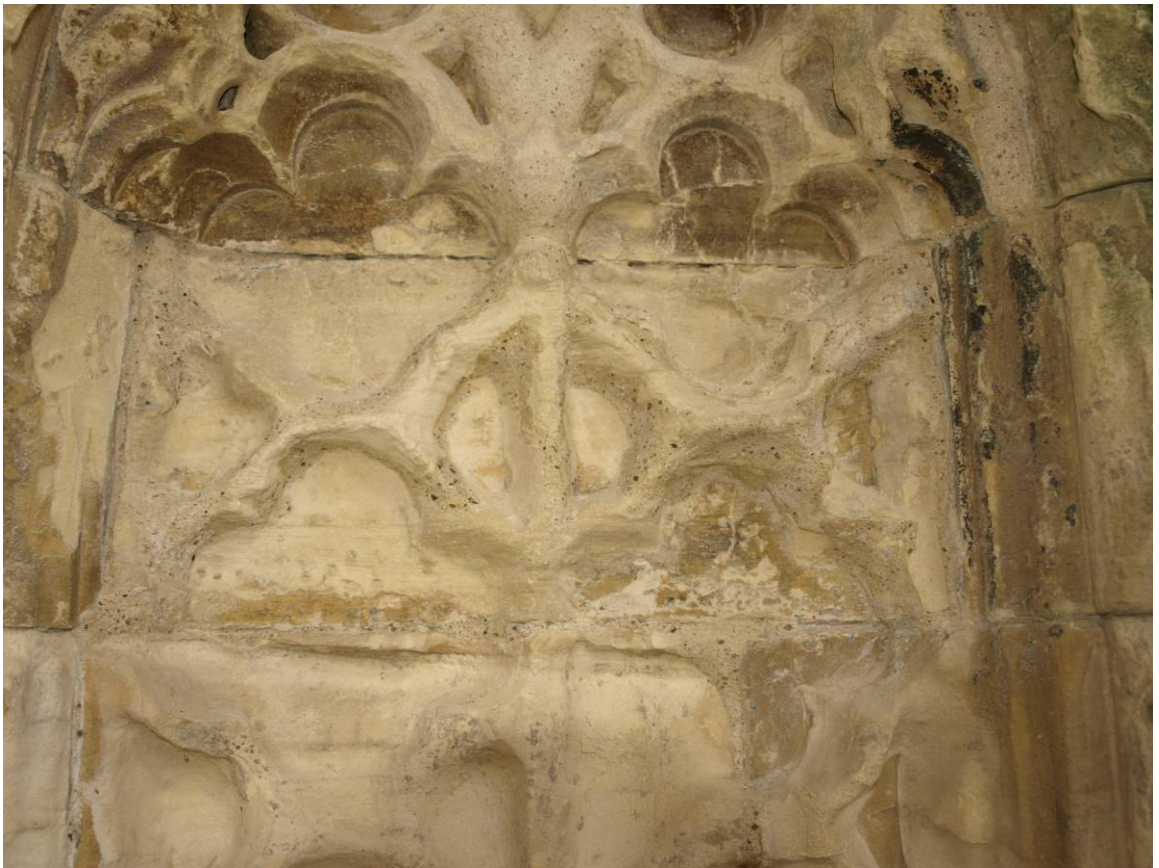
Figure 452: Howden Minster Chapter House, deteriorating NHL2 mortar repairs, June 2010
