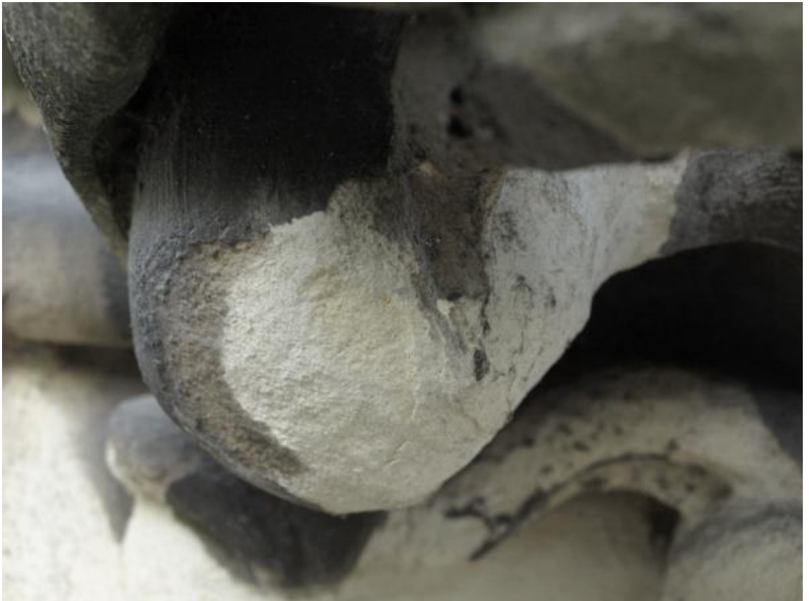
Figure 460: East Front, north-butress grotesque, detail of decay
