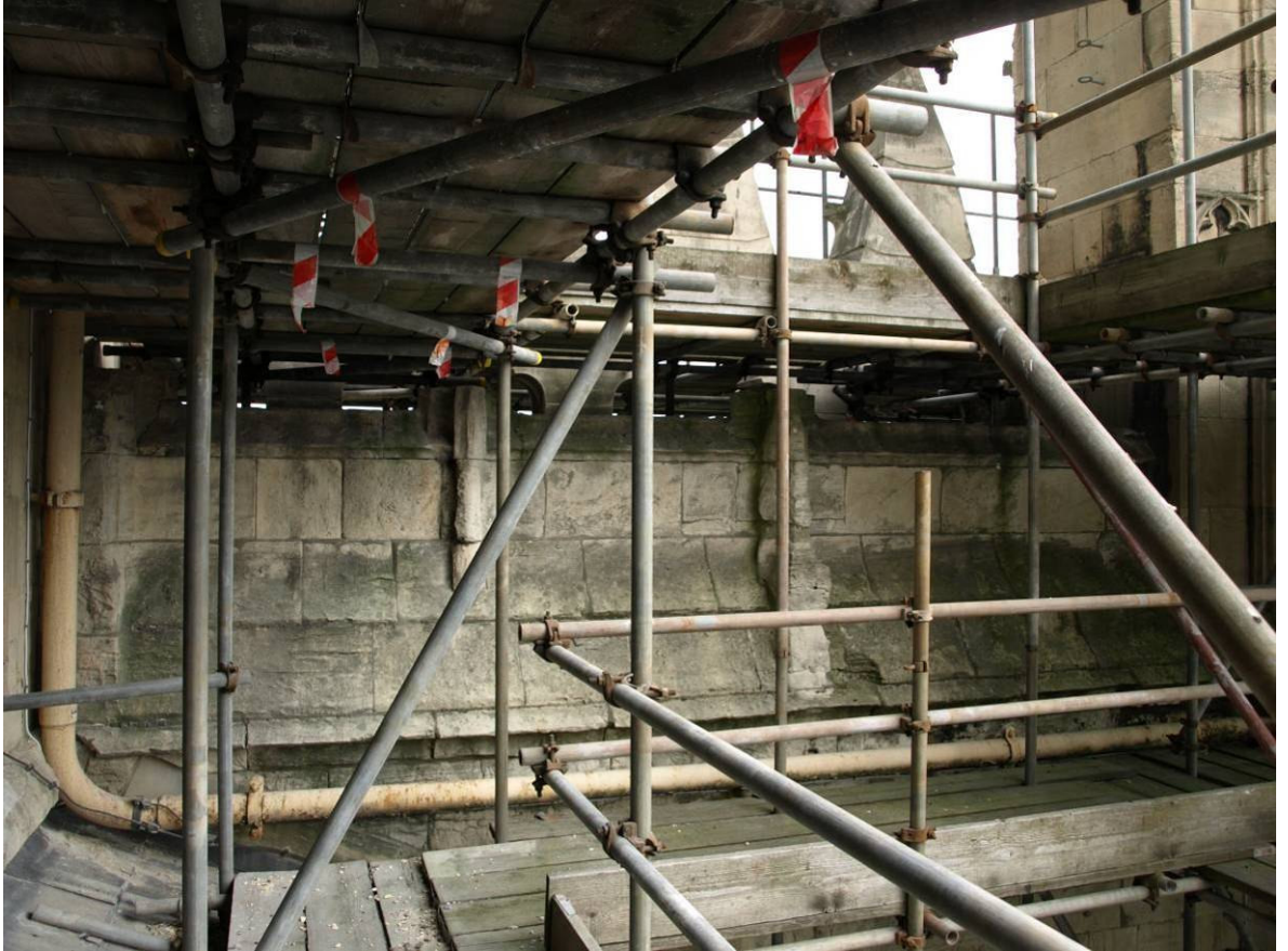
Figure 242: East Front above south-aisle roof, disused stoolings to rear of parapet, Level D
