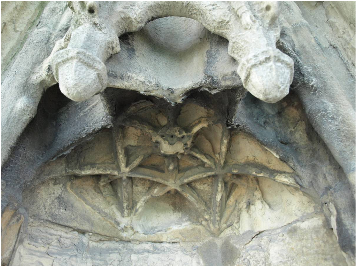
Figure 433: East Front, example of decay upon underside of canopy, north buttress
