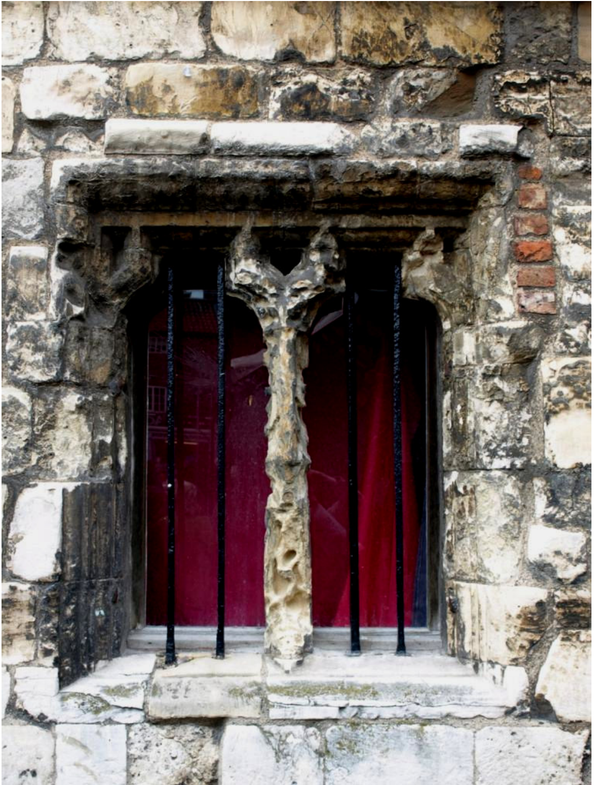
Figure 4: Example of advanced sheltered decay of magnesian limestone, Newmarket, York
