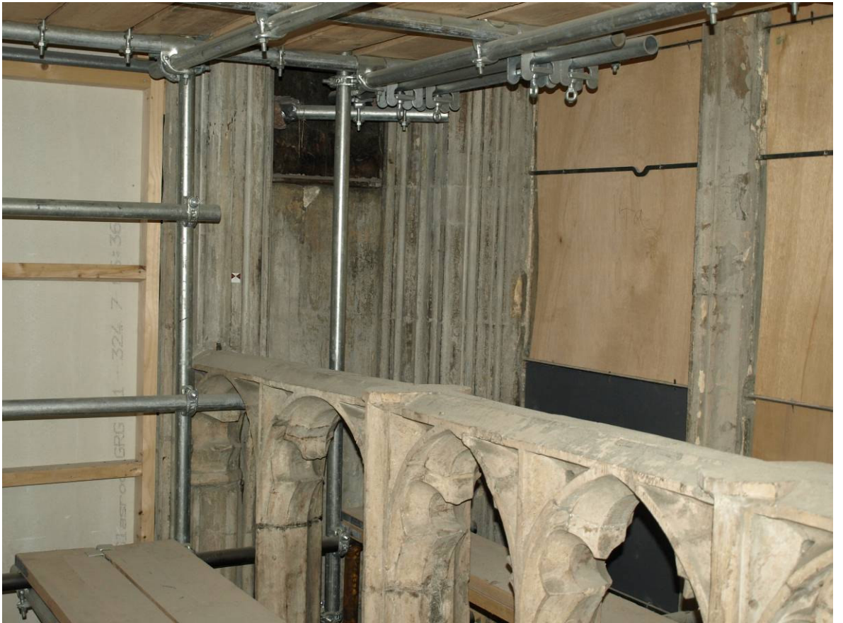
Figure 335: Great East Window interior, entrance to wall passage at springing level, north side
