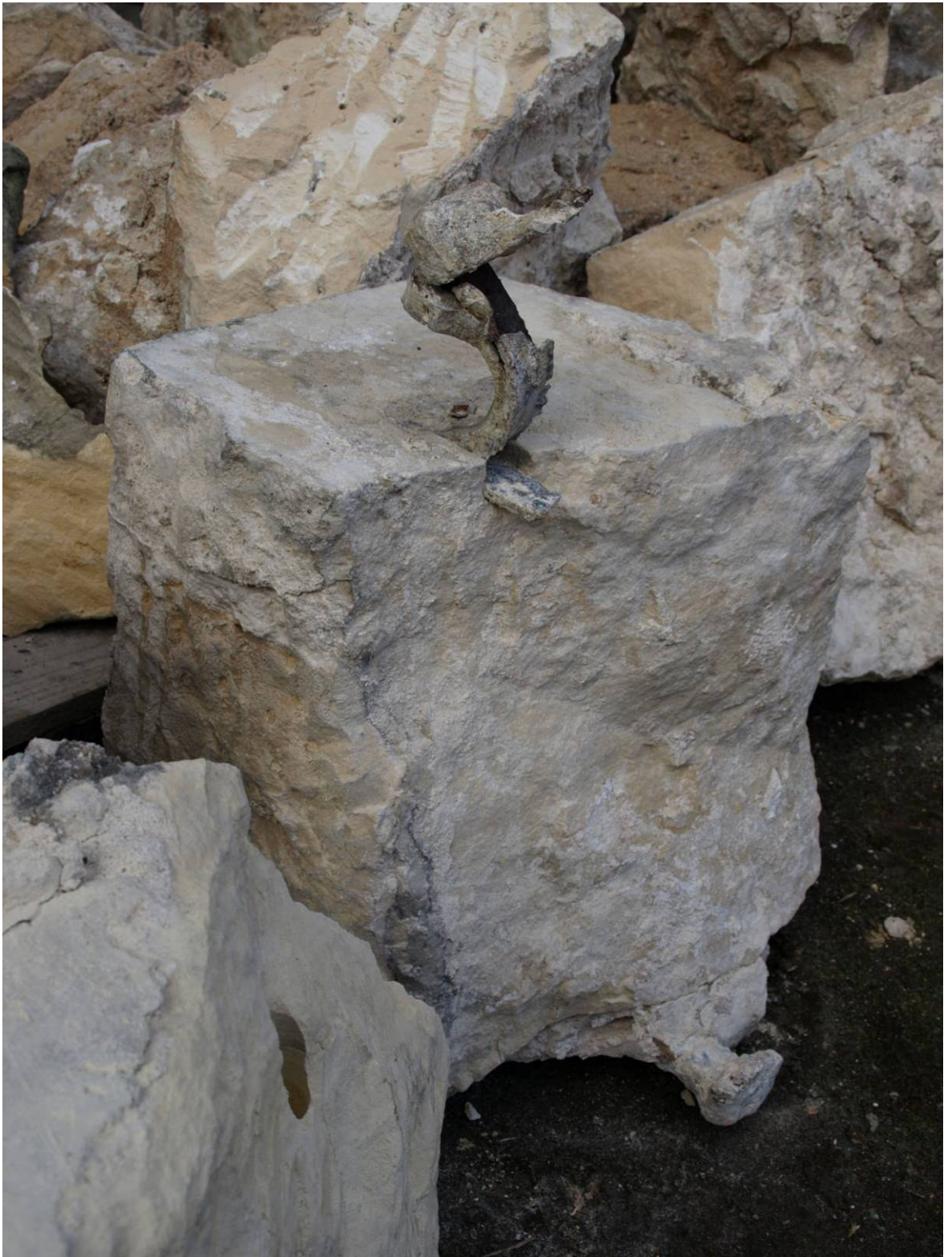
Figure 298: Removed medieval core-work from south-buttress Level F showing iron cramp used to secure later cladding
