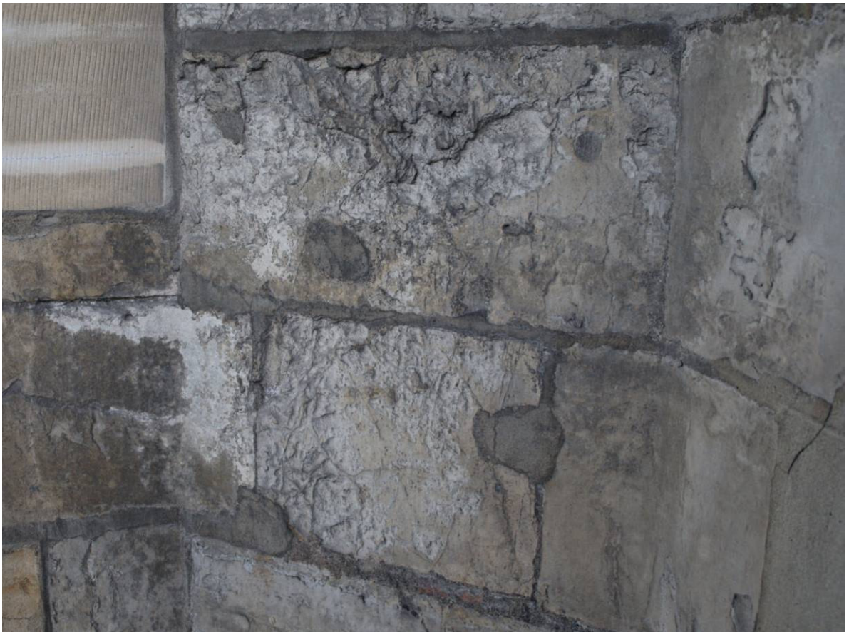
Figure 191: East Front, detail of holes for statuary fixings in niche in north-east turret, Level A
