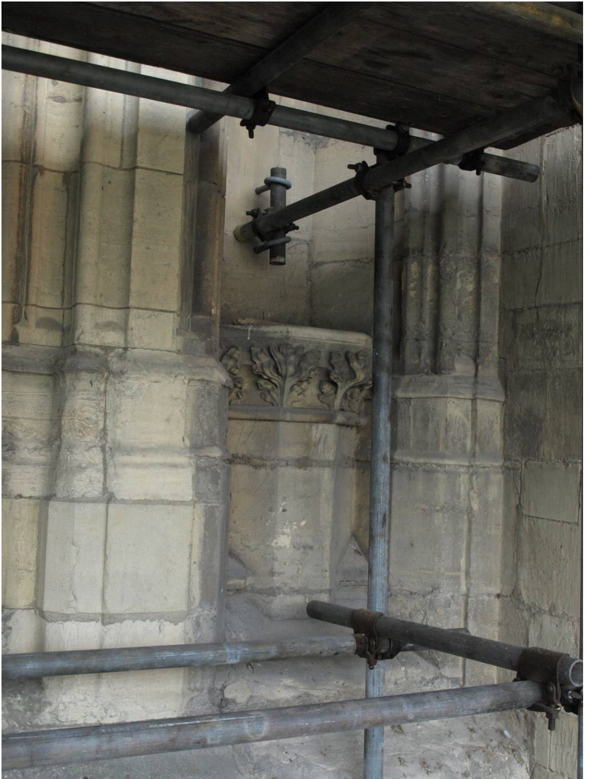
Figure 202: East Front, base of niche to north of Great East Window, Level A
