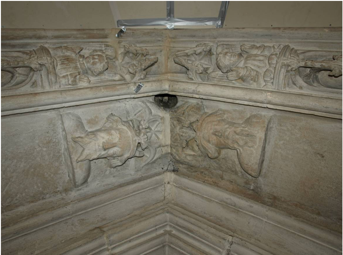
Figure 392: Great East Window interior, apex of arch showing truncated carvings
