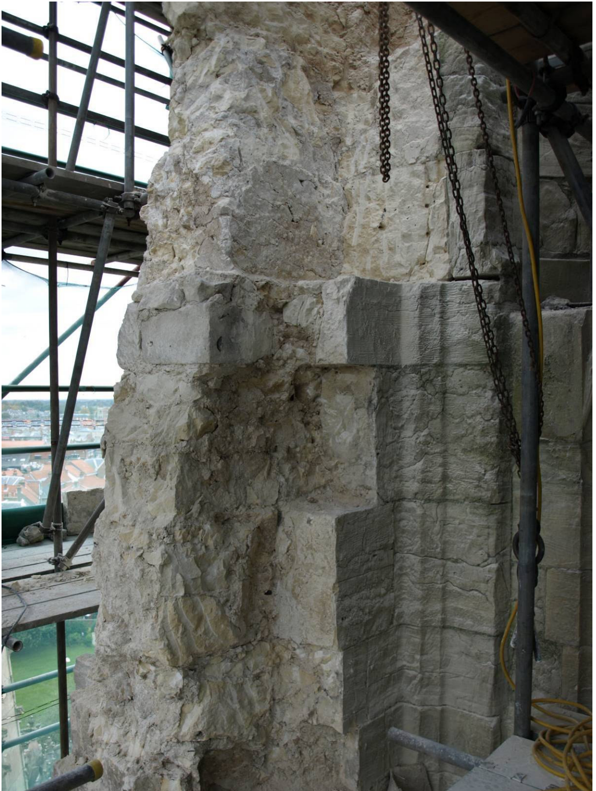
Figure 296: East Front, south buttress Level F during dismantling showing intact medieval core
