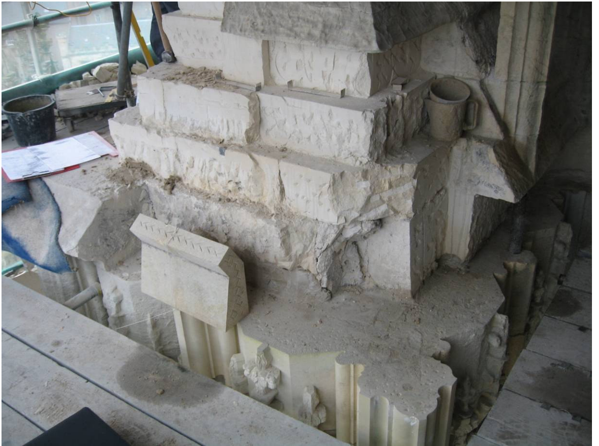
Figure 302: East Front, south buttress, Level E during repair (east and north faces) (Andrew Arrol)
