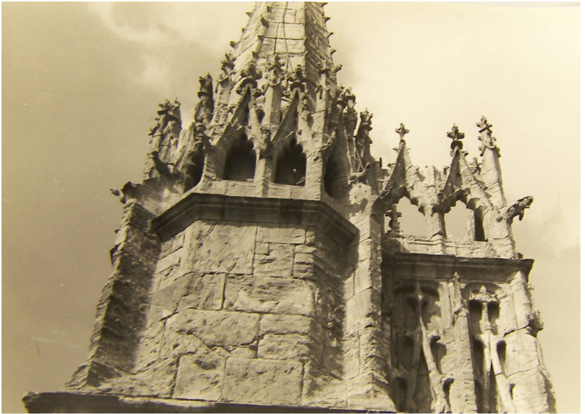
Figure 80: East Front, south buttress, turret and pinnacle from the south, 1950s (YML/APYM/A57iv)
