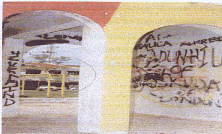
b. Vandalism in the form of graffiti.
