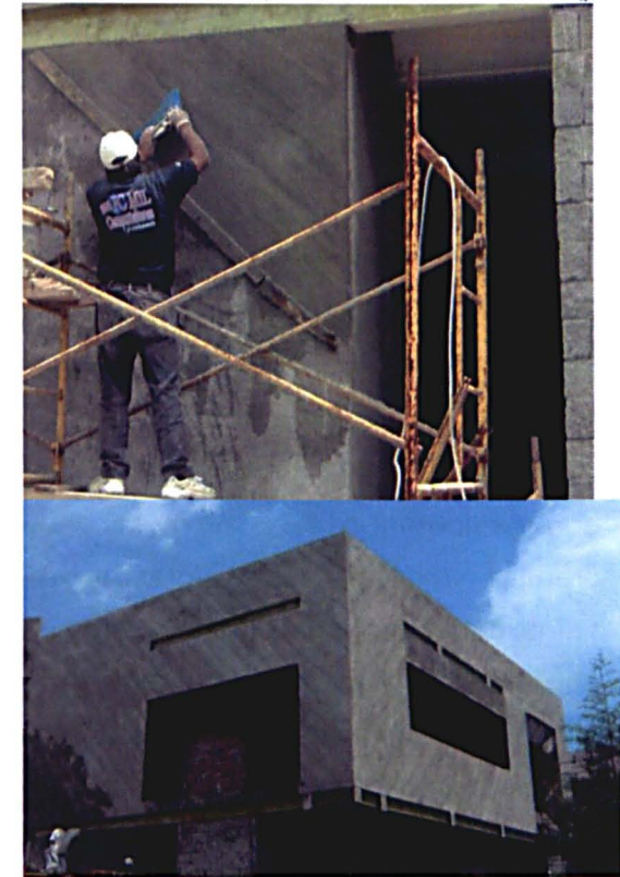
Fig. 1.5 & 1.6 Above: Master builder developing cement rendering with a top part of a brush over the facade of the future Institute of Chemical and Biological Research of the UMICH in Morelia, Mexico. This rendering technique is a very well known local technique. Bottom: Final impressions of the facade before painting.
