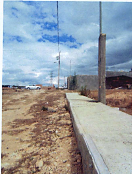
Street with a footpath and electricity post awaiting for paving and electricity supply.
