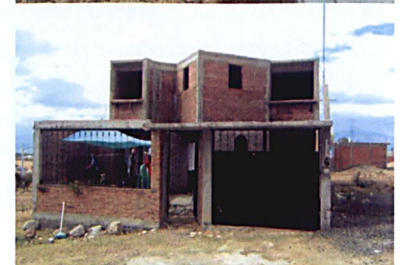
Figs. 2.11 Above: View of one street at Colonia Popular of El Durazno, Morelia, Mex. A footpath and electricity have been recently introduced. Additional services are planned to be introduced in the following 3 years.
