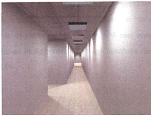
Set C1 (Image 21): Straight bearing 1.42m, reference corridor and left hand corridor 2m
