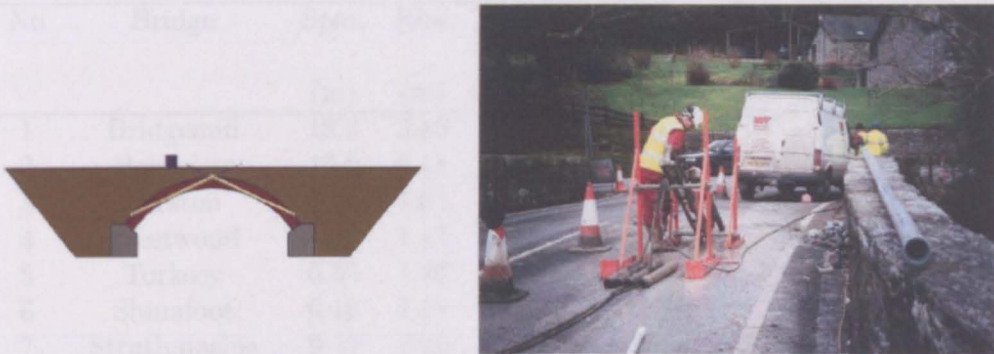
FIGURE 2.3: Typical anchor positions and installation of reinforcement from the road surface (Mabon 2002)
