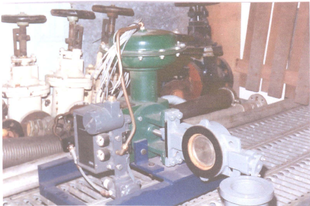
Plate 3.5: Example of a pneumatic control valve
