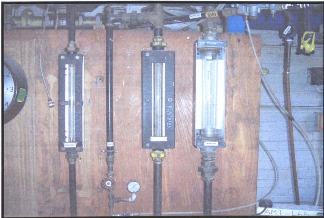
Plate 3 Gas and Air controller
