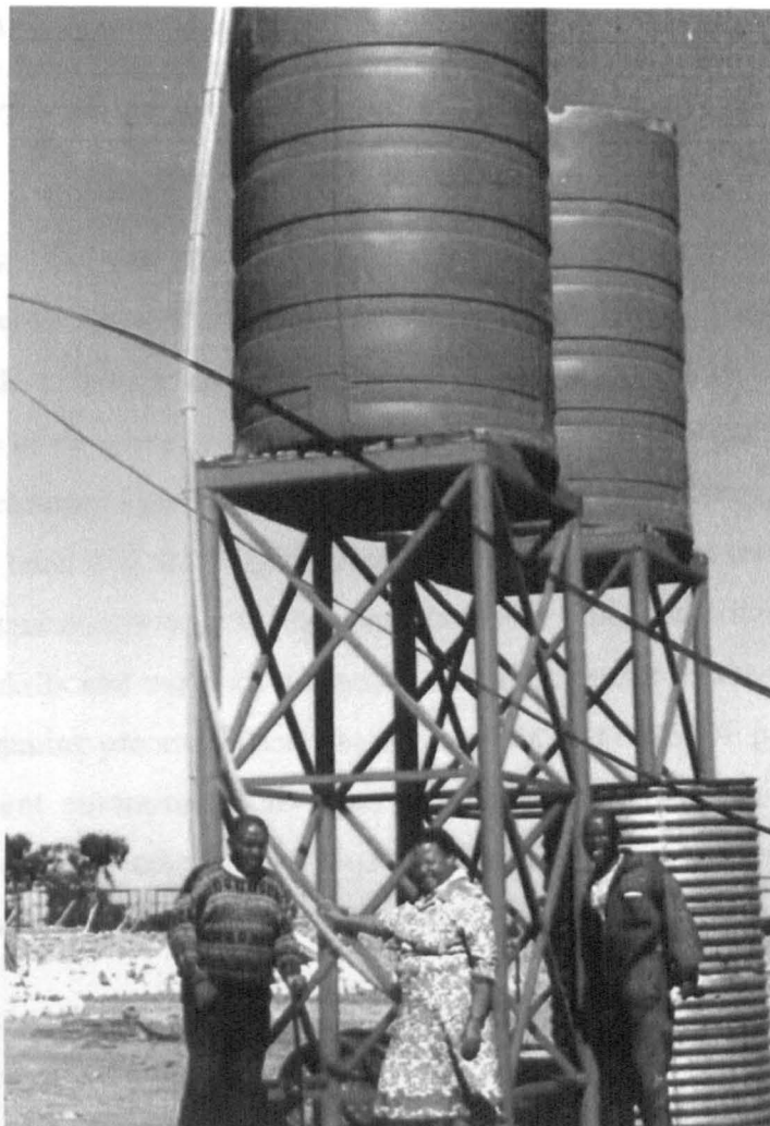
Water tanks installed as part of the new water supply system at Mogopa, 1995
