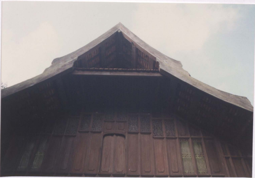
Figure 2.21: 'Pemeleh' at the roof edge of a traditional Malay timber palace in Terengganu.
