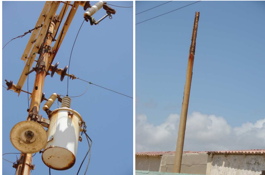
Figure: 4. Electricity line and equipment, next to Las Cumaraguas Salina
