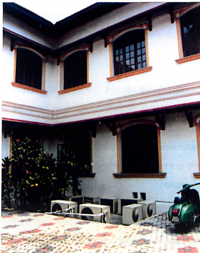
Fig.48 Placing air-conditioning units at outside is more preferable than on windows and walls
