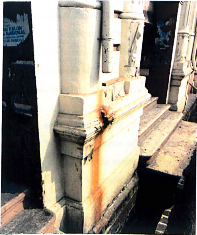
Fig.57 Common problems associated with defective rainwater goods
