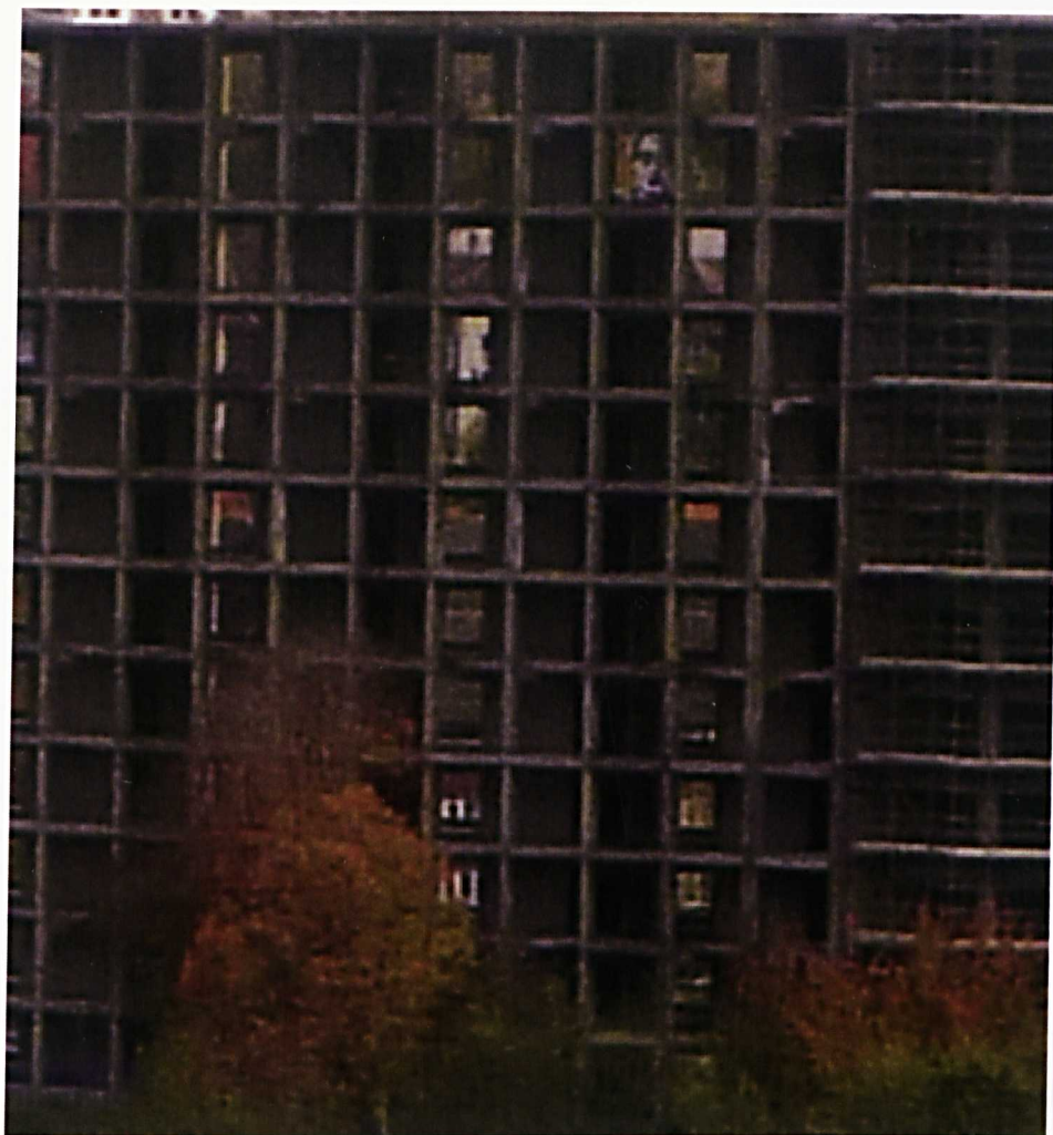
Photo taken from Hallam University building, looking through the retained concrete frame. Taken during strip-out works Oct 2009. (Source: author)
