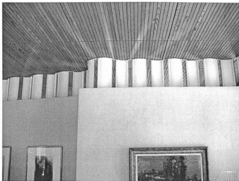
[Fig. 5-57] 'Shafts of light' at the glazed slots of the library wall
