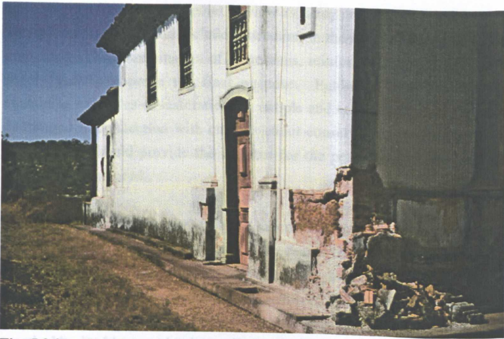
Fig. 5.3.21 - Church of Rosario (Santa Rita Durão, district of Mariana): the mortar and bricks used as part of the wall are coming loose at this corner.
