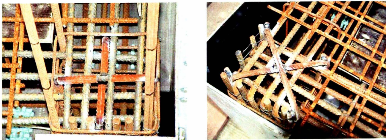
Figure 5.4. Detail of anchorage of column bars at the top of the storey joints (Chaudat, 2005).
