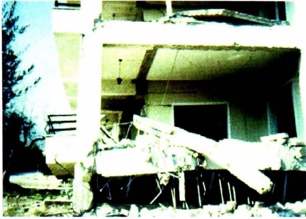
(a) Shear failure in joints
