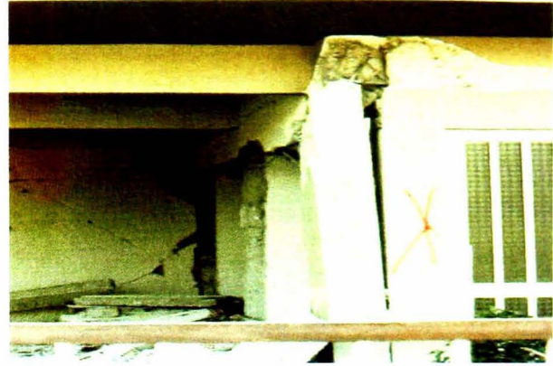
(b) Column bars debonding
