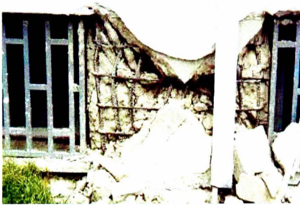
(c) Short column failure
