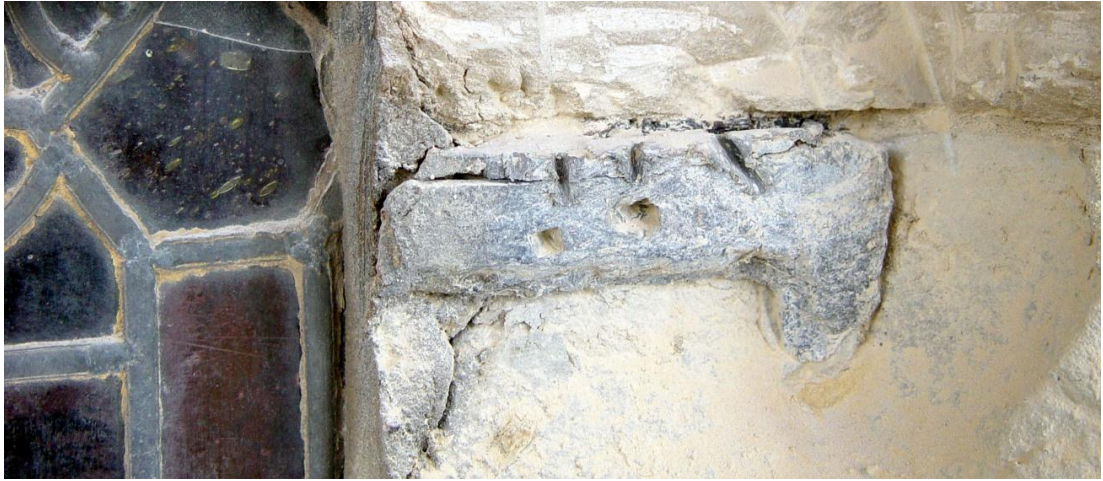
Fig. 7, Durham Cathedral, example of right angled ferramenta anchor end with lead encapsulation.
