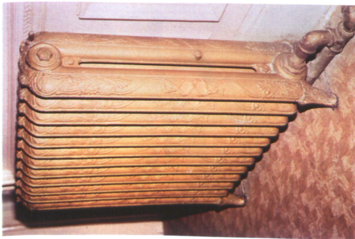
4.92 Corridor radiator in use in 1991.
