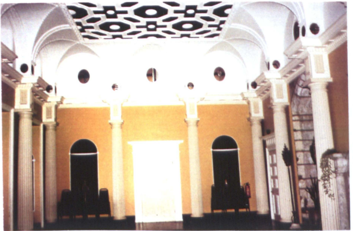
4.157 Great Hall/Saloon by John Carr, restored by S.D.K. and subsequently repaired, in 1993.
