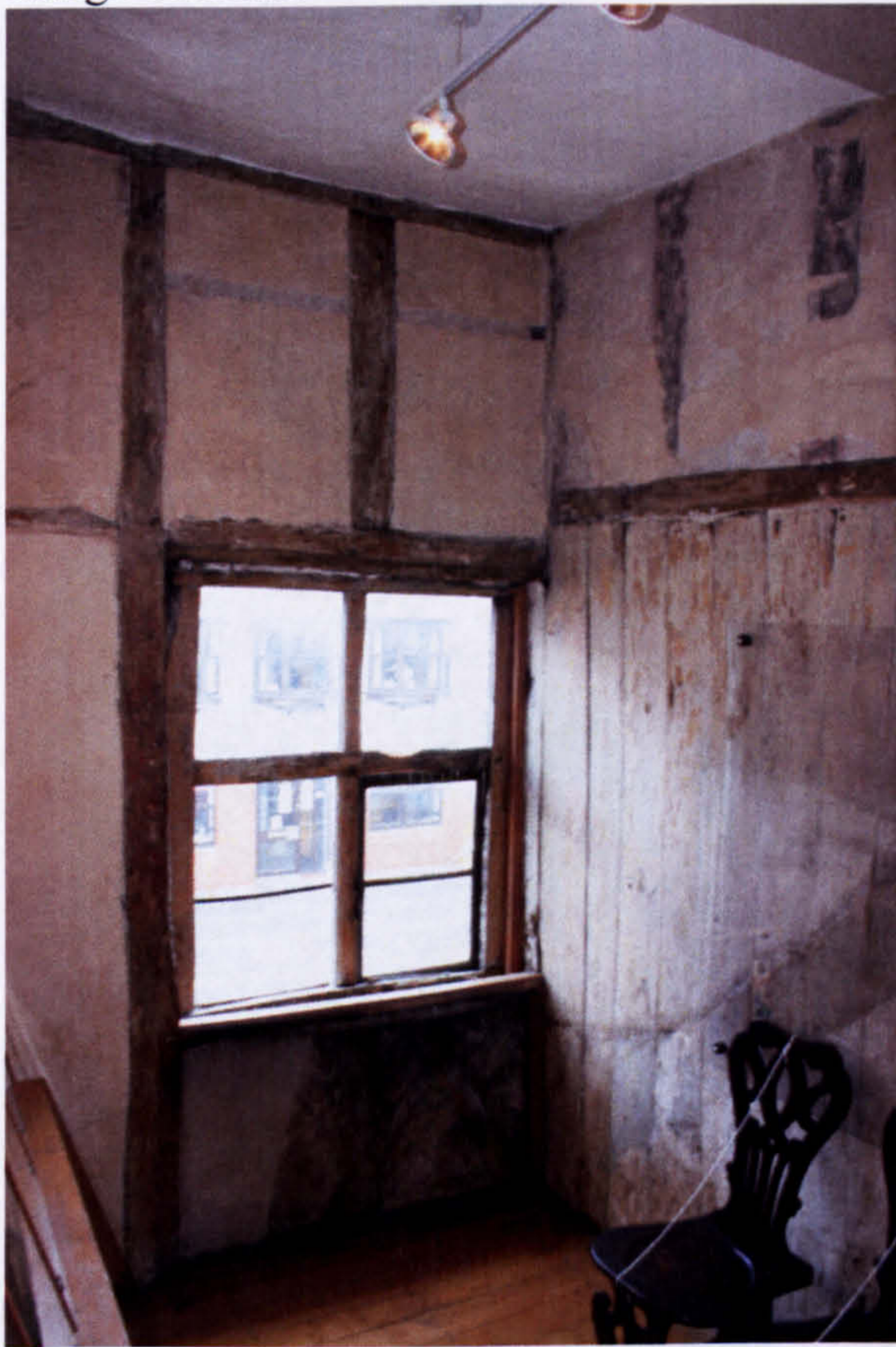
Fig. 40. 8 Charing Cross: first-floor level, north wall window and exposed herring-bone design beneath.
