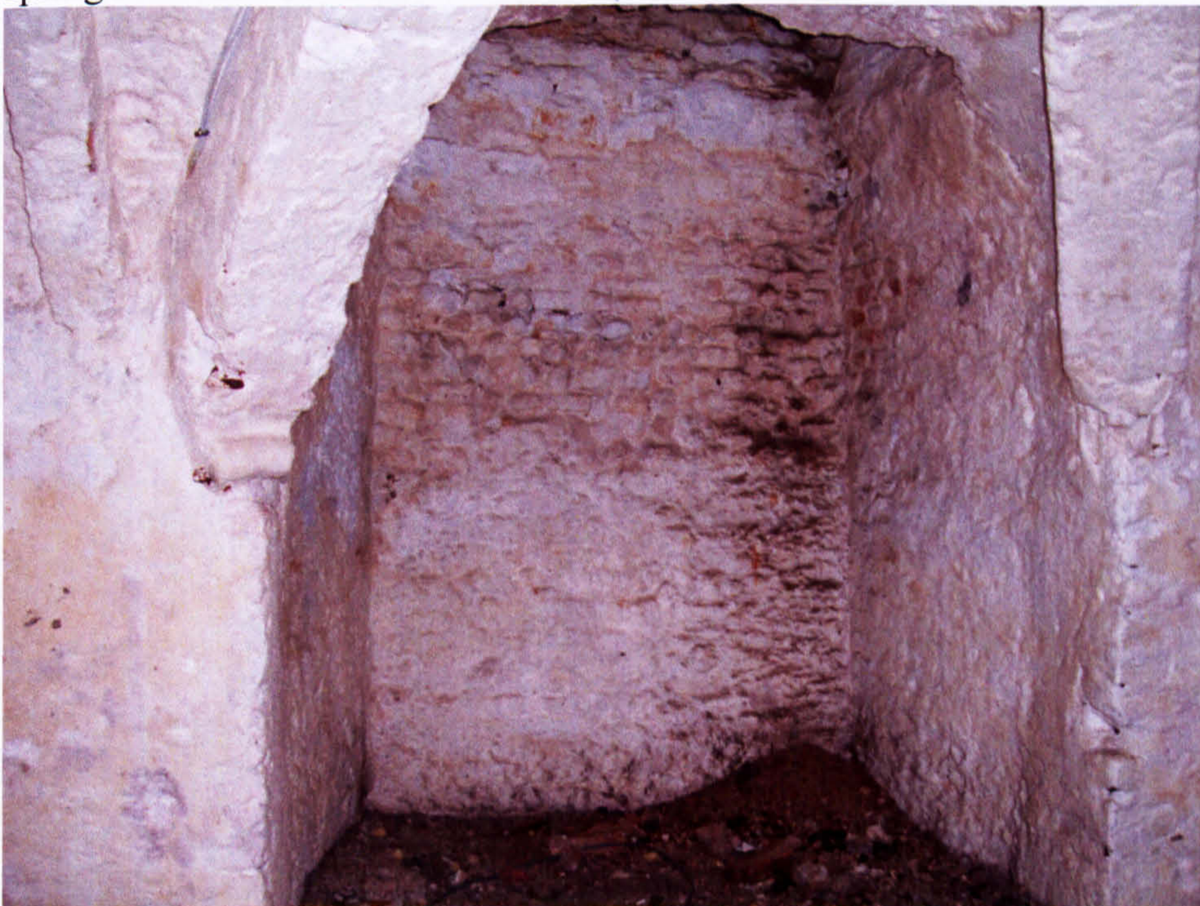
Fig. 32. 15 Bedford Street: side chamber in east wall of undercroft; re-used corbel at spring of north-east vault.
