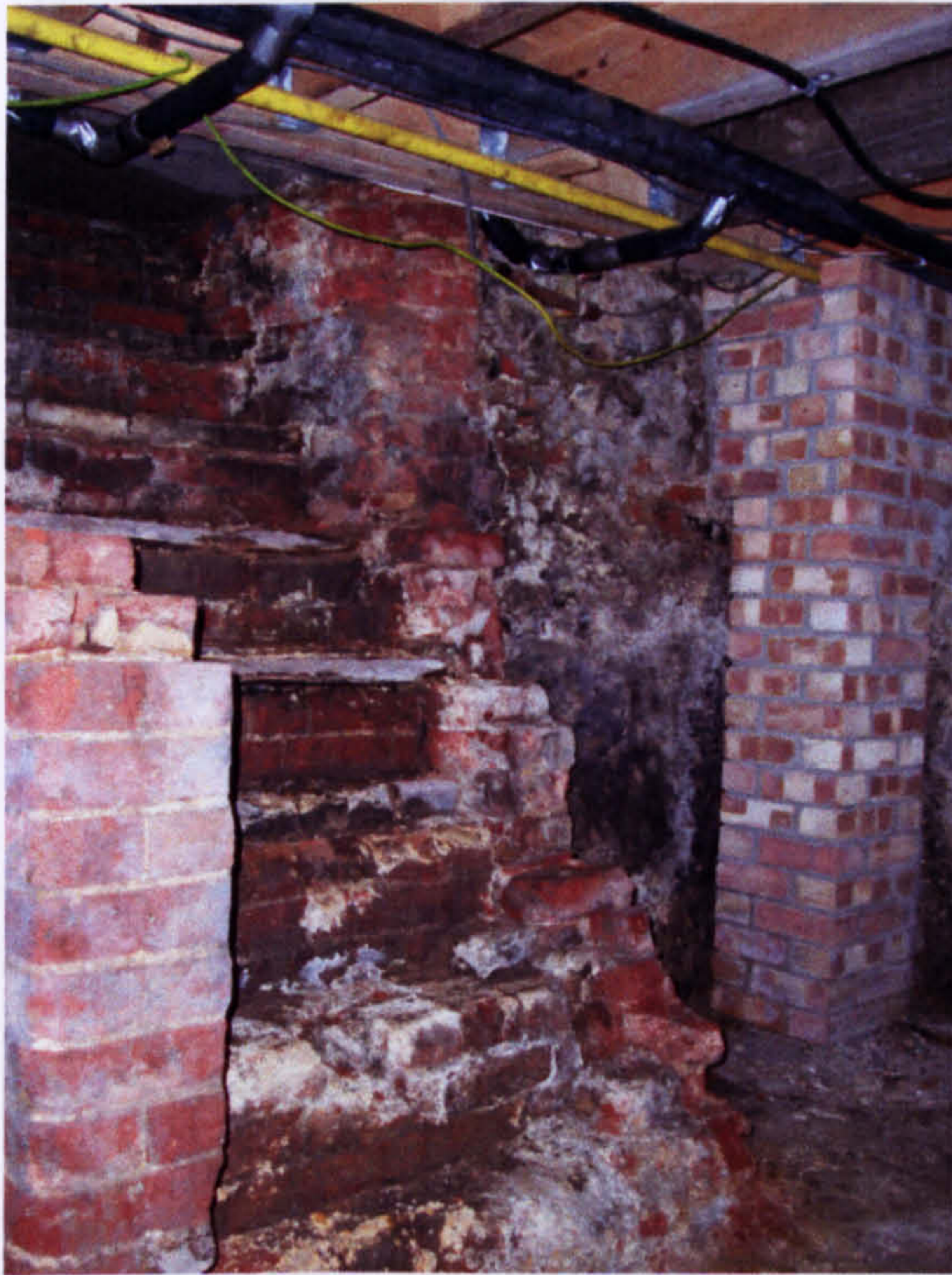
Fig. 29b. 15 Bedford Street: south-west corner of cellar 1 showing flint south wall and inserted staircase.
