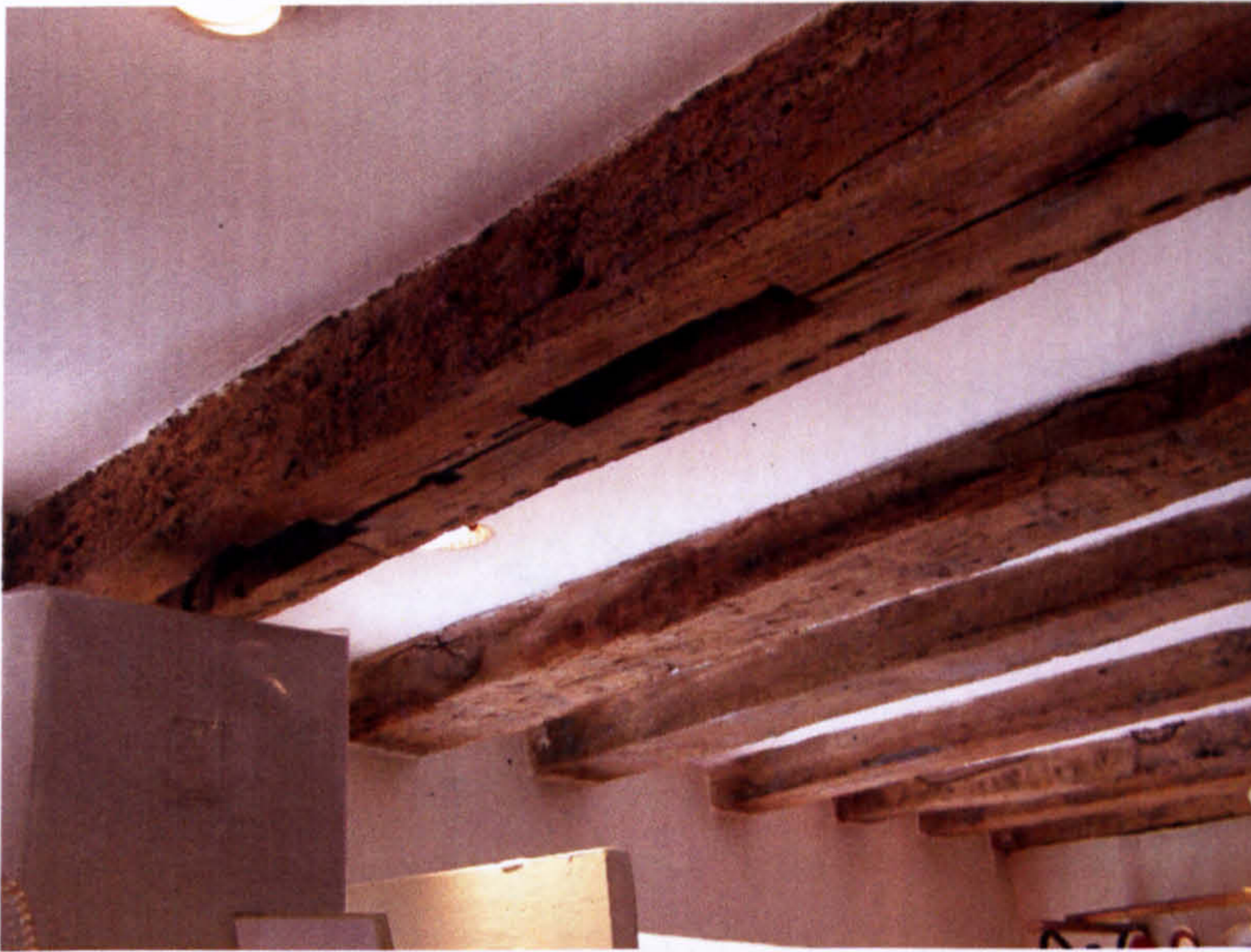
Fig. 72. 64 Goodramgate: empty mortice holes at the east-end of the ground-floor central truss.
