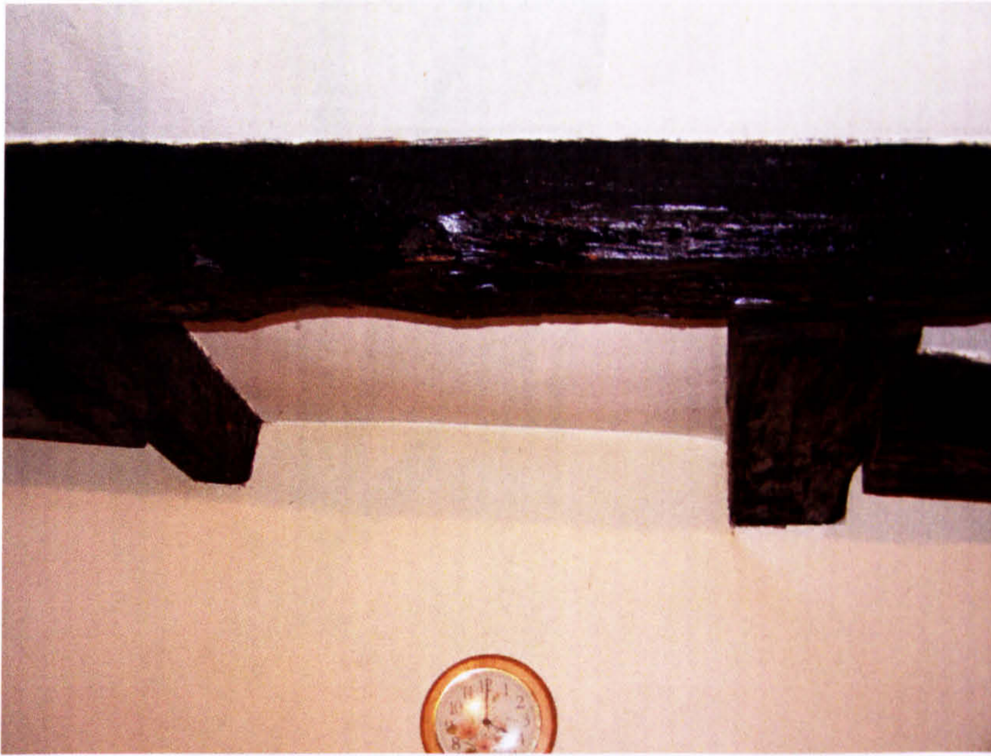
Fig. 84. 1 All Saints' Lane: ground-floor level, position of inserted chimney stack to the west of the unit.
