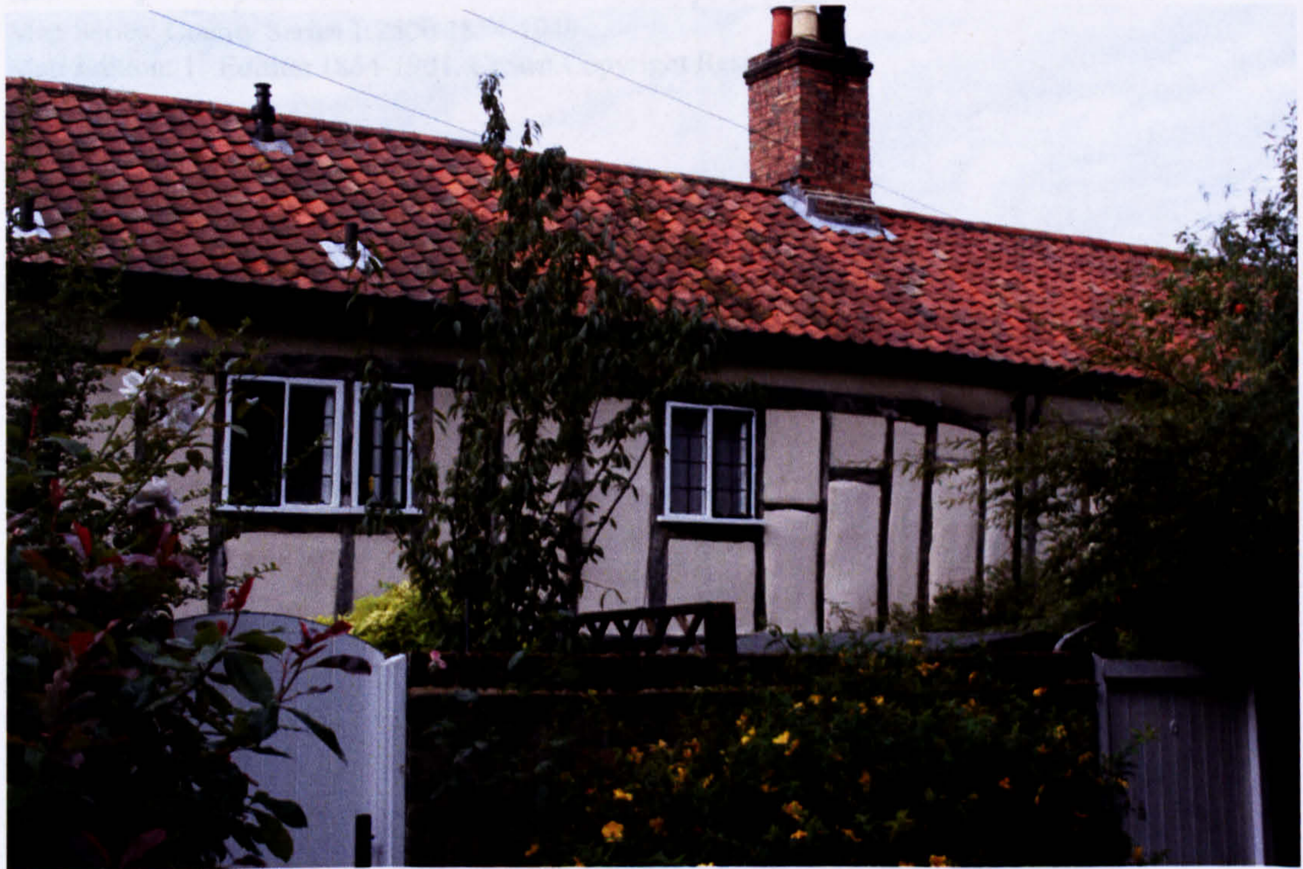
Fig. 50. 6 Gildencroft: remains of former timber window-sills at first-floor level (rear).
