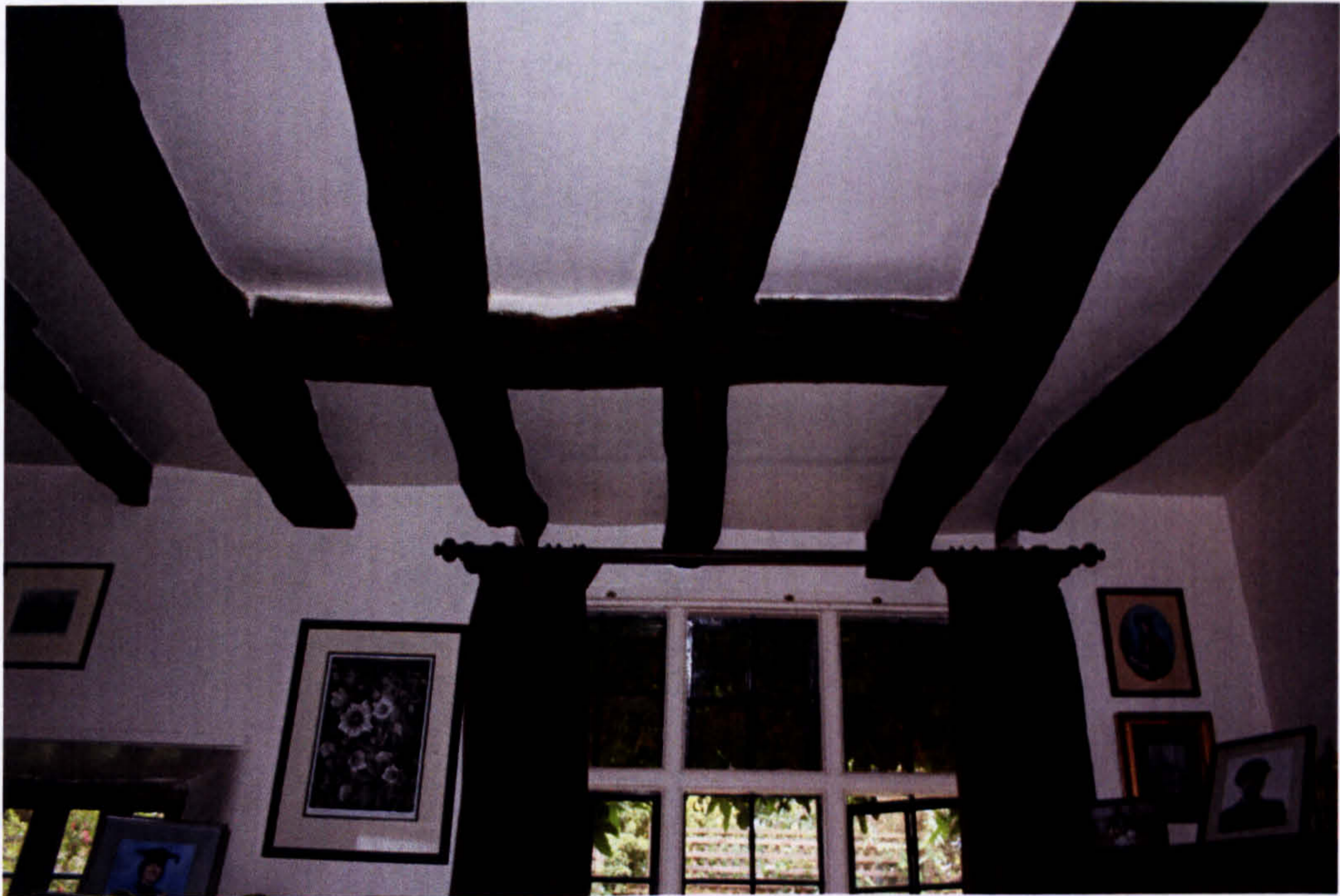
Fig. 55. 10 Gildencroft: ground-floor level, cross-beam in east bay delineating a former staircase opening.
