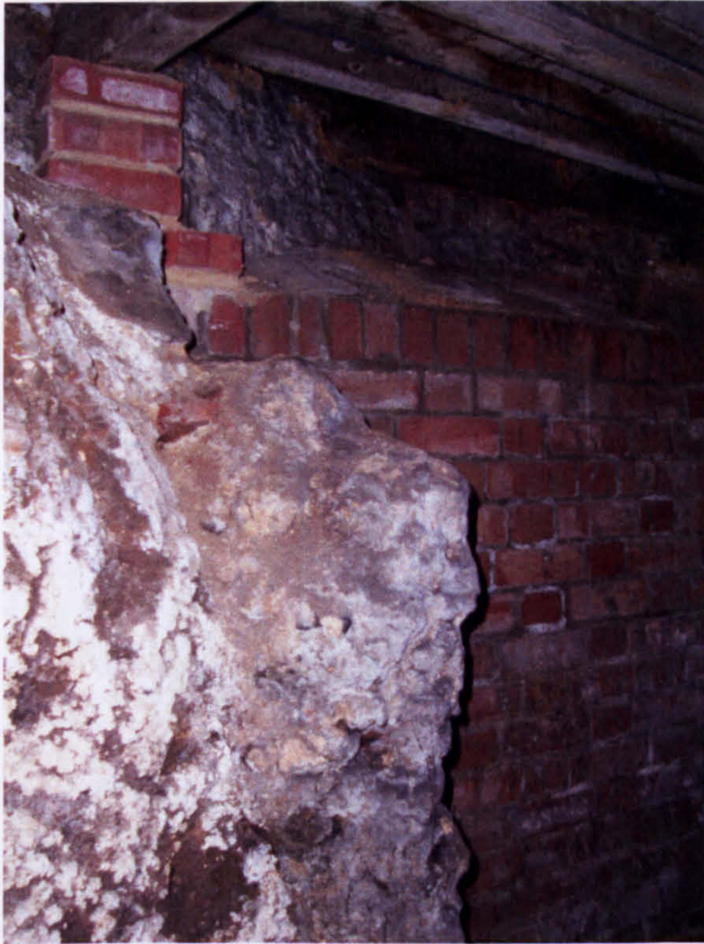
Fig. 28. 15 Bedford Street: flint walls in cellar 2; remains of north wall in foreground, and on east wall above brickwork in background.
