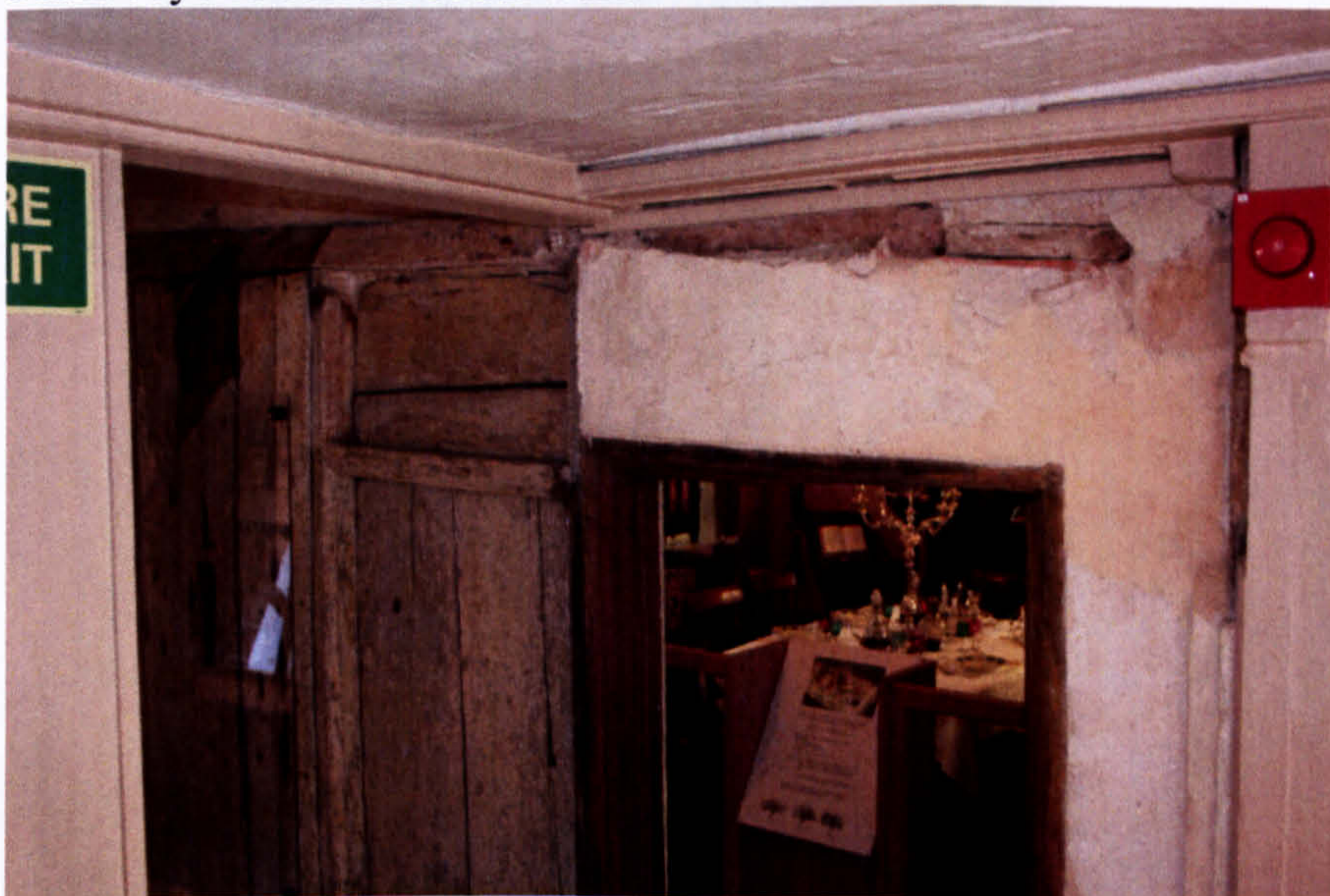
Fig. 42b. 8 Charing Cross: first-floor level, east partition showing extent of horizontal beam beyond current south wall.
