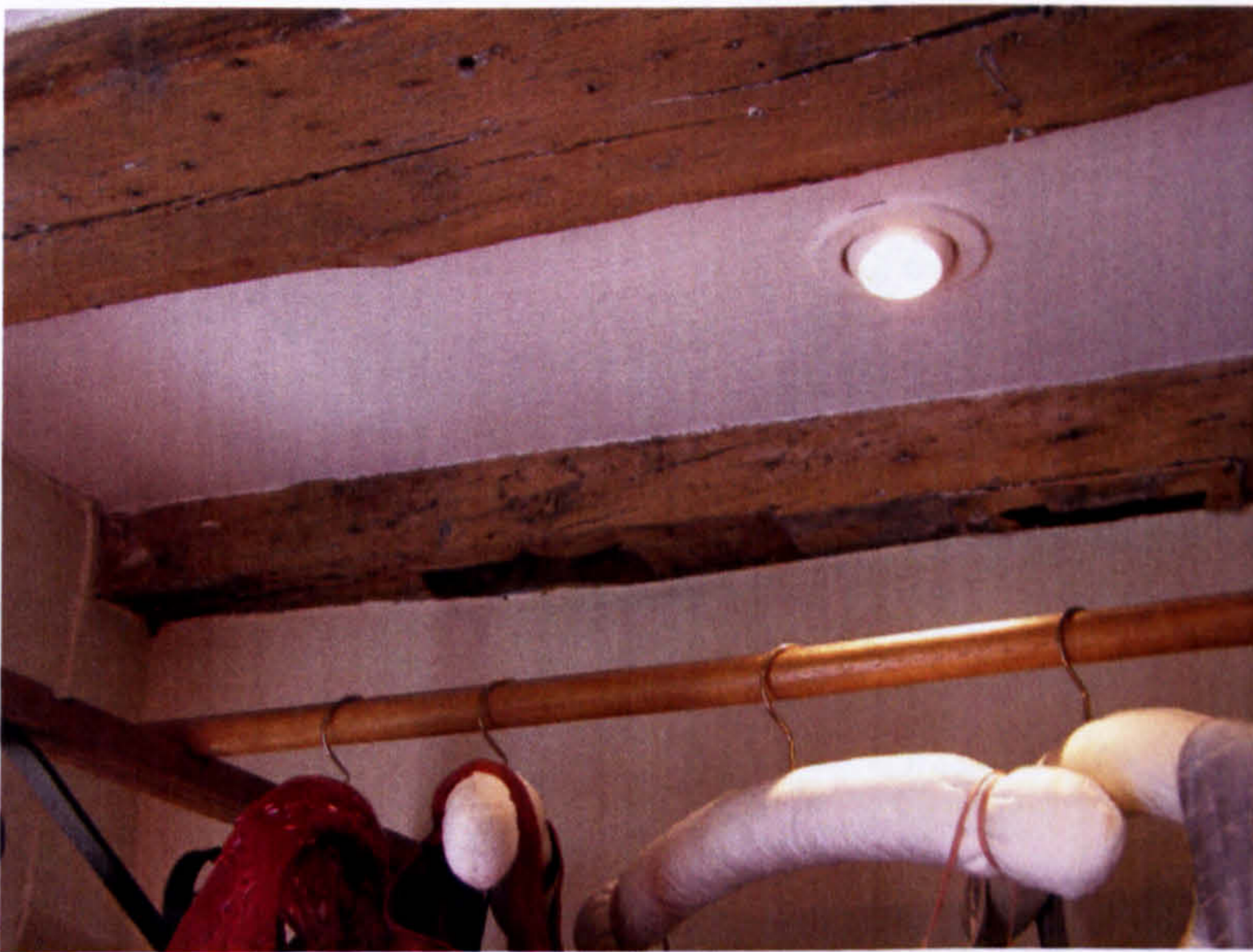
Fig. 73. 64 Goodramgate: empty mortice holes at the east-end of the ground-floor south truss.
