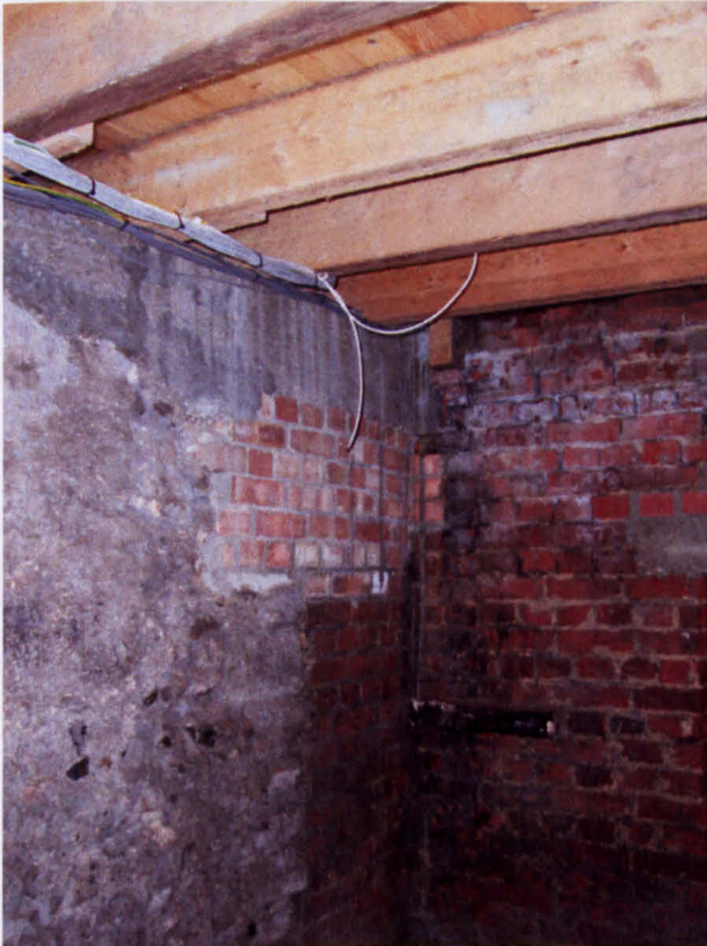
Fig. 29a. 15 Bedford Street: north-east corner of cellar 1, showing flint north wall to left.
