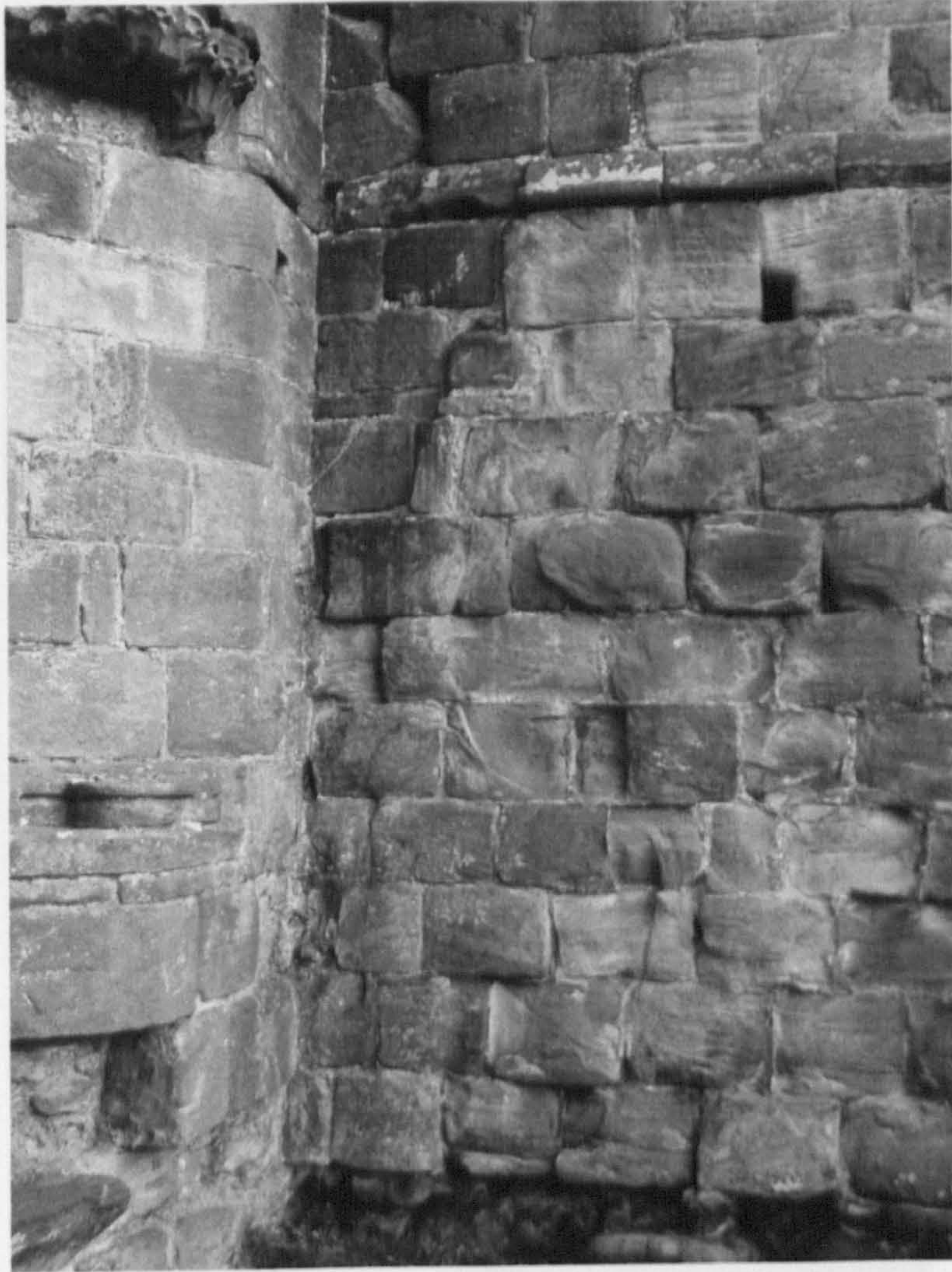
Figure 114: North-east corner of cloister, showing building break between nave south aisle and south transept.
