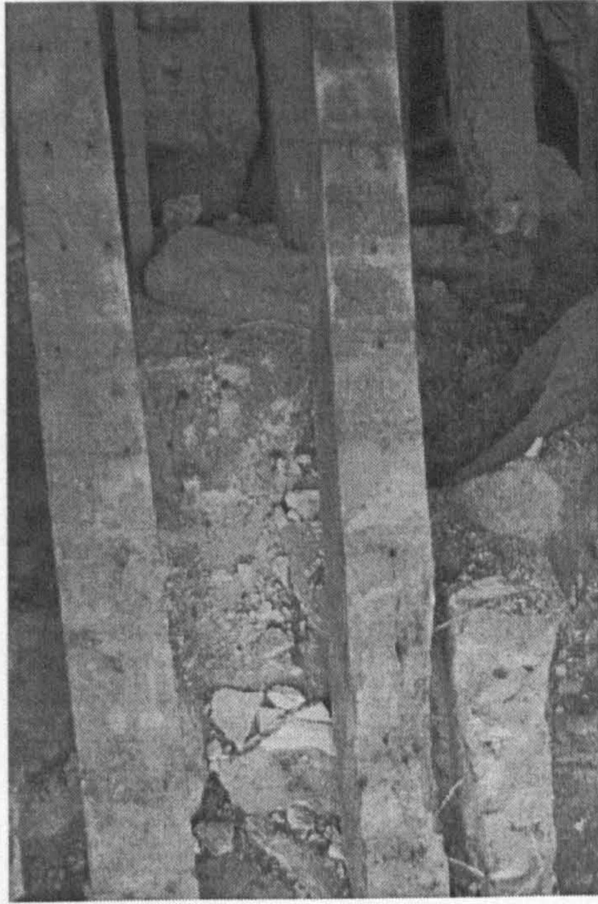
Fig. 144. Scarring left by the dismantling of chimney 2497, at the junction of the gatehouse and guest range (note the alterations to the principal rafter in the background)
