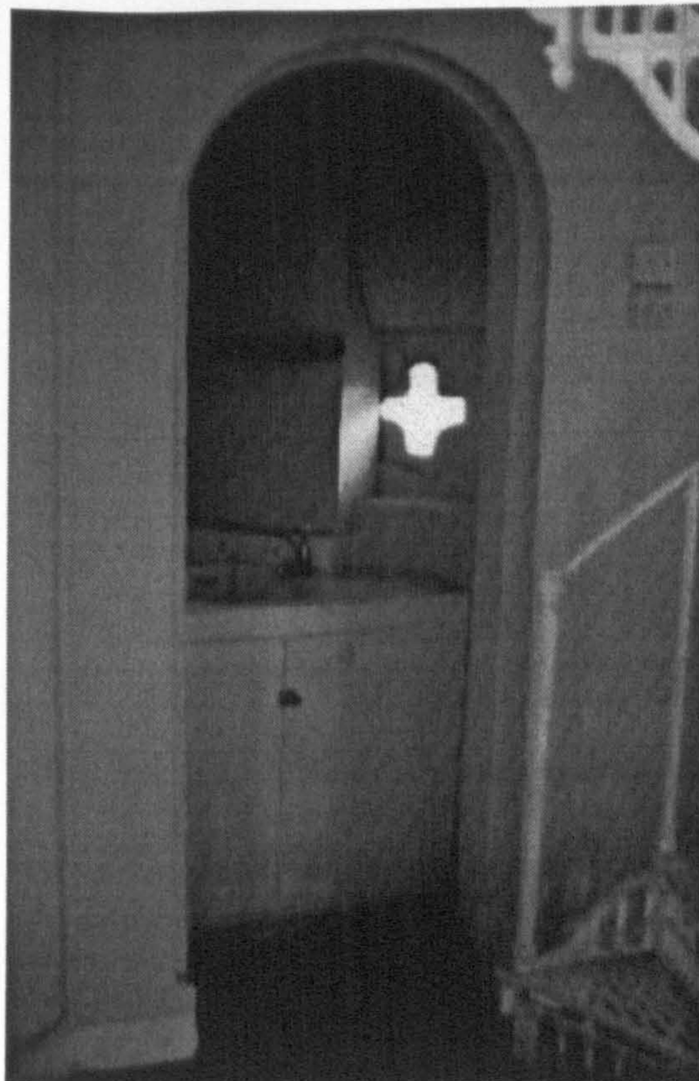
Fig. 101. Eroded sandstone carving in elevation 12, reputed to bear the arms of the founder, Henry II
