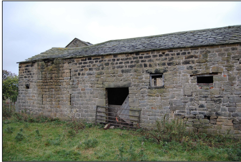
4.10 Part of the western elevation of the barn at Hollin Hall. The rest of the elevation shows signs of rebuilding, raising of the roofline with insertion and filling of doorways.
