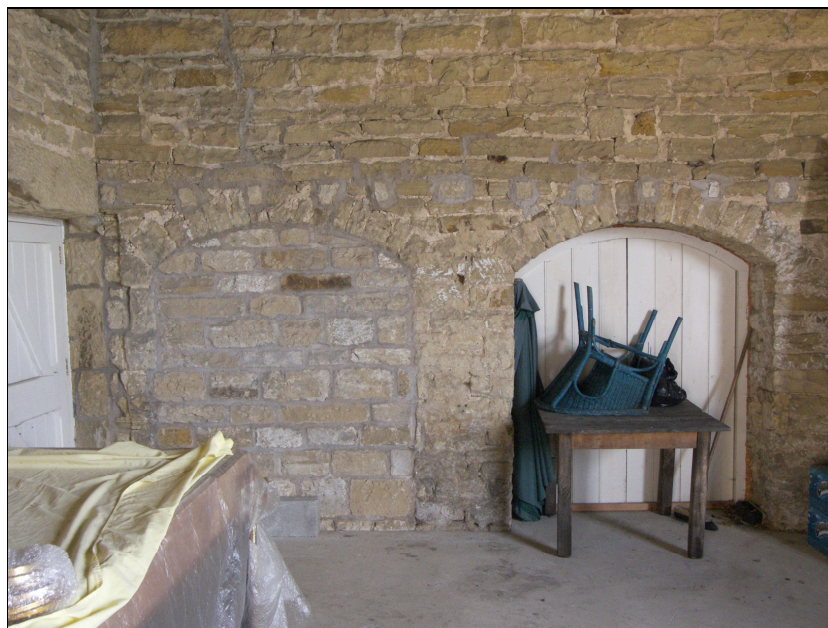
7.7 Blocked archways located in the western end of the barn at Stables Farm. Formerly provided access to another room in the western end of the building. A row of mortices above the arches indicate the addition of a new floor, possibly used a grain store.
