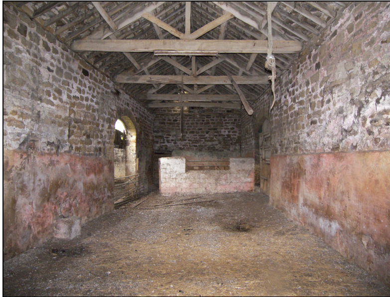
5.7 The reused barn at Lofthouse Grange that was altered during the eighteenth century. In the left of the image are insertions for nineteenth-century machinery showing that the building has been subjected to several building phases.
