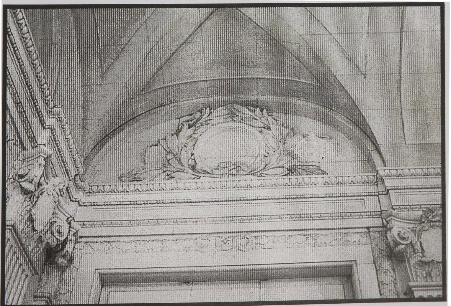
1309 - artists unidentified No. 10 CHT, Upper Staircase Landing detail, showing Caen Stone architrave with stuc pierre overdoor and coffering.
