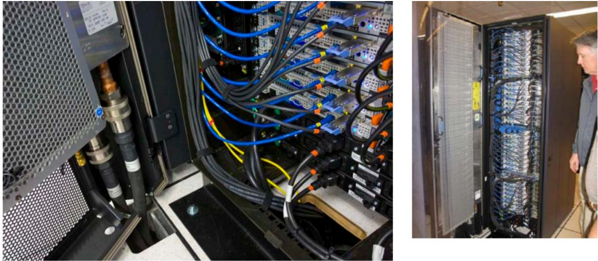
Figure 2-20 Back door heat exchanger water cooled system at Lawrence Berkeley National Laboratory (LBLN) (US DOE, 2009)
