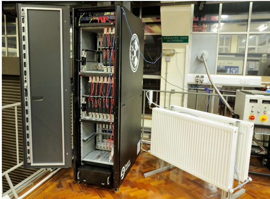
Figure 6-2 Photo of the full immersed liquid-cooled computer cabinet (left) with 11 nodes and passive radiator (right) in the university lab
