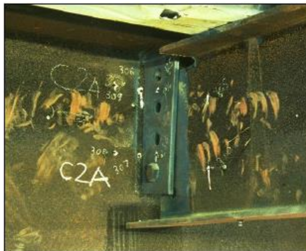
Figure 2: Fin-plate connection failure in Cardington test
