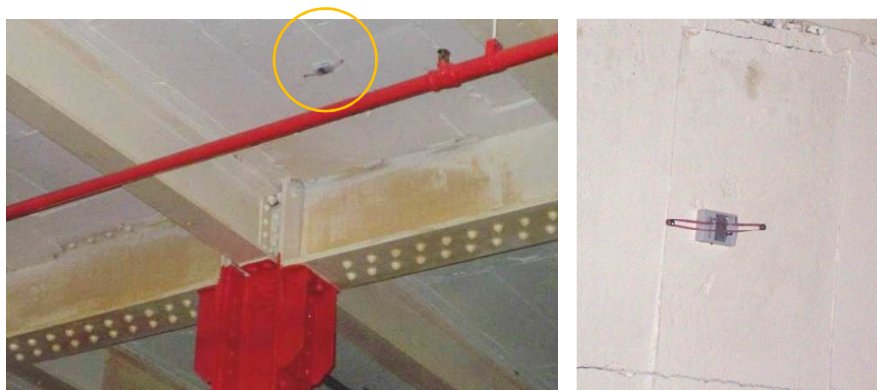
Figure 4.7 Temperature and humidity logger mounted on the ceiling under the green roof to measure ambient air temperature
