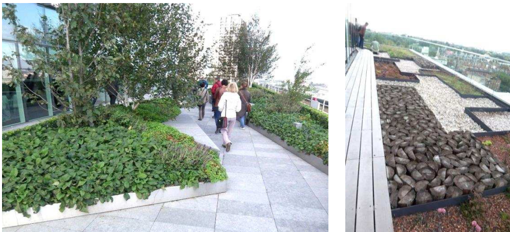
Figure 2.2 Intensive (garden) roof with trees and shrubs providing a recreational area for office workers (left). Mixture of extensive and semi-intensive green roof designed to promote biodiversity (right). Both green roofs were installed on a high-rise office building in London. (2010)
