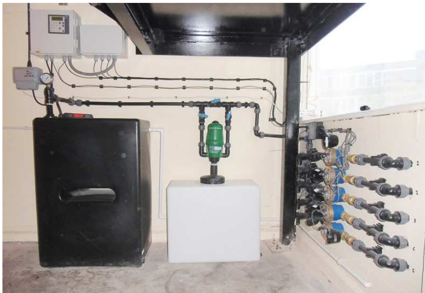
Figure 7.9 Irrigation control and monitoring system of the test beds (2012)
