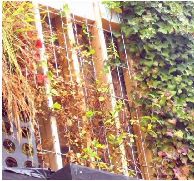
Figure 7.2 Climber system 12 months after the installation. Plants failed to establish and provide foliage cover (2013)
