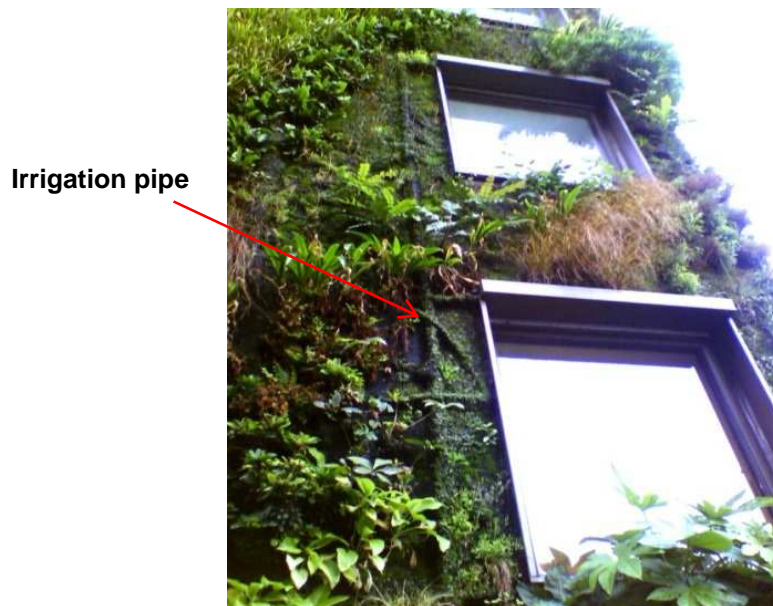
Figure 7.7 Irrigation for the felt system, pipes and tubes are spread under the top layer of felt distributing water to the surface of the wall (2010)
