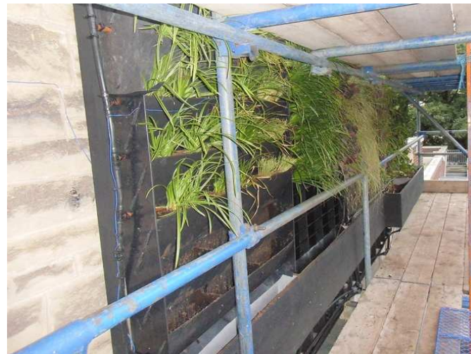
Figure D- 4 Test beds after the installation of living wall panels. Gutters and containers were placed at the bottom of the systems to collect excess water discharged from each system
