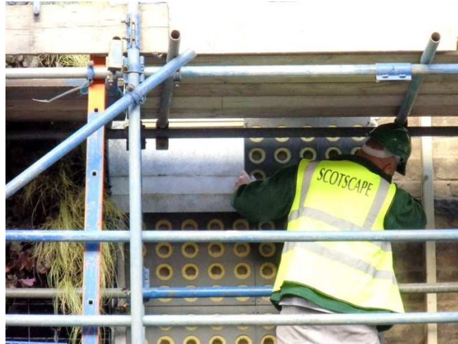
Figure D- 3 Installation of hydroponic panels. The panels are usually pre-planted although plants were inserted into the 'pockets' in situ for the test bed due to the limited installation time and lengthy delivery time.
