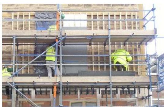
Figure 5.14 Timber battens before test bed installation. Strips of insulation panels were inserted between the battens behind the 'added insulation' section of the test beds at the top
