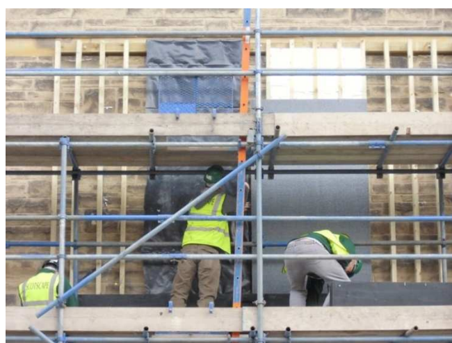
Figure D- 2 Installers fixing a black sheet of waterproof membrane for Compost and Trough systems, and a grey weatherproof board for the Hydroponic system.
