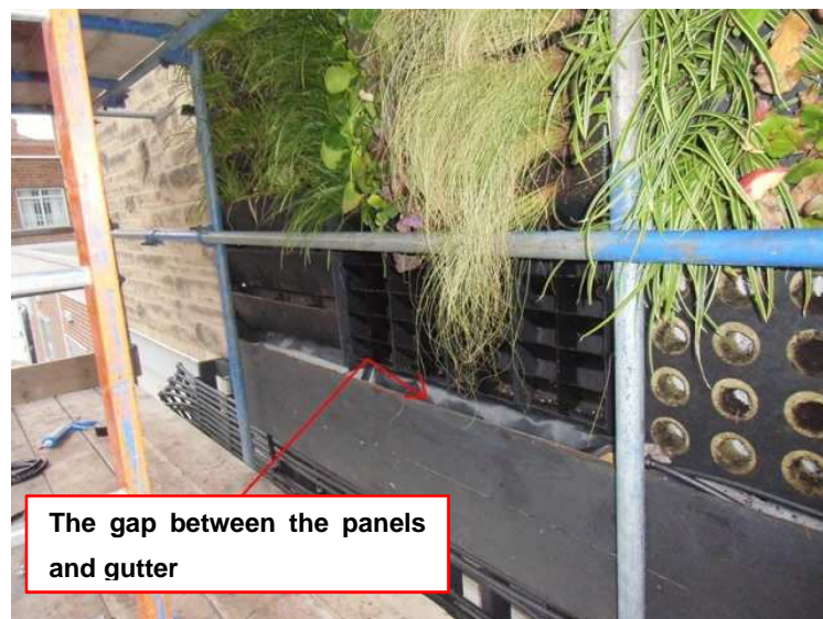
Figure 7.12 Image of the bottom of test beds before covering the gap between the living wall panels and the gutter (2012)
