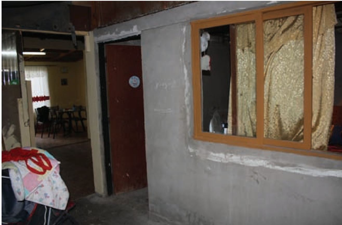
Fig. 5.58 Case 05, view of the two rooms built on the rear sector of the enlarged unit.
