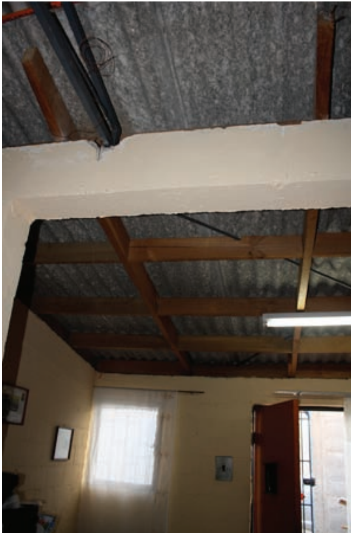
Fig. 5.56 Case 05, the original structure was extended through an opening in the back wall.
