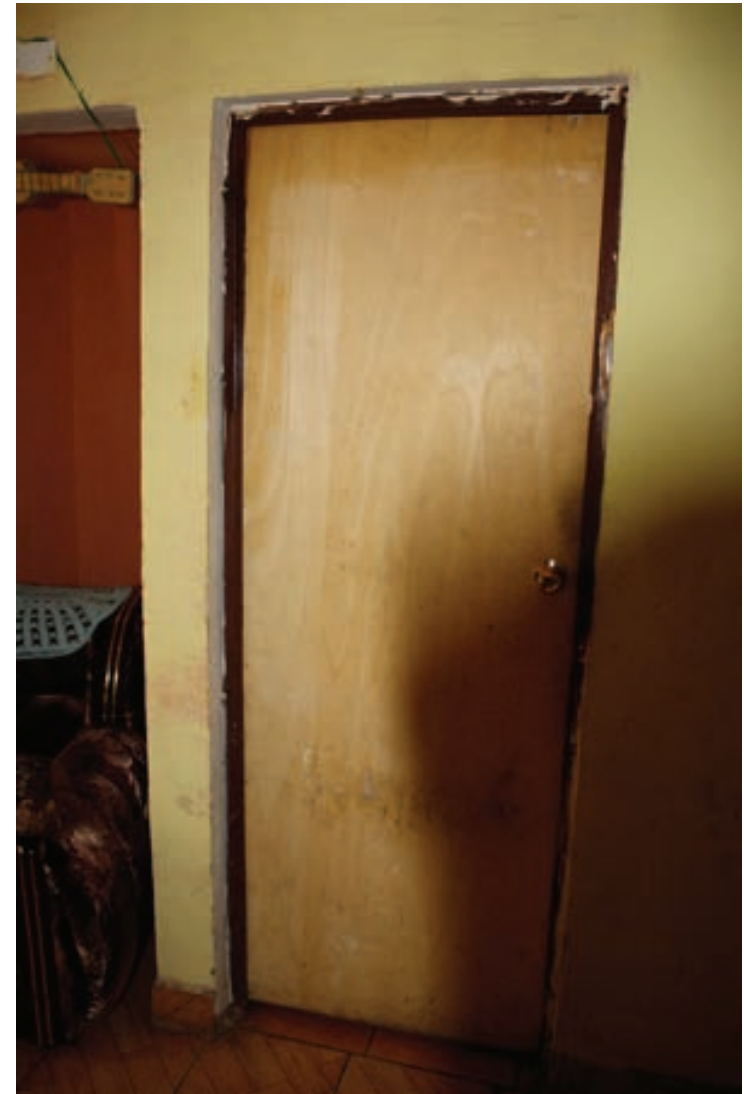
Fig. 5.72 Case 06, bathroom entrance.
