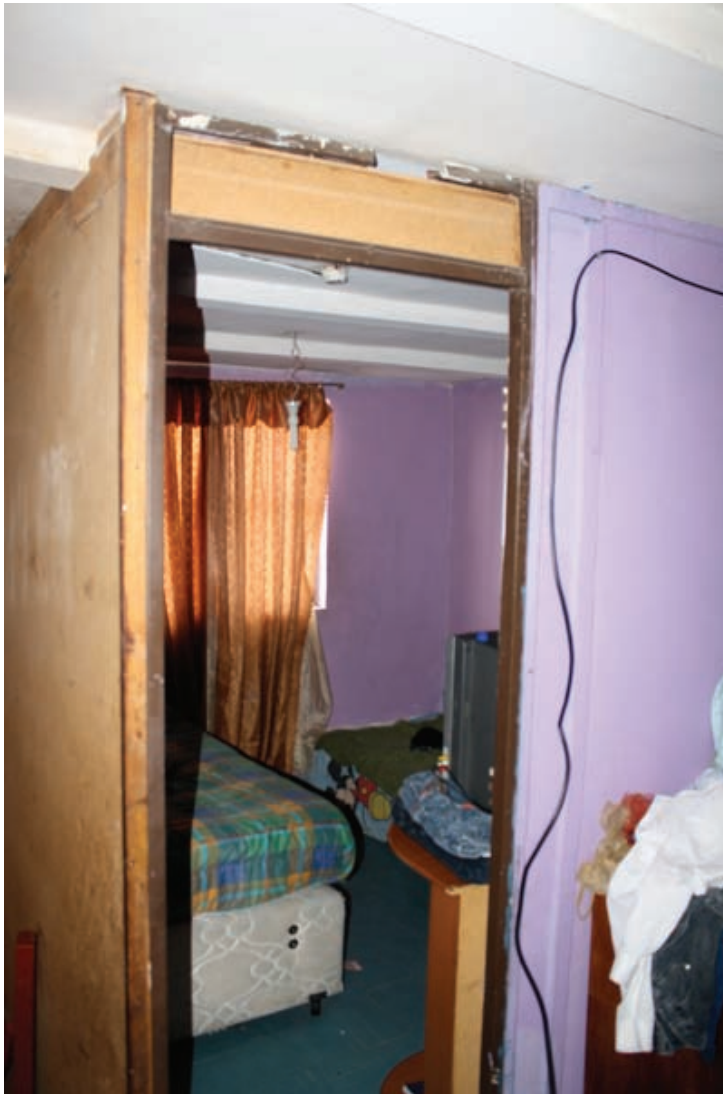
Fig. 5.18 Case 02, absence of doors between rooms.
