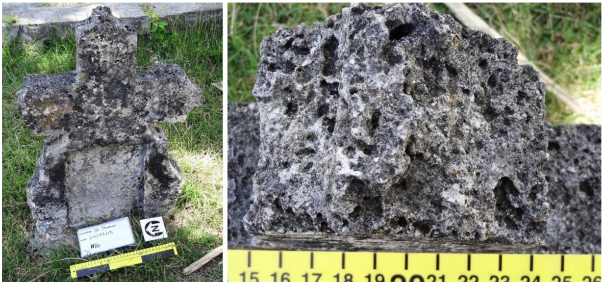
Figure 3.10 Example of a coral stone ( Monastrea annularis ) monument from St. Thomas Parish Church, exhibiting erosion likely caused by acid rain.
