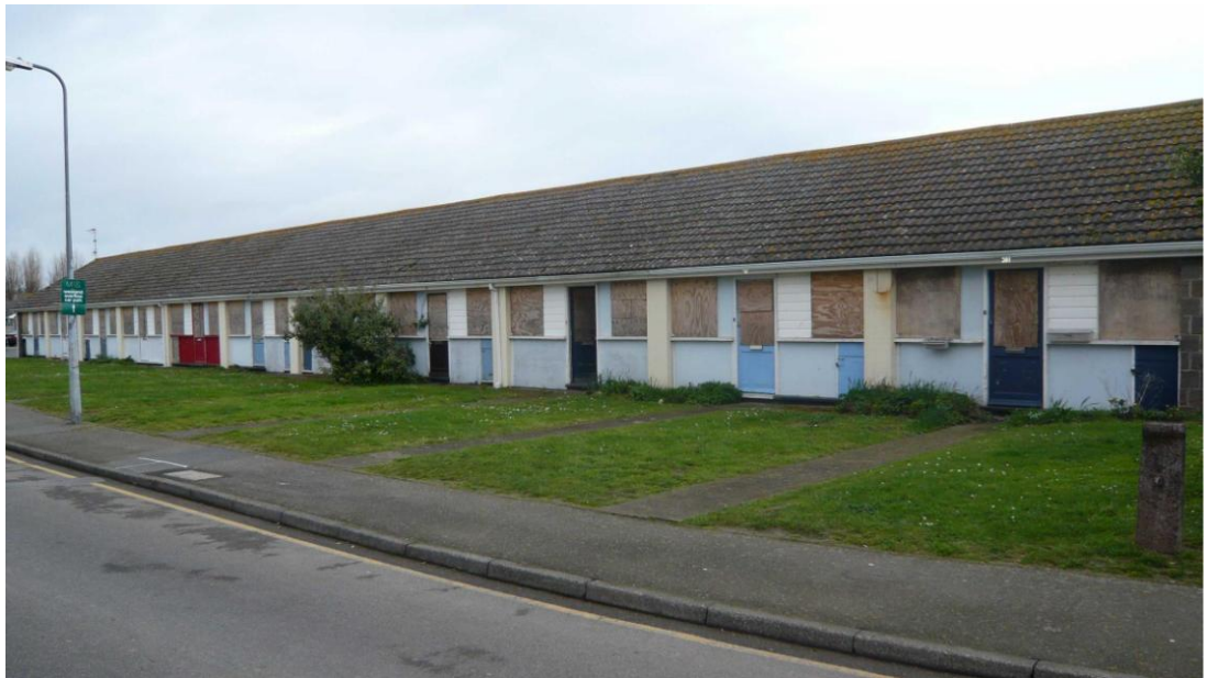
Figure 3-13: View of School road bungalows starting from #68 (used for Test 8) on the right then #67 (used as a control room for test 8) and sequence continues till #58 on the far left.
