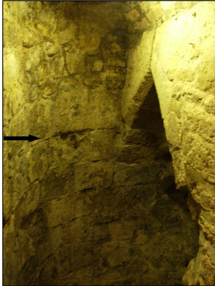
Fig. 5.25: The wall bordering the steps inside the porch annex, with the height of the medieval masonry highlighted with arrow. Note the medieval arched doorway that leads to the tunnel and remainder of steps (Photograph author's own).
