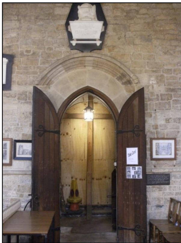
Fig. 5.26: The current doorway leading from the church interior to the porch interior. Note the stone arch above the door is not in its original position. It is also rounded, yet the arch from the interior of the porch is pointed (Photograph author's own).
