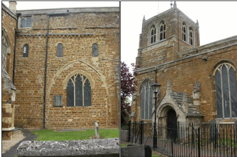
Figs 5.28 & 5.29: The eastern portion of the south exterior wall of the church. Note the extensive rebuilding works and evidence of architectural changes to the building fabric (left); the western portion of the south wall of the church and the porch over the crypt entrance.
