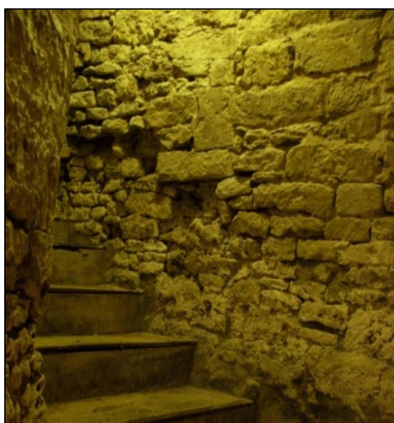
Fig. 5.24: The tunnel of steps leading to the crypt. Note the modifications to the walls above the steps (Photograph author's own).
