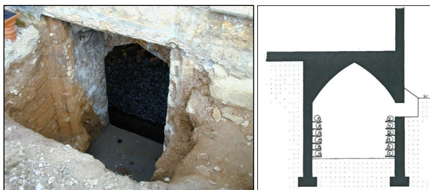
Figs 5.5 & 5.6: One of the southern windows of Rothwell chancel chamber from the exterior (Reproduced with permission from Rothwell Holy Church authorities) (left); section through chamber showing the position of windows (Adapted from Garland et al 1984: 237). Note the deliberately lowered ground level to the exterior allowing light to enter and making the chamber and contents visible from the exterior.
