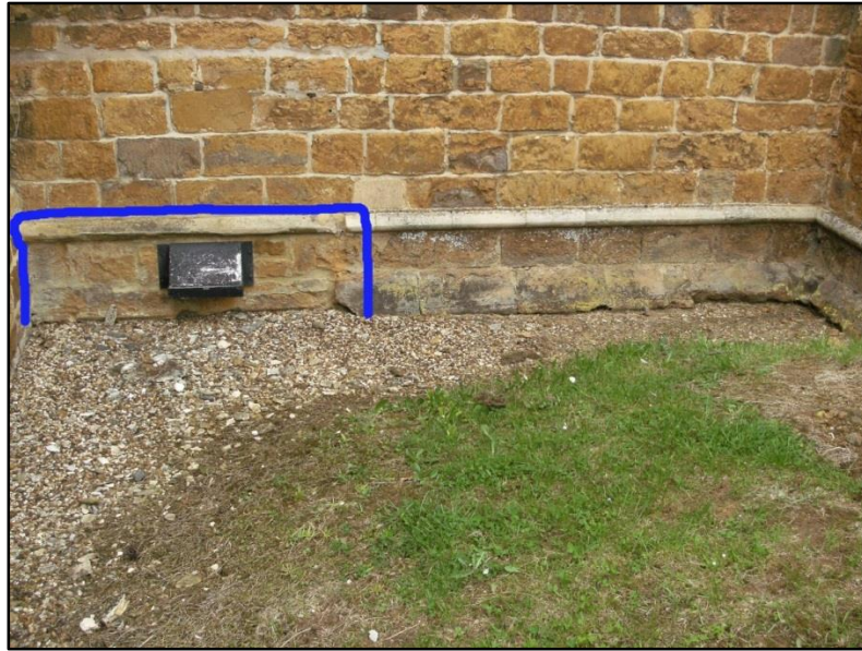
Figs 5.17 & 5.18: The westernmost of the two windows in the south wall of the crypt. Note how the window aperture extends upwards above the height of the crypt ceiling (top). The exterior of the south wall of the church showing the top of the now blocked up westernmost window into the crypt, highlighted in blue (bottom) (Photographs author's own).
