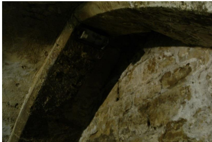
Fig. 5.31: Aperture in the ceiling at the east wall of the crypt (Photograph author’s own)
