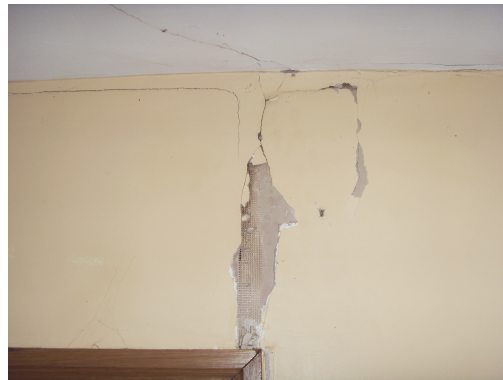
(c) Cracking and spalling plaster to upper right of living room doorway
