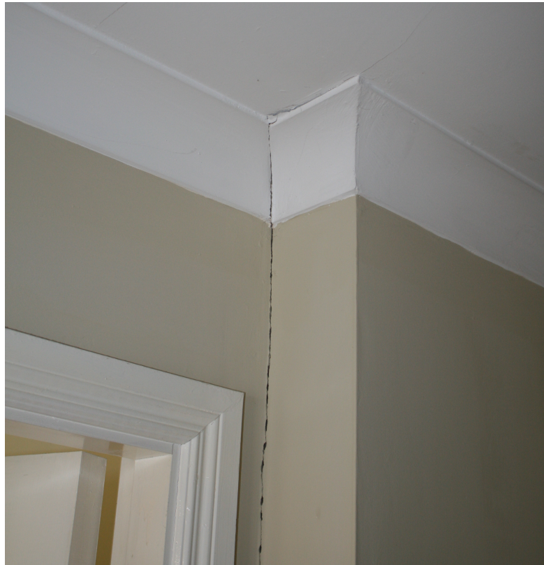
Figure 5.5: Cracking of plasterboard at wall/wall interface in Property A (with permission from Aidan O'Connell Associates).
