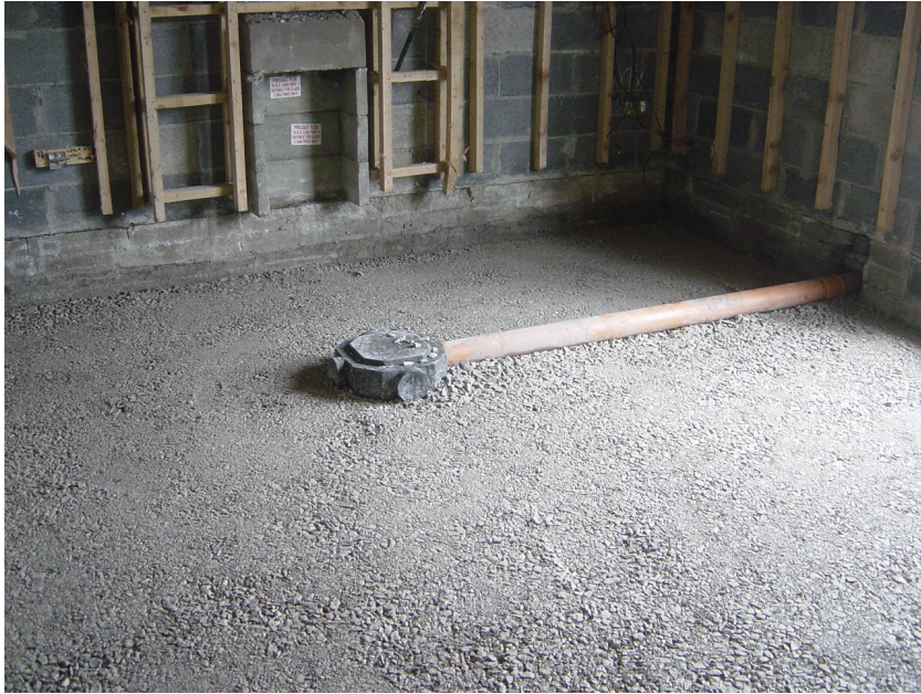
Figure 4.13: Replacement of fill material and radon sump. (used with permission of Aidan O'Connell associates).
