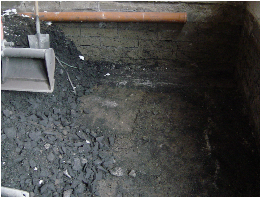
Figure 4.12: Removal of defective fill material from an Irish property, showing the natural material at the base of the foundation (used with permission of Aidan O'Connell associates).
