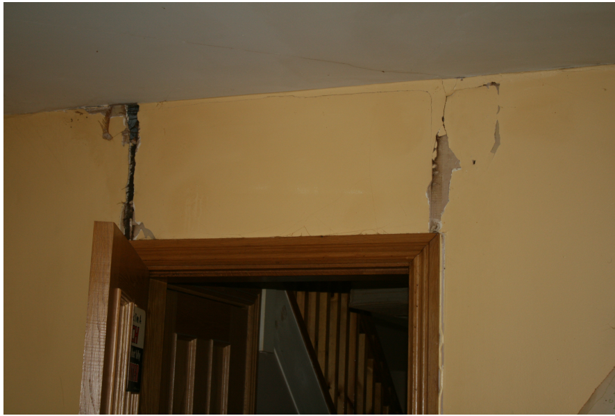
(a) Cracking to the plasterboard above the living room door. Images b) and c) show the cracks in more detail
