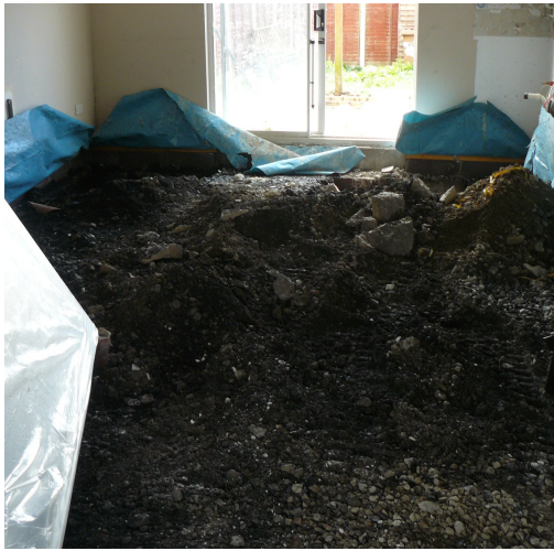
(a) Fill material below the kitchen area, with the double doors at the rear of the property.
