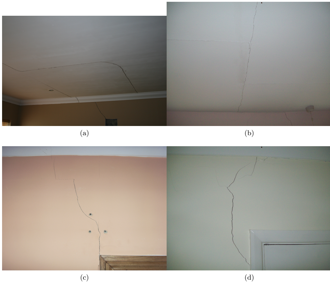
Figure 4.4: Damage to residential properties caused by pyritic heave (a & c) and foundation settlement (b & d). Images a & c used with permission of Taylor Tuxford Associates, images b & d used with permission of Aidan O'Connell Associates.
