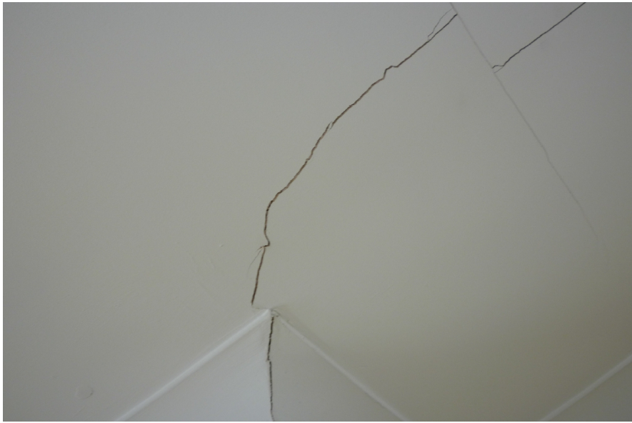
Figure 5.7: Significant cracks to the plasterboard finish of the ground floor ceiling at Property A (with permission from Aidan O’Connel Associates).
