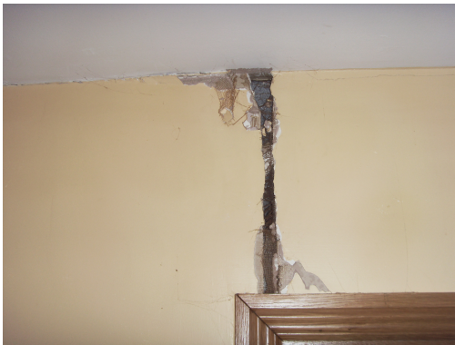
(b) 10 mm crack to upper left of living room doorway
