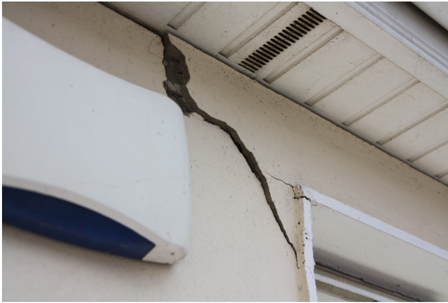
Figure 5.8: Cracking to the render around the living room window at Property A (with permission from Aidan O'Connel Associates).
