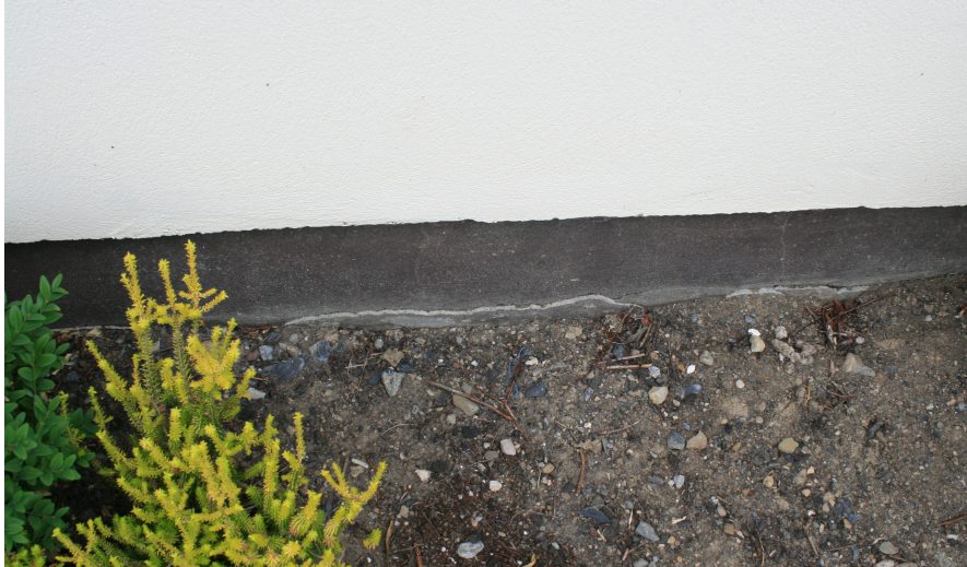
Figure 5.9: Damage to external walls of Property A (with permission from Aidan O'Connel Associates).
