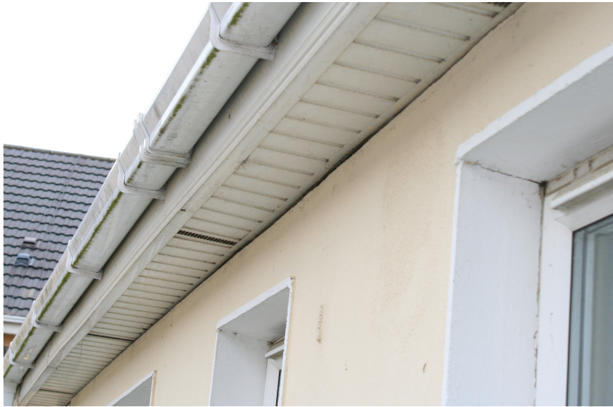
Figure 5.10: Gap at soffit level at Property A (with permission from Aidan O’Connel Associates).
