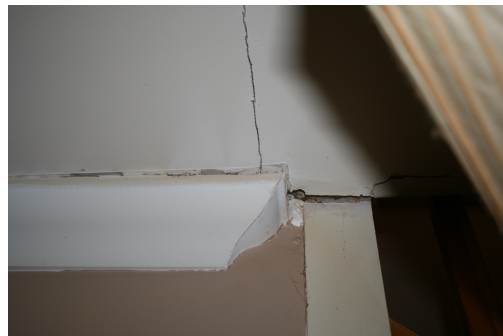
(e) Cracking and upward movement to stairwell, maximum movement 6 mm
