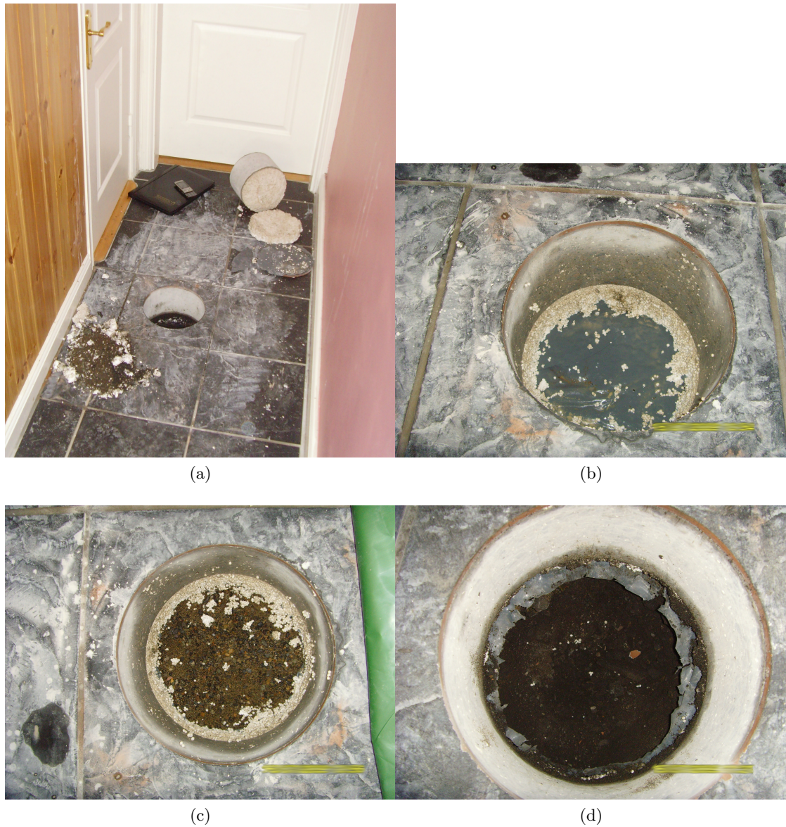
Figure 4.9: The process of coring through the floor slab and taking samples for geotechnical testing.
