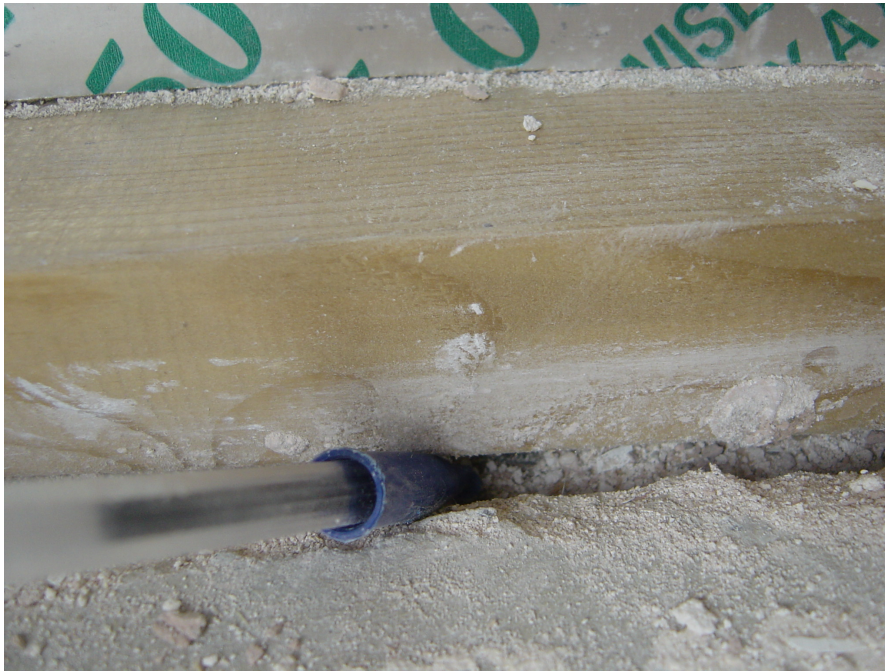
Figure 5.6: Uplift of an internal partition wall at Property A by approximately 5 mm (with permission from Aidan O’Connel Associates).
