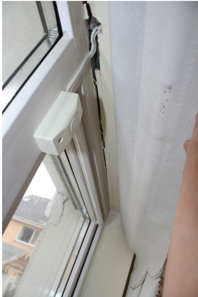
Figure 5.4: Gapping at top of window frame in the living room of Property A (with permission from Aidan O’Connel Associates).
