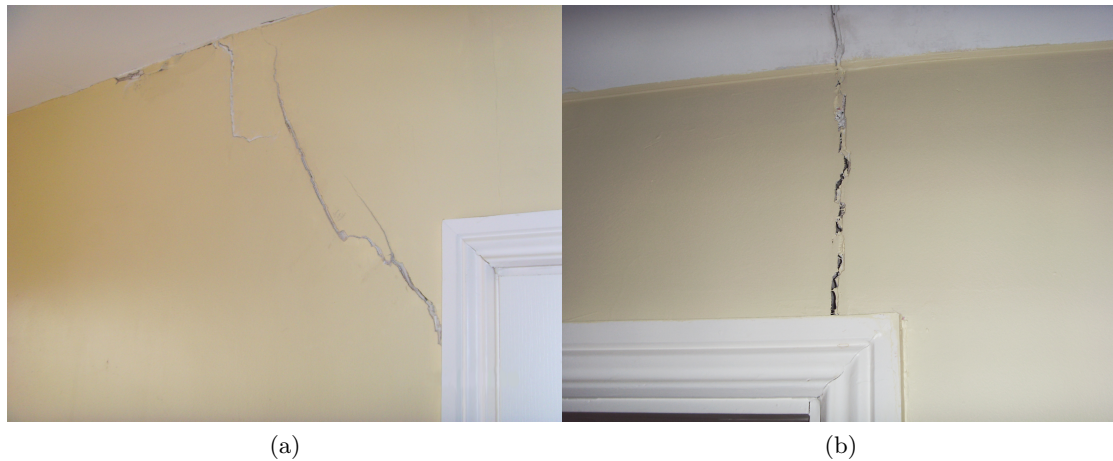
Figure 5.12: Cracking to ground floor walls at Property B (with permission from Aidan O’Connel Associates).
