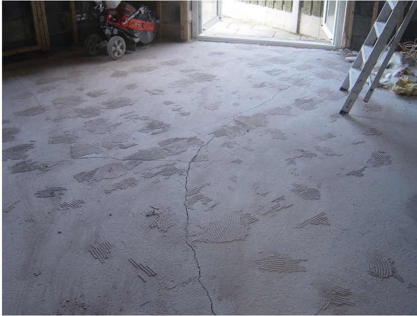
Figure 4.11: Stellate cracking of floor slab recorded during the remediation process (used with permission of Aidan O'Connell associates).
