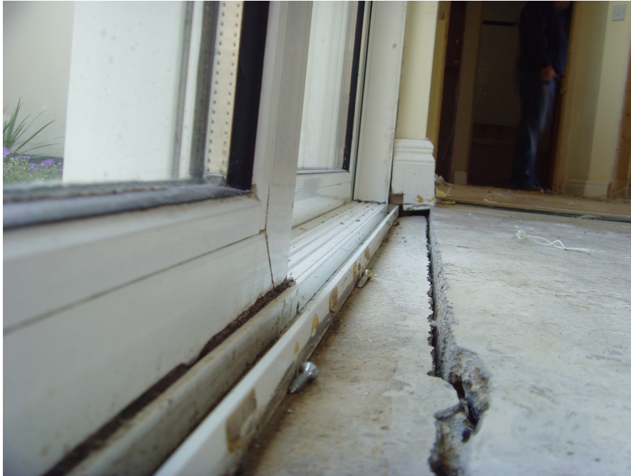
Figure 5.3: Uplift of the floor slab and displacement of skirting boards at Property A, uplift was recorded at around 6 mm in this area (with permission from Aidan O’Connel Associates).
