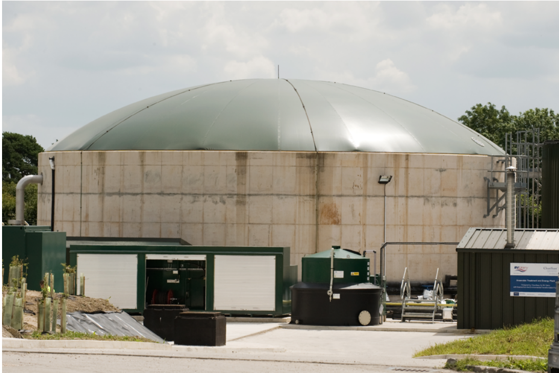
Figure 1.7. A process scale AD facility, located at a dairy facility. The digester has a 1000 m 3 capacity, taking in 200 m 3 of effluent daily.
