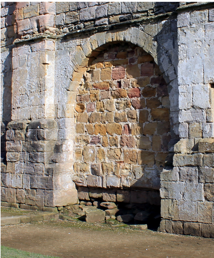
FIGURE 4-13. The wall recess of a book cupboard in the wall of the arm of the south transept, near the south door to the church at Fountains Abbey, West Yorkshire.
