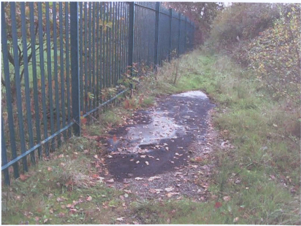
Figure 1.9: Fencing around the edge of Hoole Bank acid tar lagoon. Tar seepage is clearly visible outside the fence boundary as a result of tar migration.
