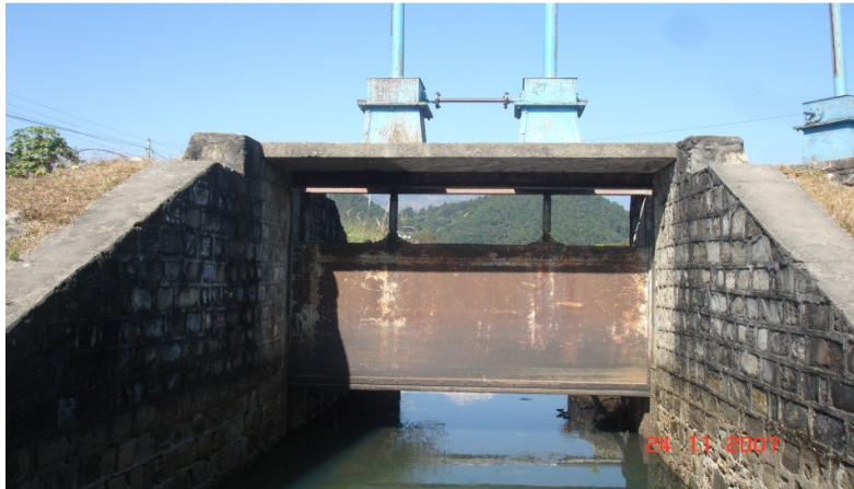
Photo 6.2 Open-Close Slot Gates in AMIS
