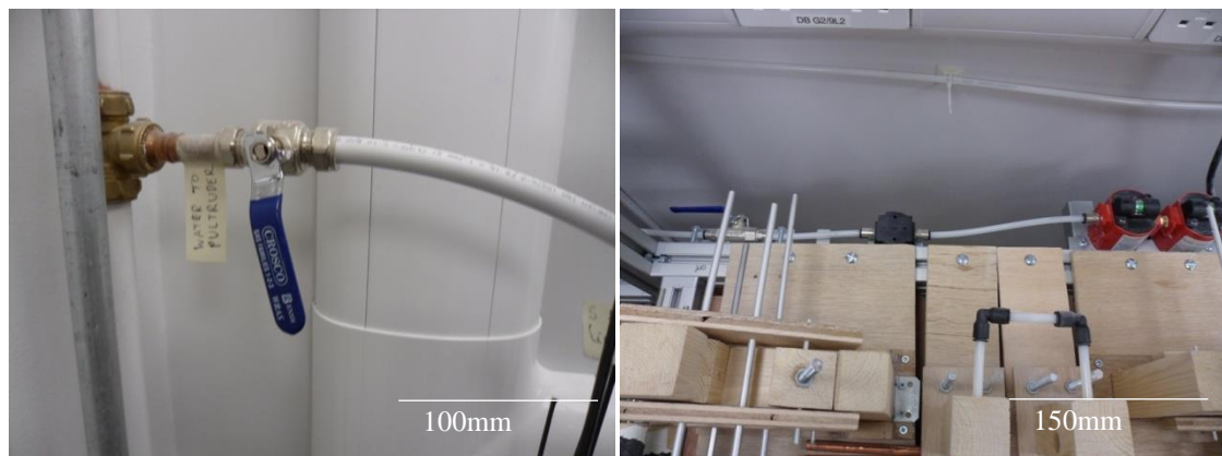
Figure A.10 Water tap and compressed air line.
