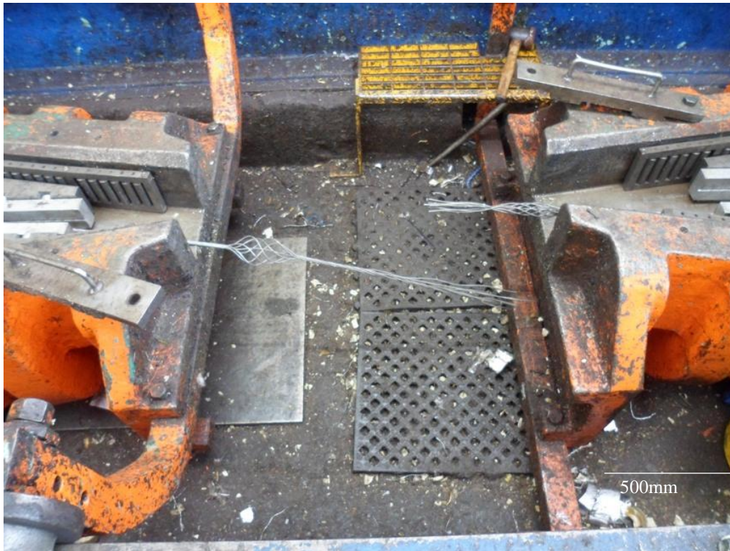
Figure 5.35 Birdcage failure of a steel strand.
