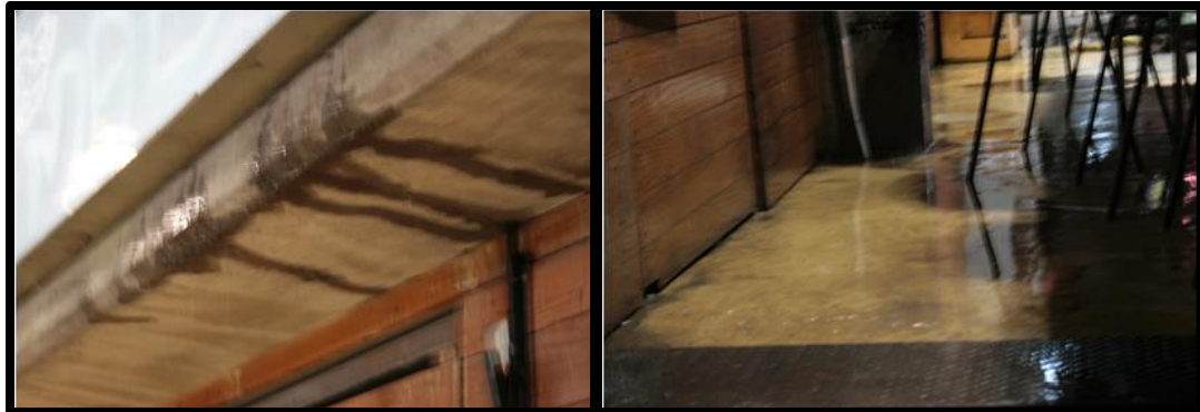
Figure 12 Leaks in the main building
