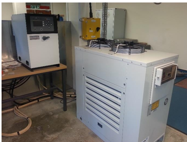
Figure 9: Induction furnace generator and water chiller for levitation induction furnace
