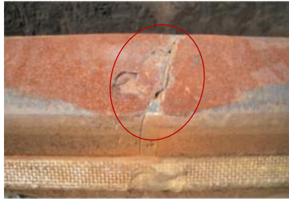
Fig. 1:23- Rail Head Metal Spalling in the Gap between Adjoining Rail at IRJs [27].
