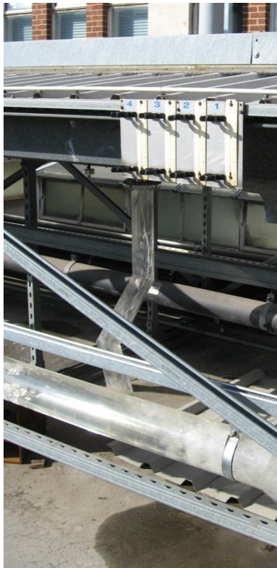
Figure 3.15 Image of Outlet C Tailpipe Configuration
