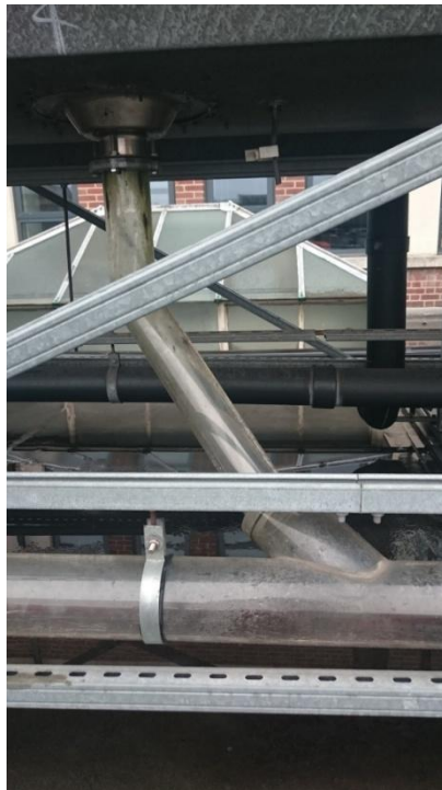
Figure 3.13 Image of Outlet B Tailpipe Configuration
