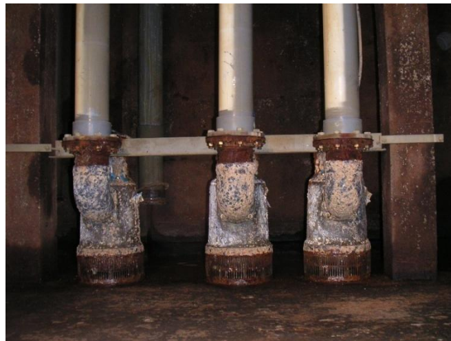
Figure 3.5 Image of the Submersible Pumps within the Sump
