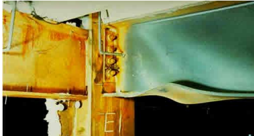
Figure 6: Beam buckling in Cardington (Newman et al. 2000)
