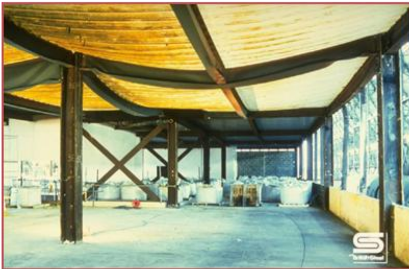
Figure 5: Composite slab in large deflection after Cardington fire tests (Kirby 1998)
