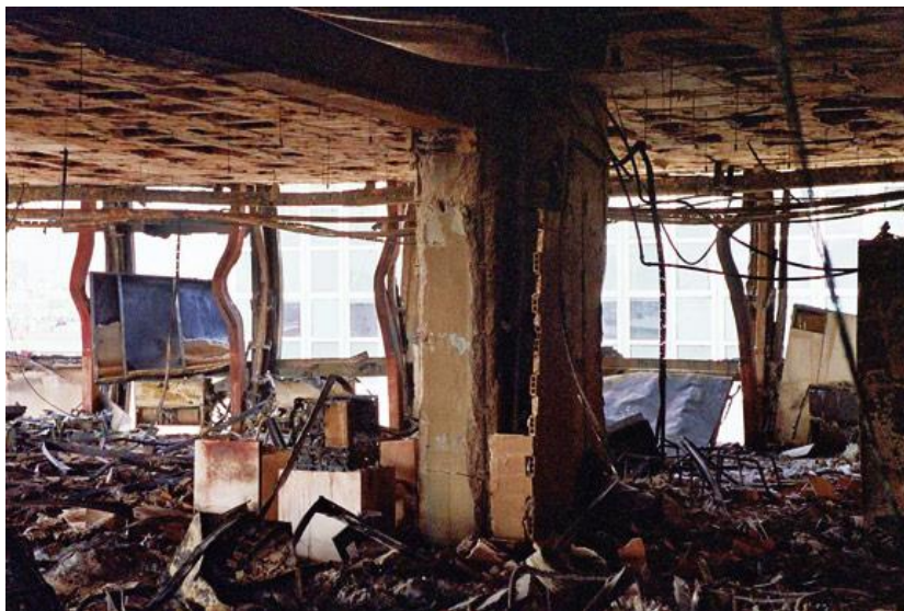
Figure 4: Columns buckling of the 9th floor, Windsor Tower (Pope 2006)
