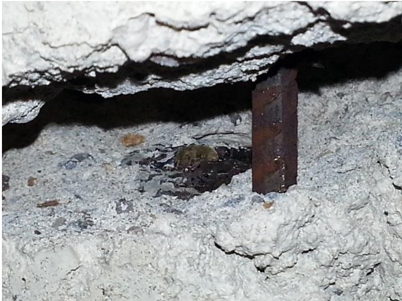
Figure 90: Rebar-bolt weld detachment that occurred during testing the second specimen
