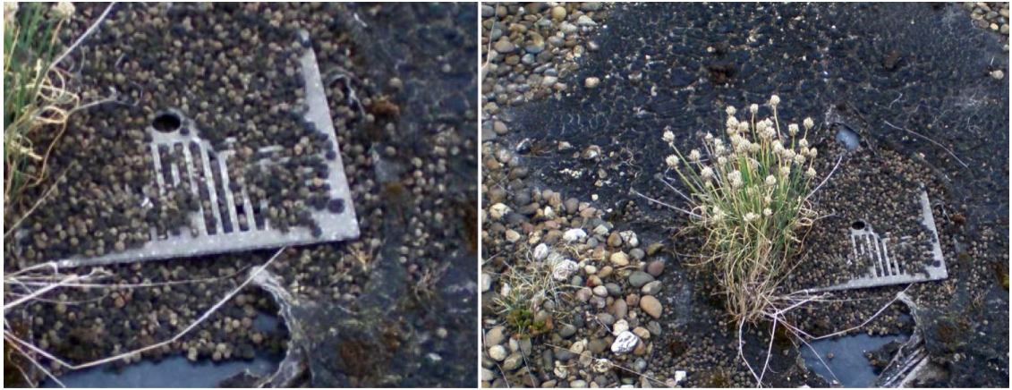
Figure 4.2. Blocked drains on VB A2 led to the re-positioning of the lightweight (LECA) substrate component; several areas have been scoured to expose the waterproofing.
