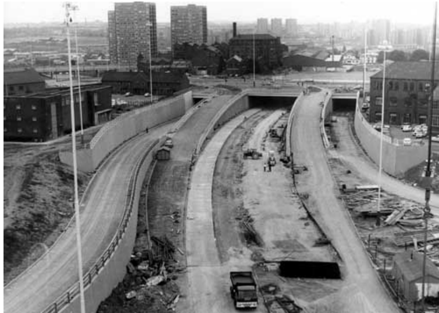
Fig. 3.5 The inner ring road under construction at its junction with Clay Pitt Lane on the eastern side of the city centre. Three newly constructed tower blocks in Little London are visible beyond the bridge. Some old industrial buildings remain in what was a densely populated residential area. Undated image from the late 1960s or early 1970s. [Leeds Library and Information Services, http://www.leodis.net/ , accessed 17 February 2015]
