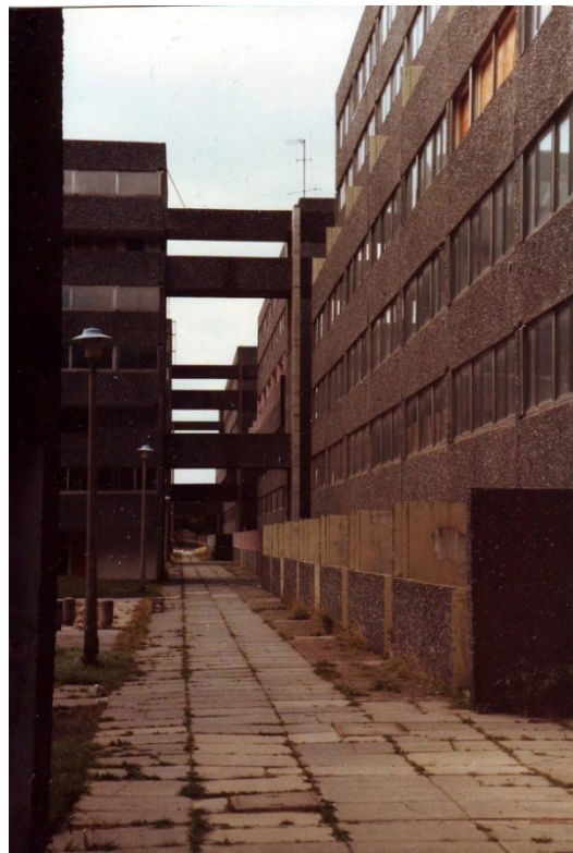
Fig. 1.6 An internal courtyard within the estate. Undated image. [Clifford Stead, flickr, https://www.flickr.com/photos/cliffordstead/albums , accessed 21 September 2015]
