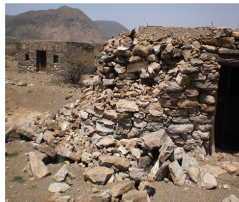
Fig. 5 Building damaged by the 31 March 2011 earthquake. Better constructed walls, as seen in the background, sustained only cracking
