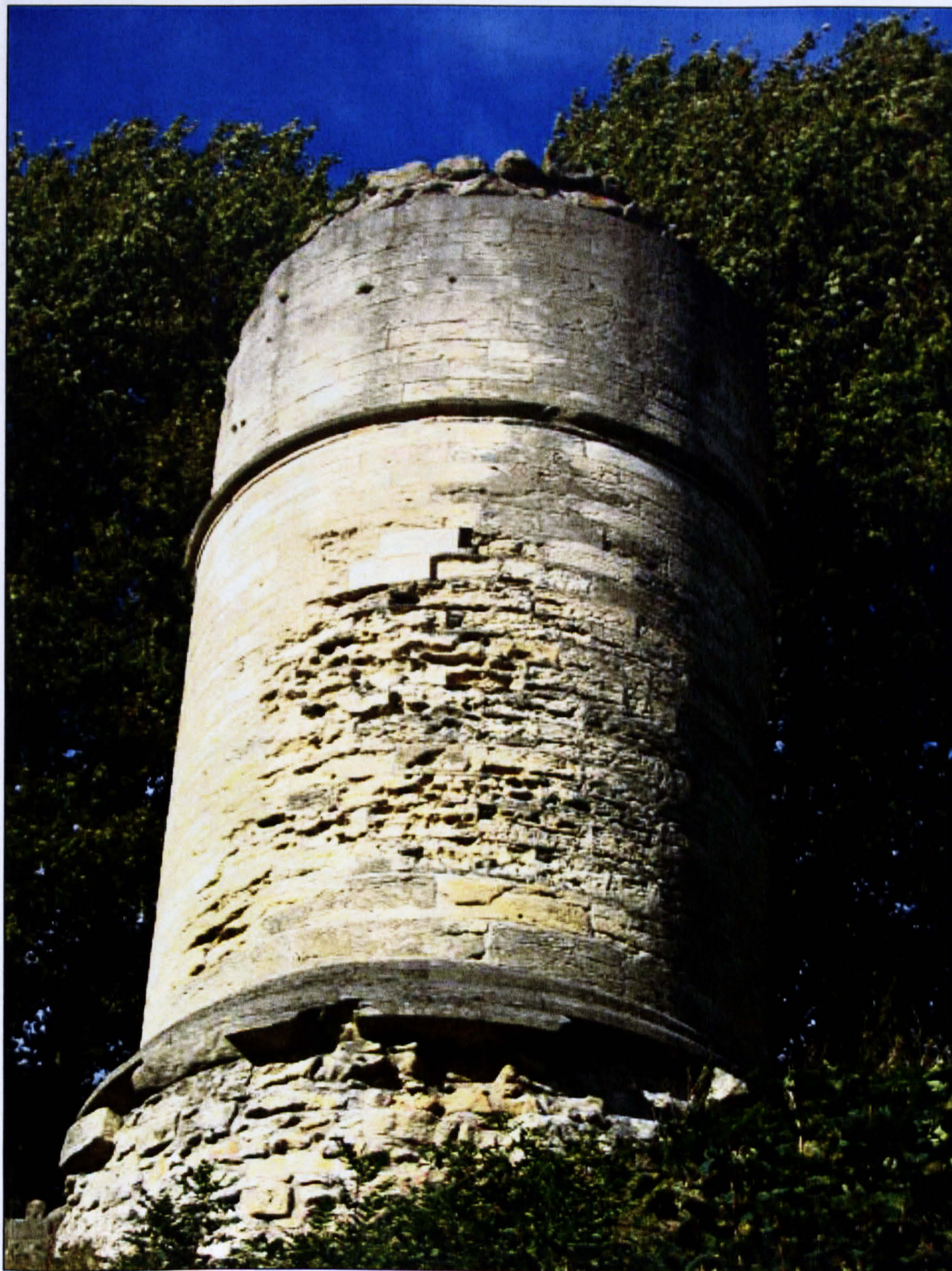
Figure 4.15 T1 showing weathering damage and replaced ashlar.
