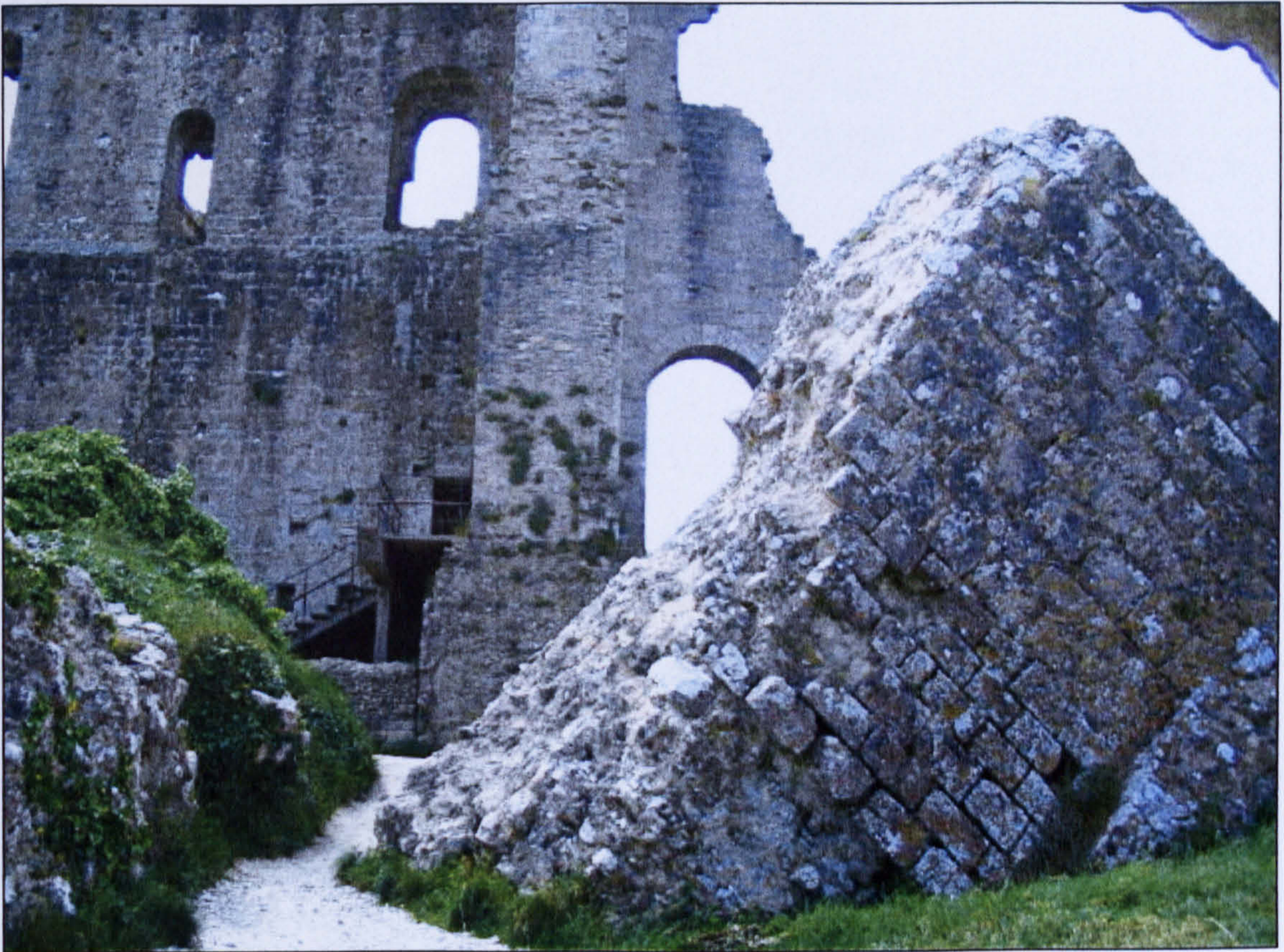
Figure 5.33 Leaning wall, west approach (View 2).
