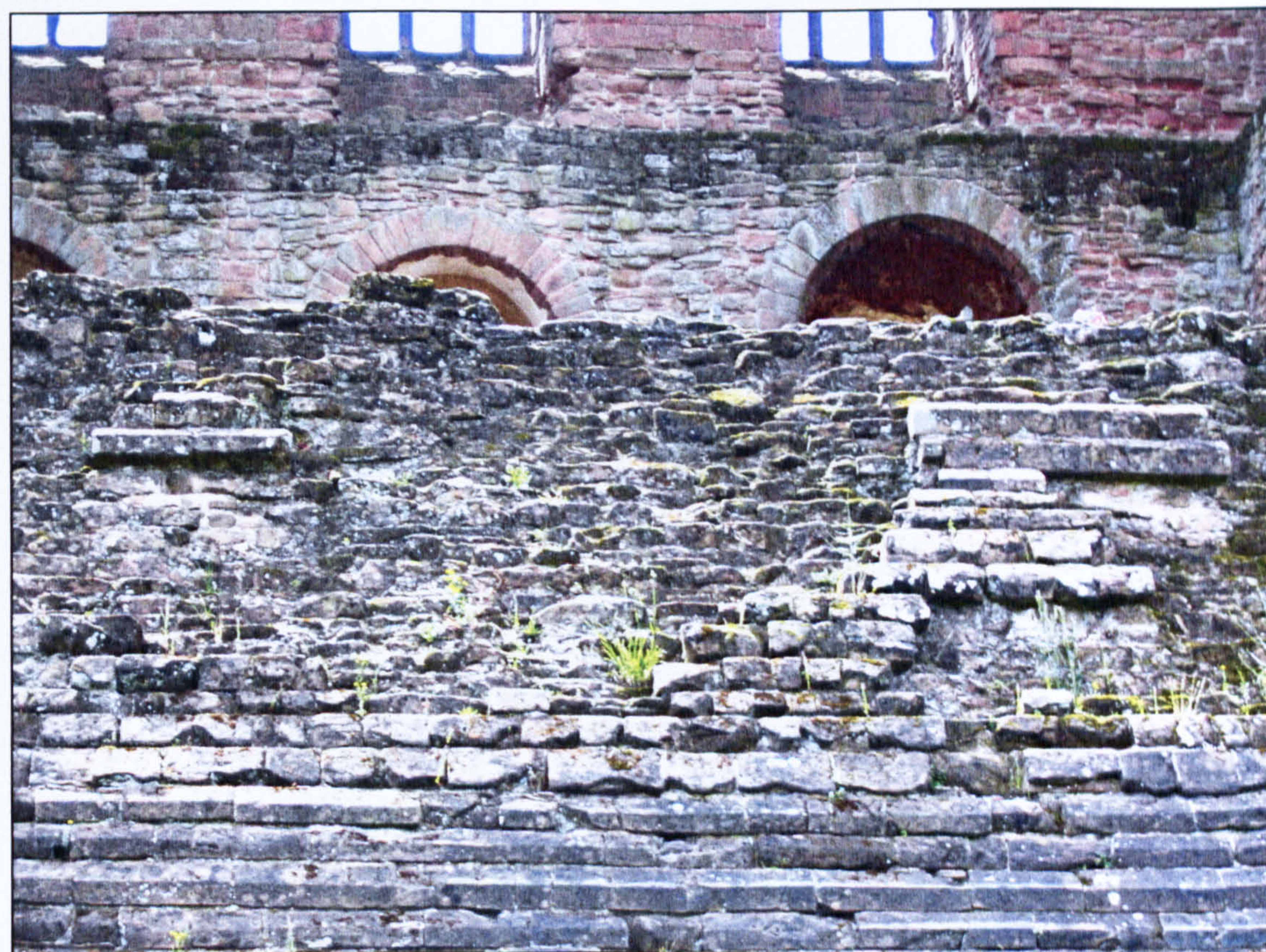
Figure 6.21 Close-up of the damaged stonework of the upper plinth of the north side of the keep.
