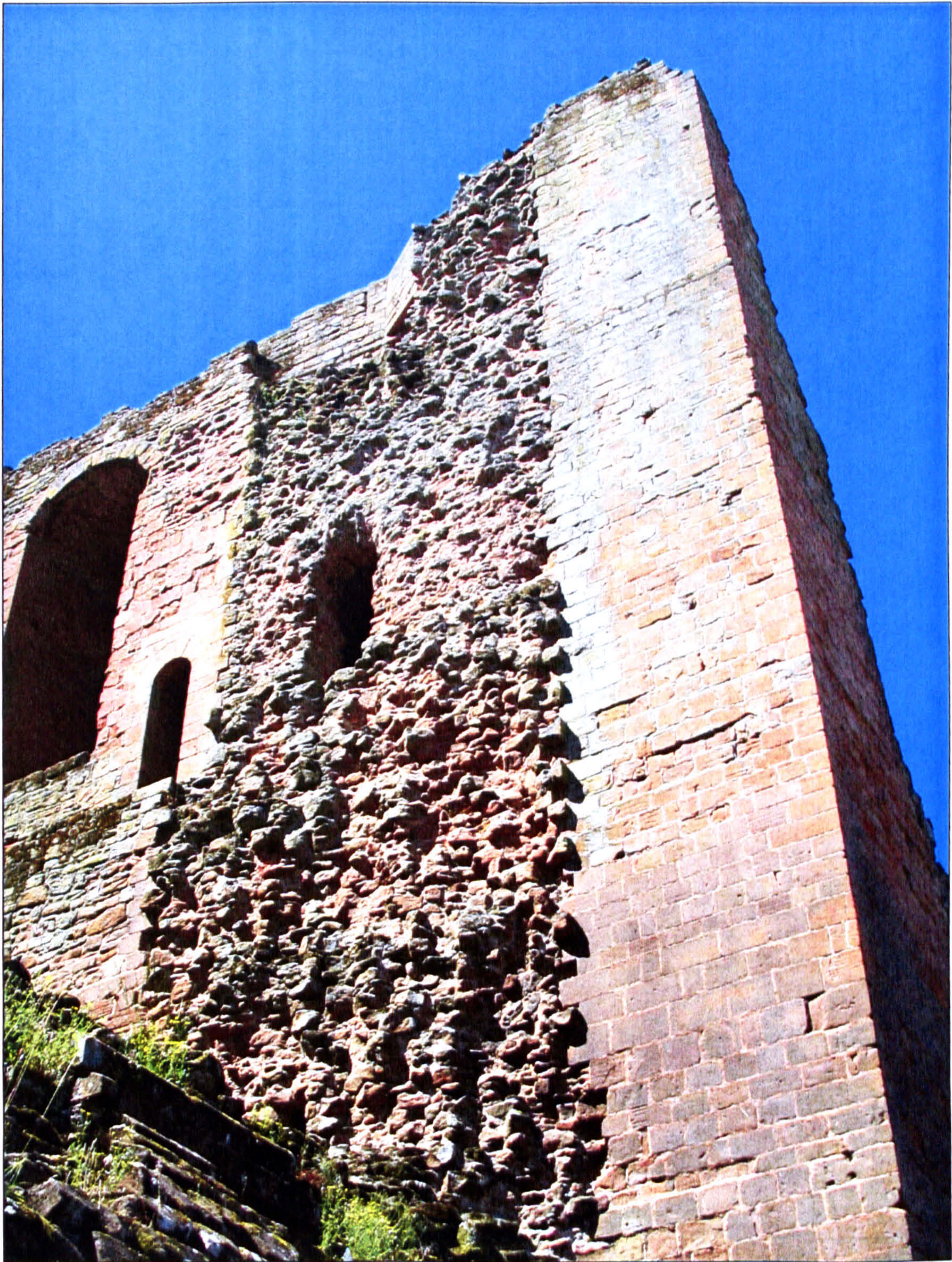
Figure 6.31 A view of the northwest corner and its exposed rubble core, showing the difference in construction quality between the upper and lower sections of the wall.
