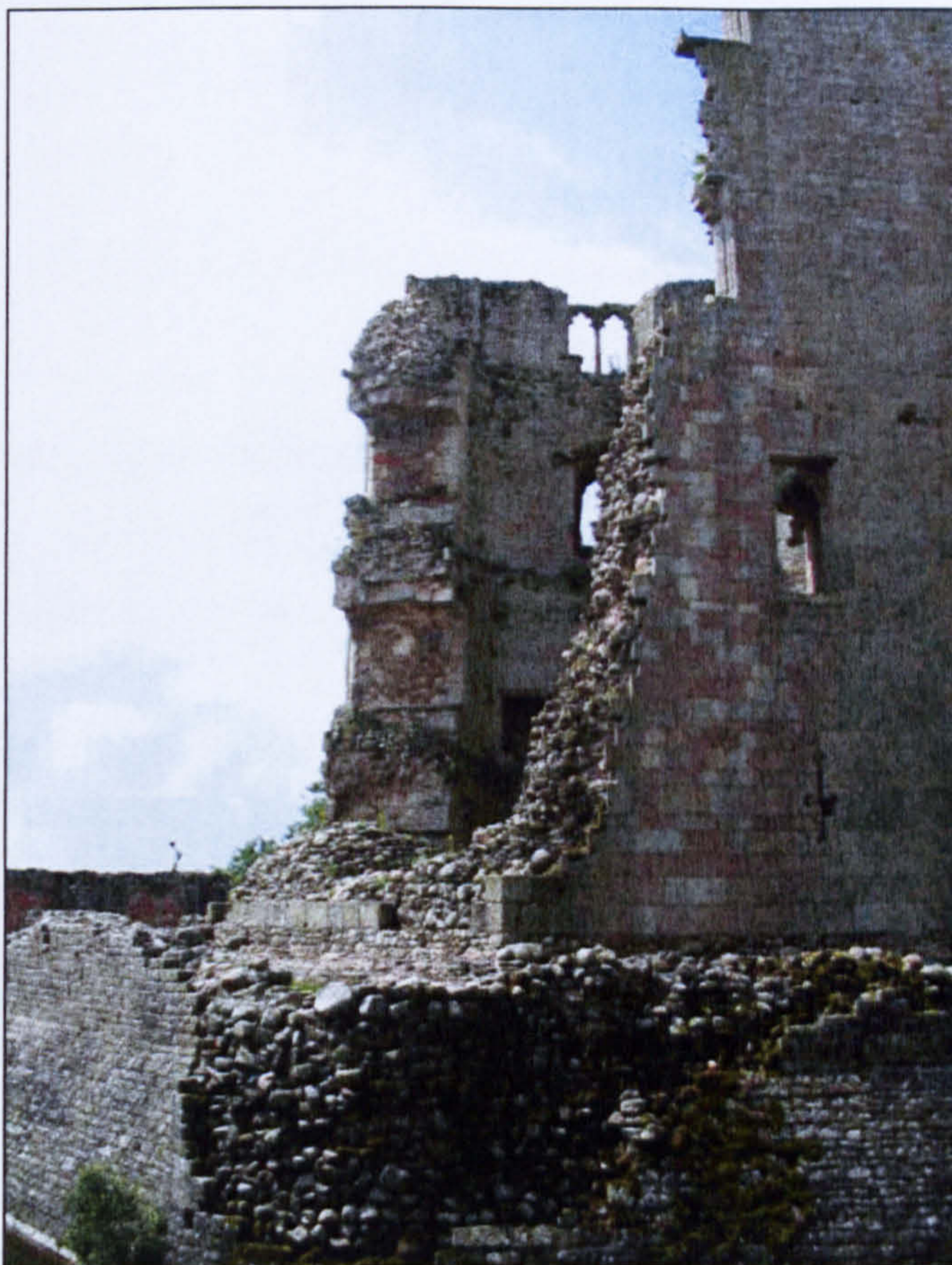
Figure 5.47 The damage pattern of the northeast wall, showing much higher placed windows.
