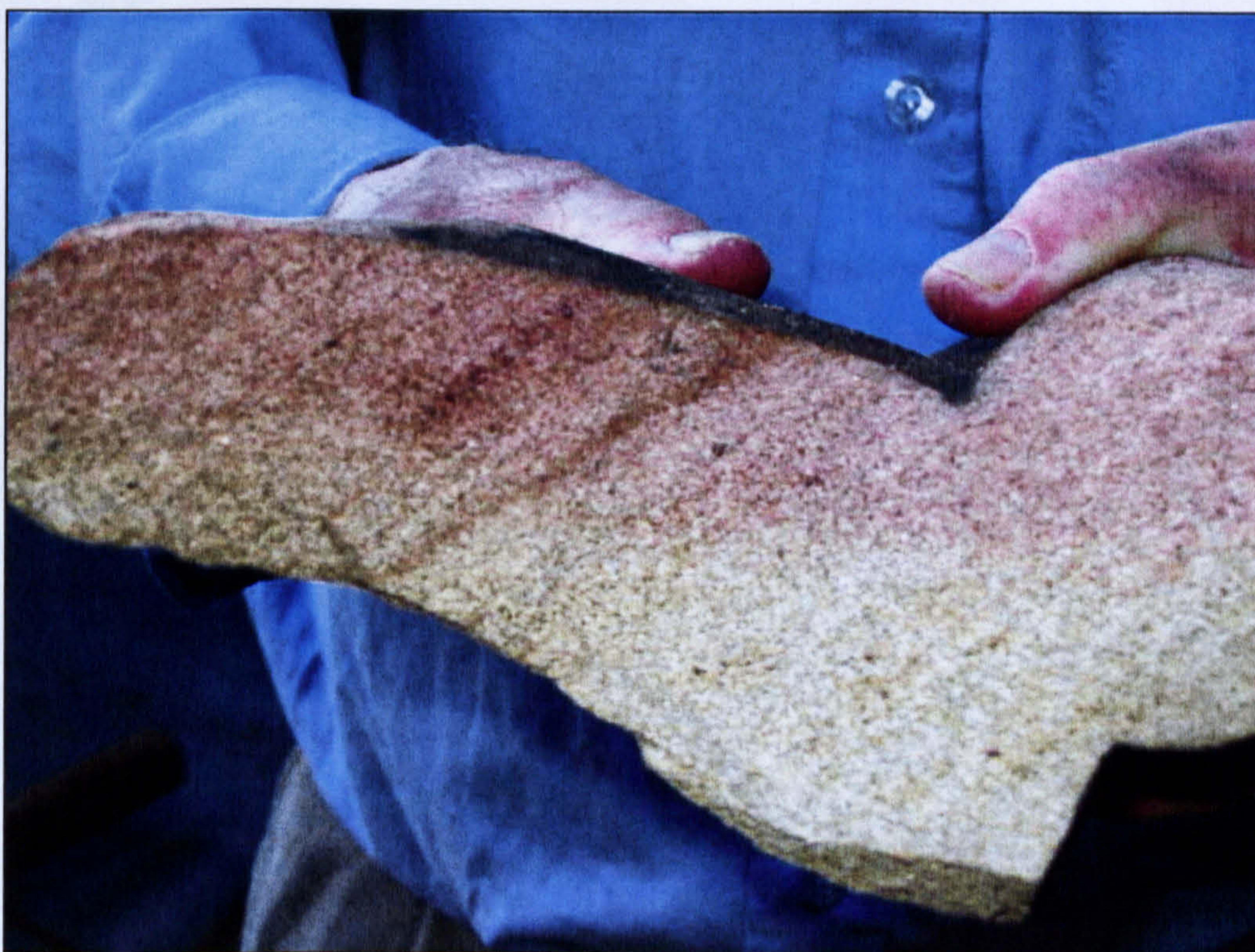
Figure 3.7 Fire damaged stone from Allerton Castle, showing signs of surface reddening.
