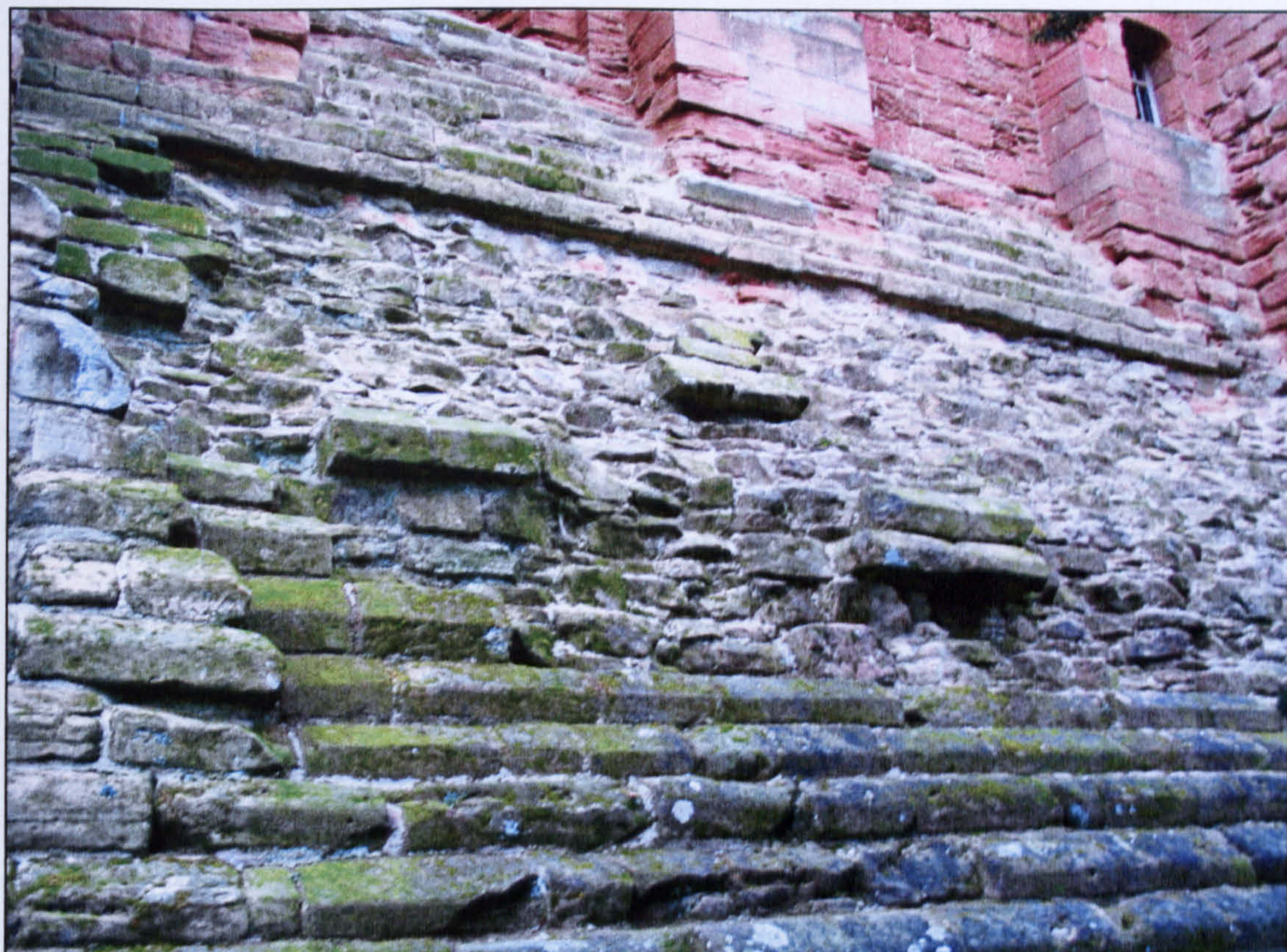
Figure 6.27 Close-up of the plinth on the east elevation, showing considerable damage to its upper courses.
