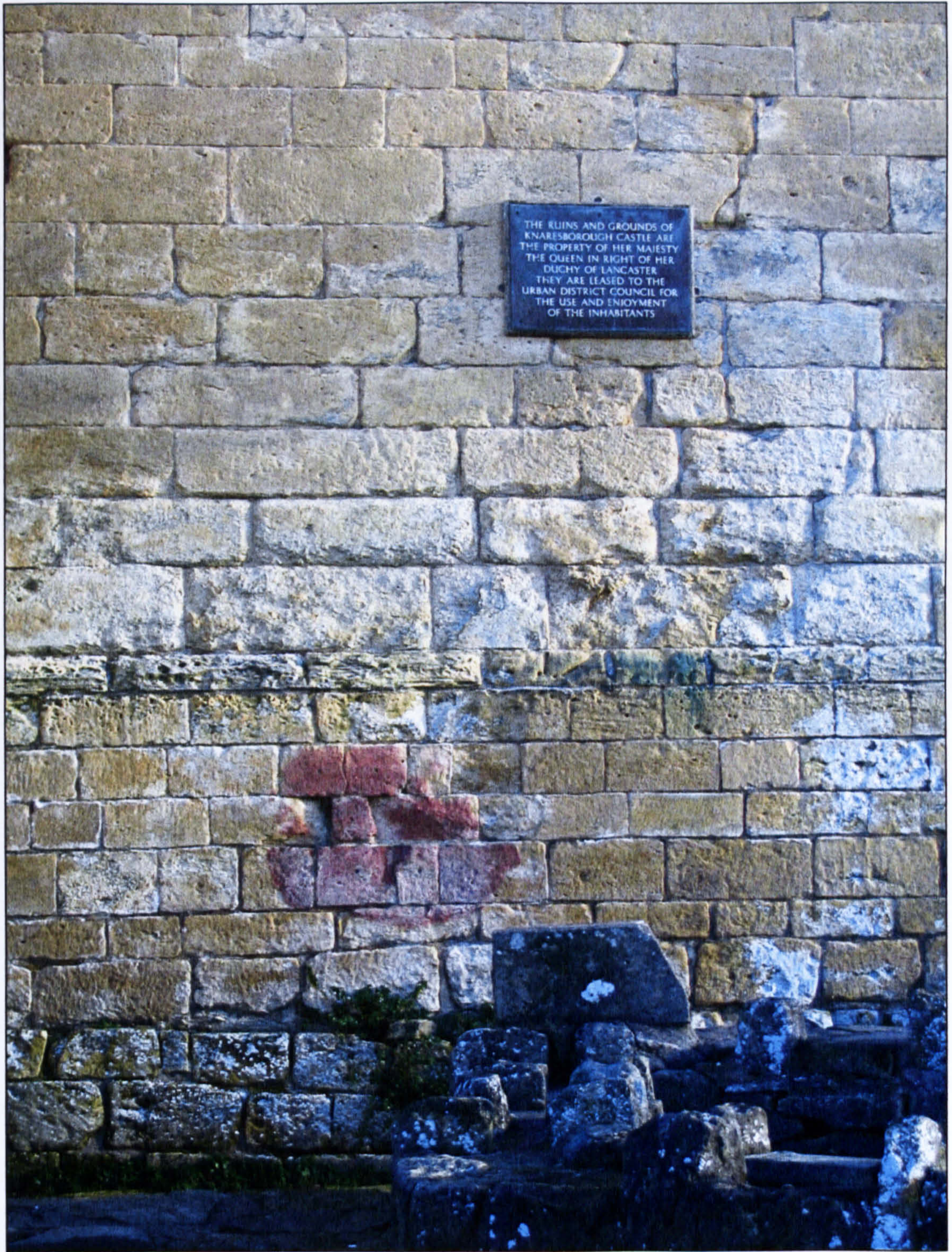
Figure 3.12 West side of keep, showing a small fire damage pattern low to the ground (Knaresborough Castle).
