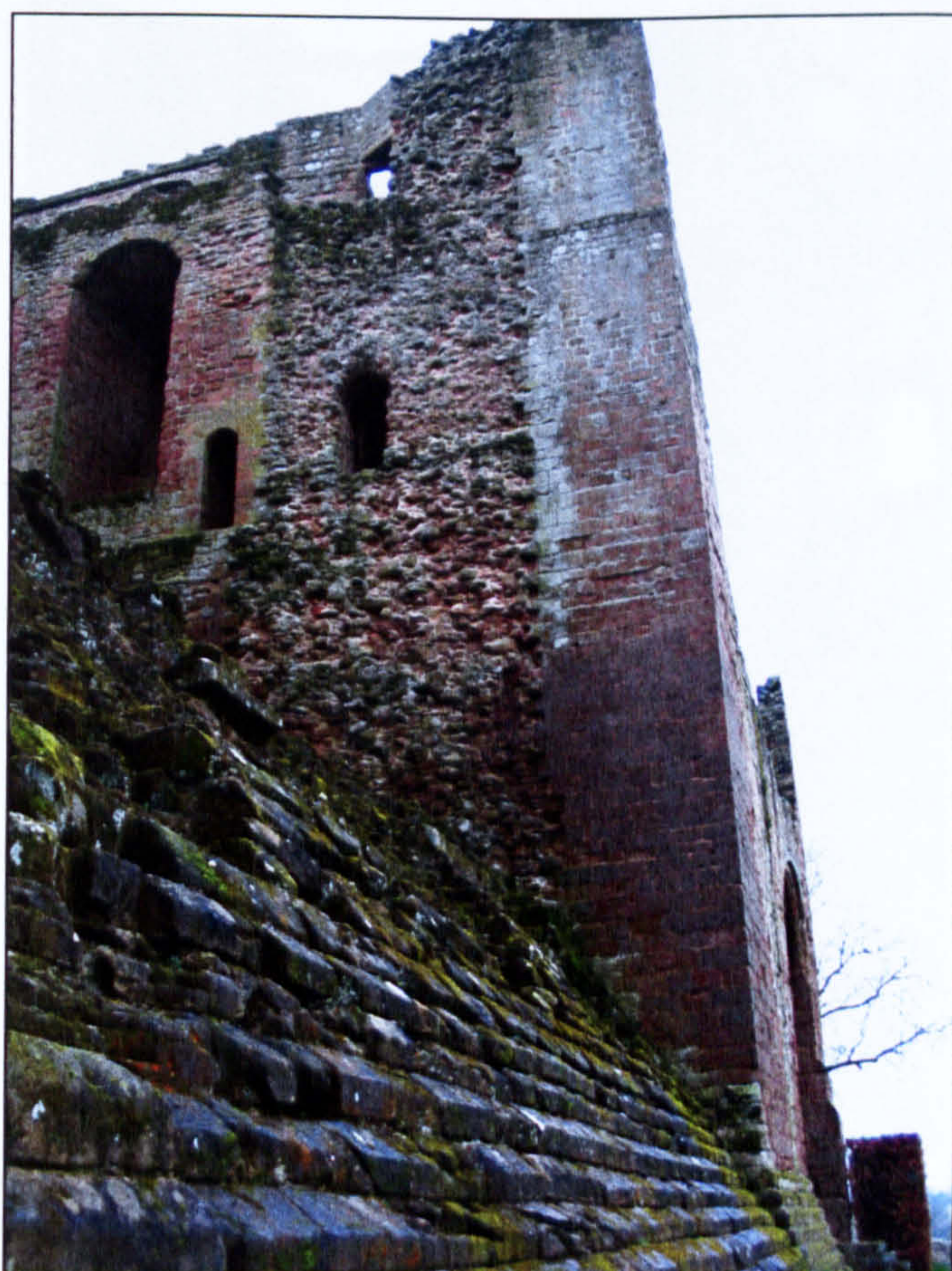
Figure 6.23 The northwest corner, showing the former point of connection with the north wall.
