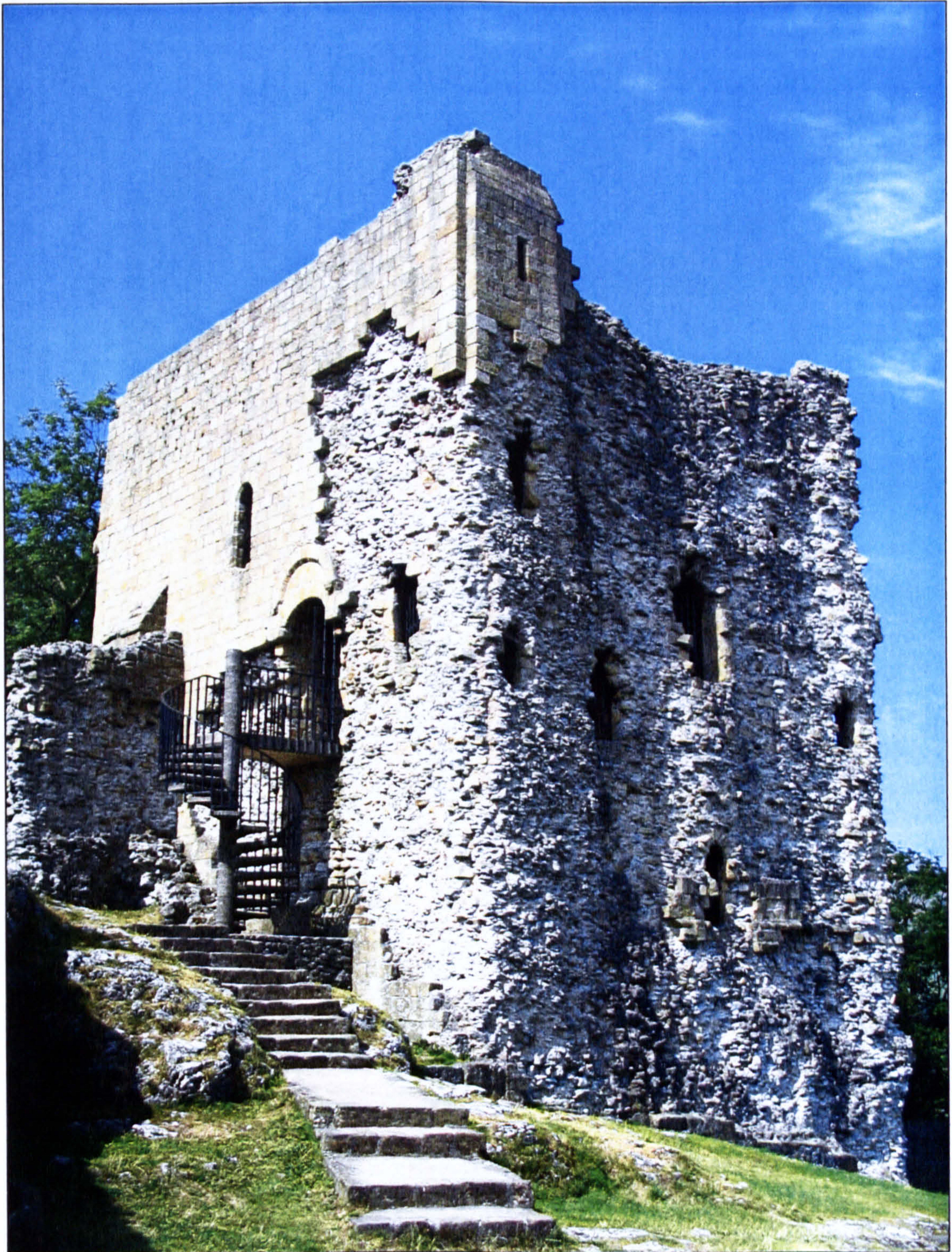
Figure 4.34 Peveril Castle Keep, looking south, showing the scale of secondary damage.
