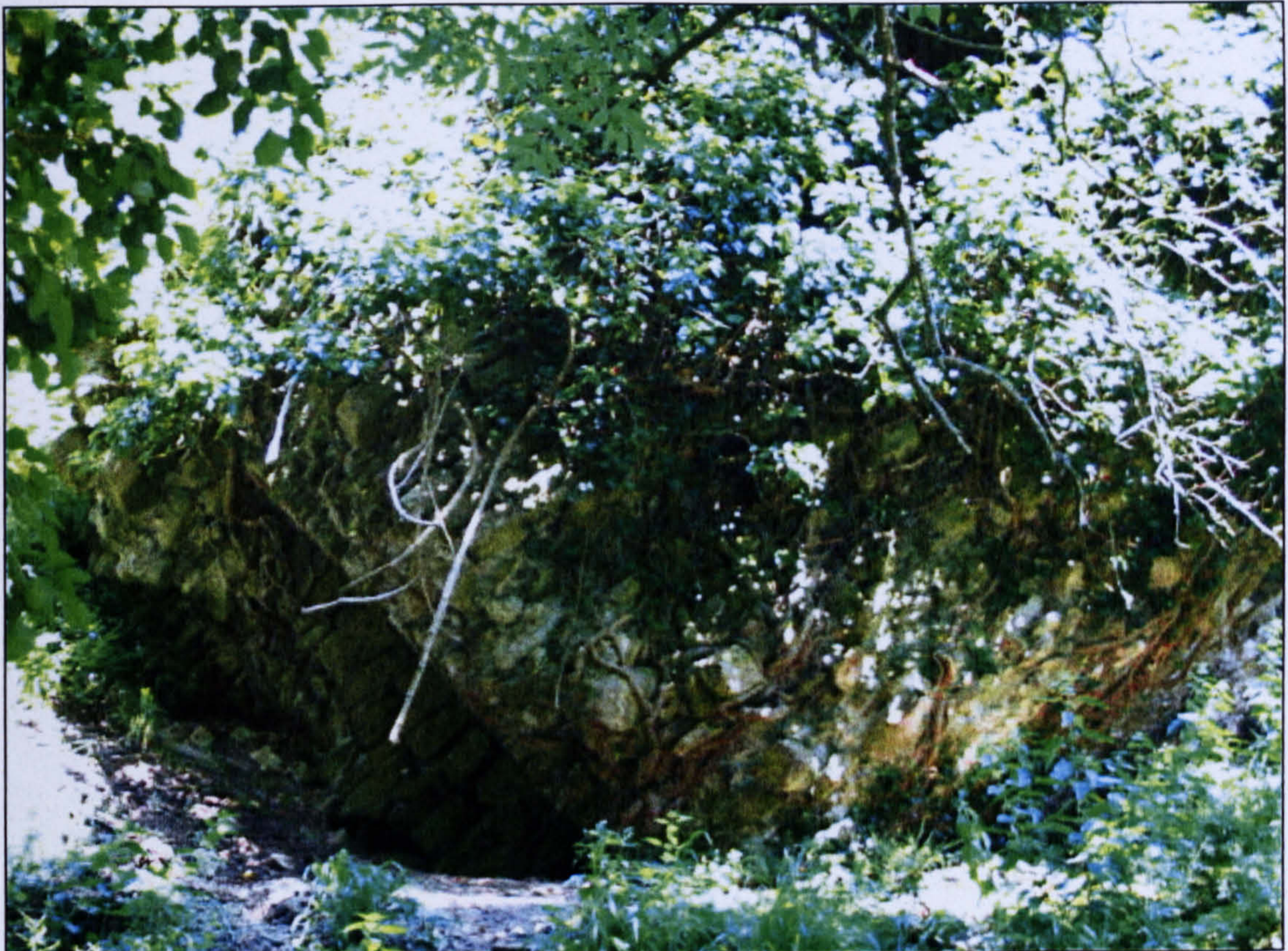
Figure 5.14 Masonry debris from southwest curtain, located at bottom of hillside.
