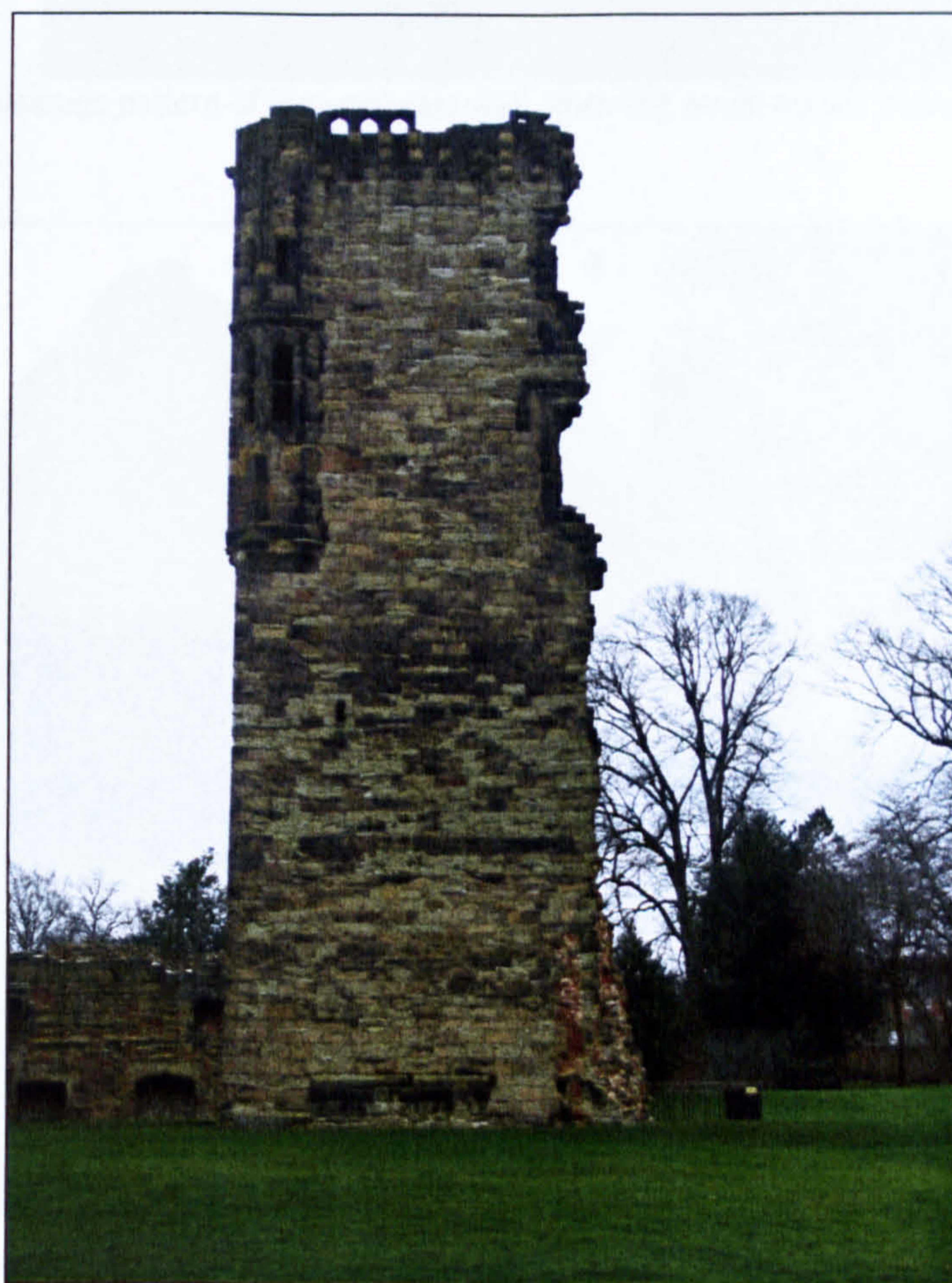
Figure 5.46 A profile view of Hastings Tower at Ashby de la Zouch (Leicestershire), showing a vertical damage pattern and the bisection of two upper windows.
