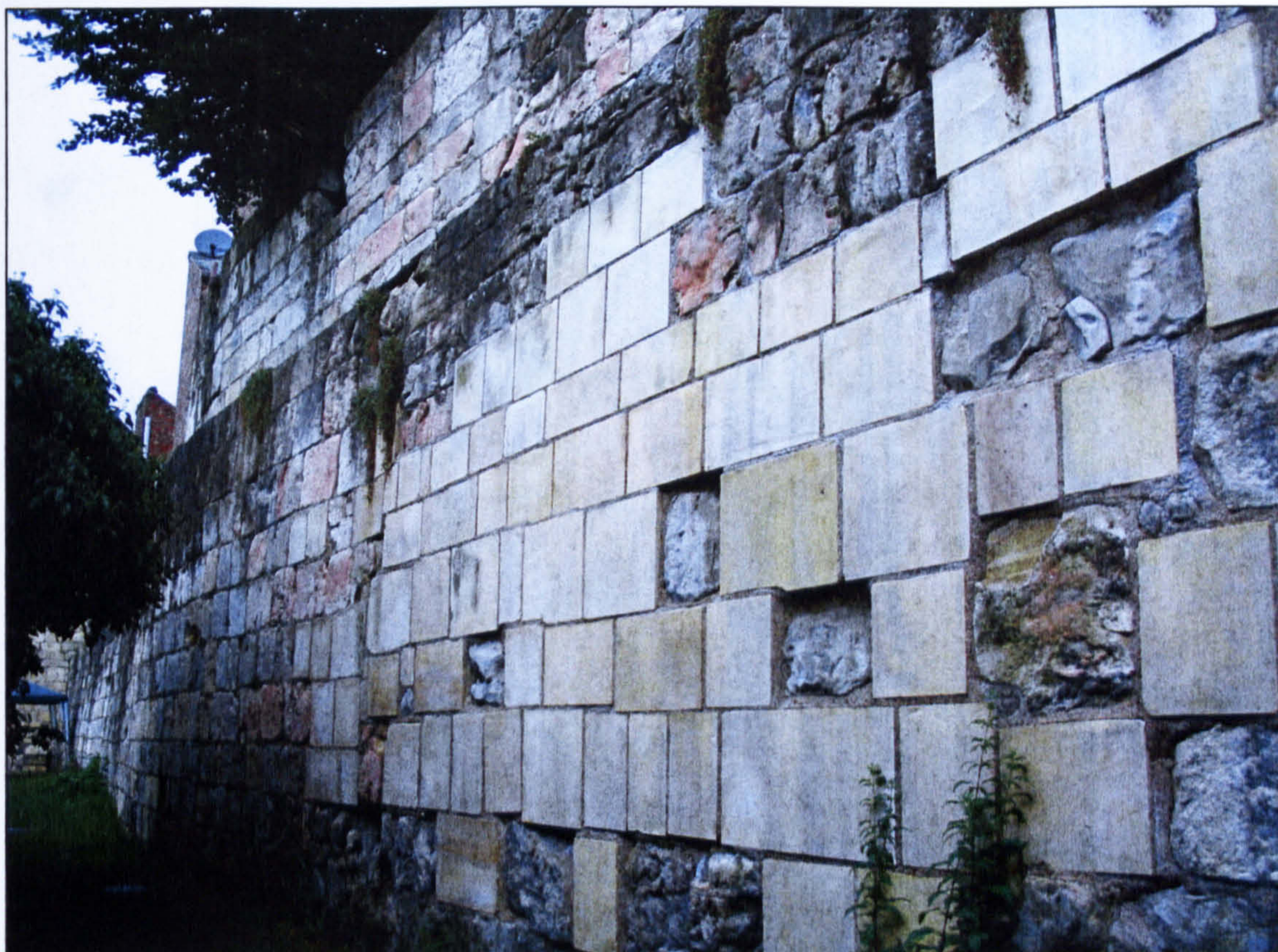
Figure 3.2 Wall at St. Mary's Abbey (York) showing fire damage in situ , as well as new ashlar blocks.
