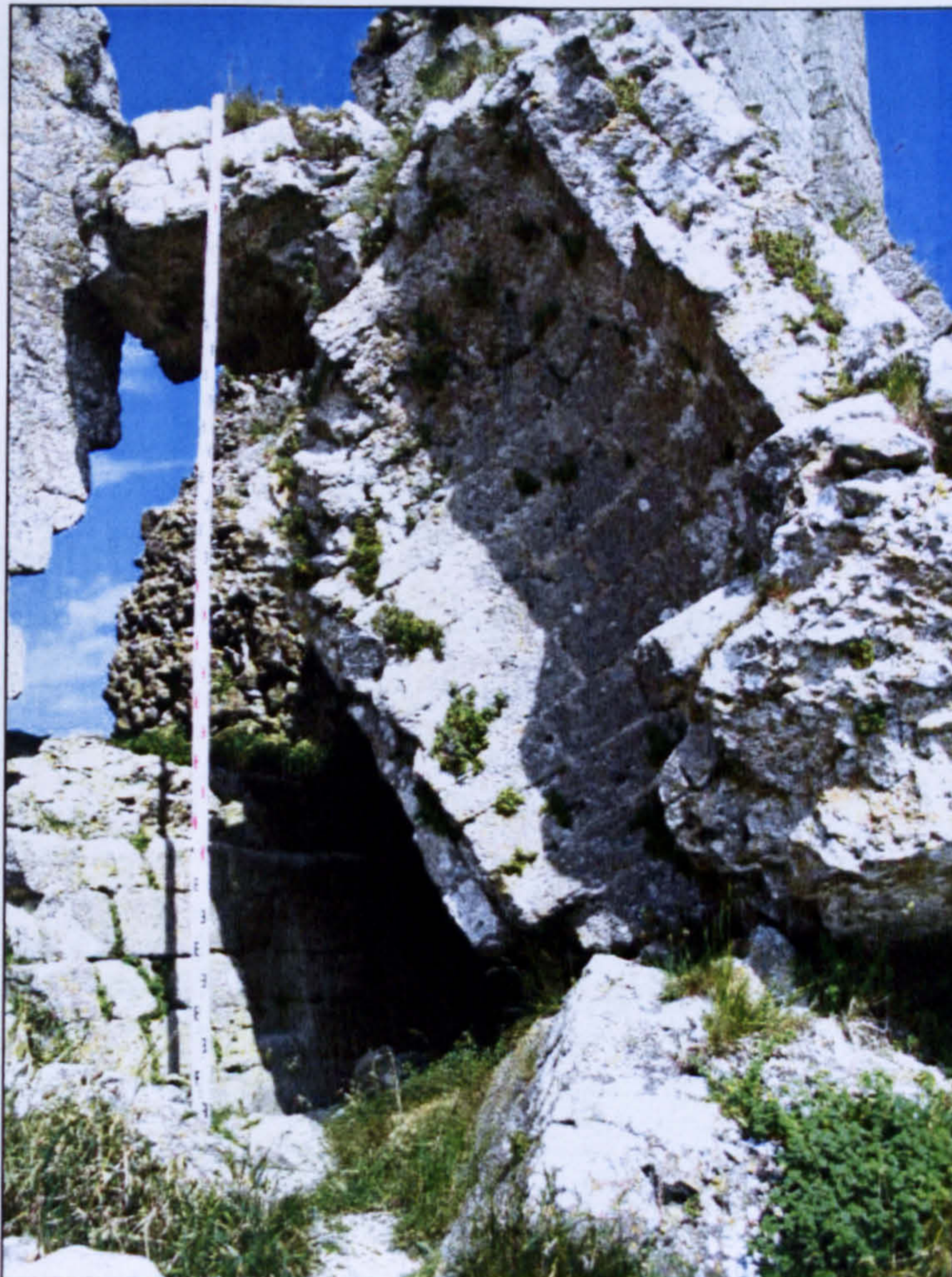
Figure 5.28 Close-up of wall collapse on the exterior side of the east wall.
