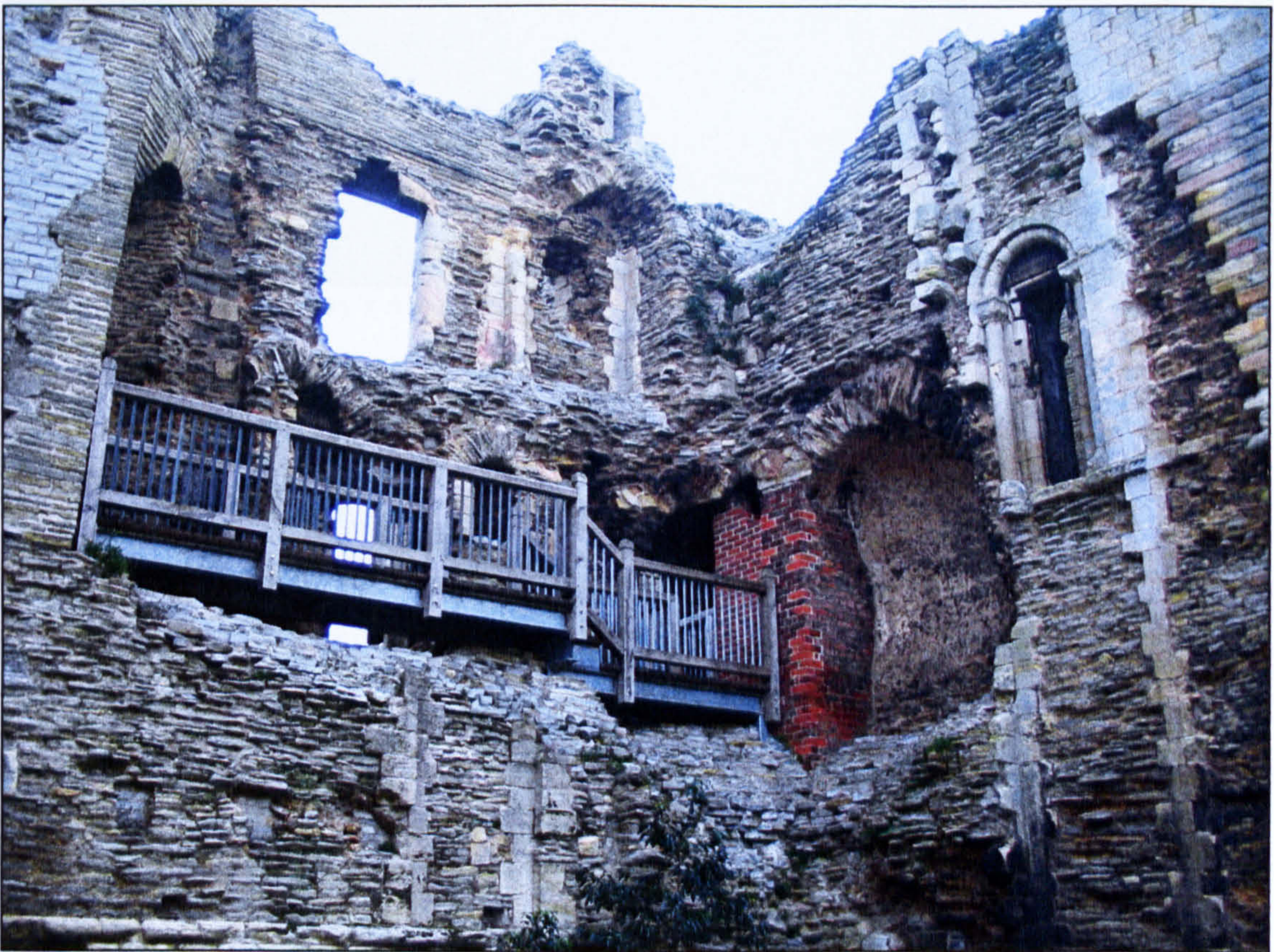
Figure 3.1 Explosion damage pattern in Gatehouse at Newark Castle (Nottinghamshire) as defined by its cratered out shape and highlighted by extensive Victorian restoration.
