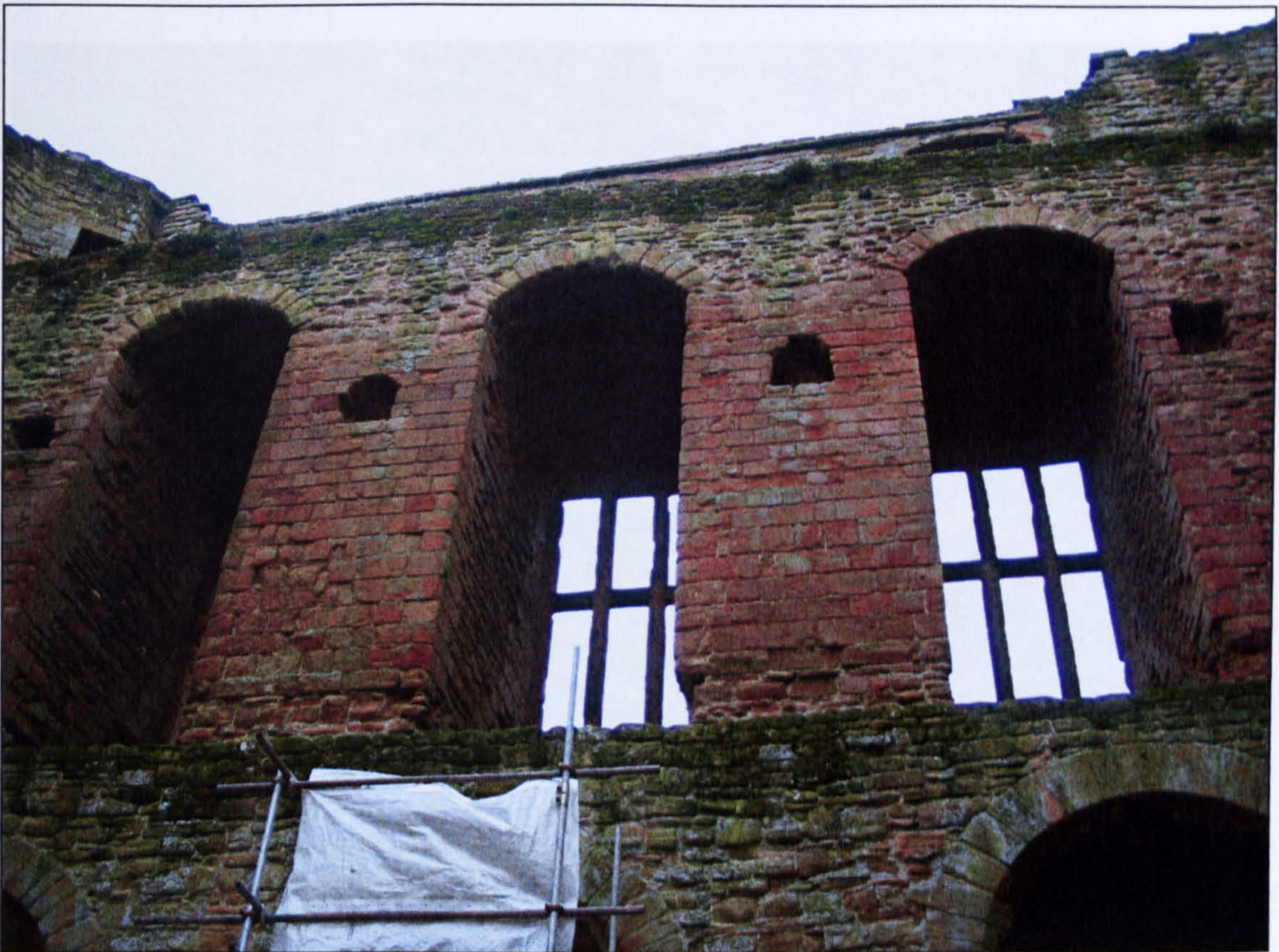
Figure 6.25 The upper half of the internal, south wall of the keep, showing intact and undamaged joist holes.
