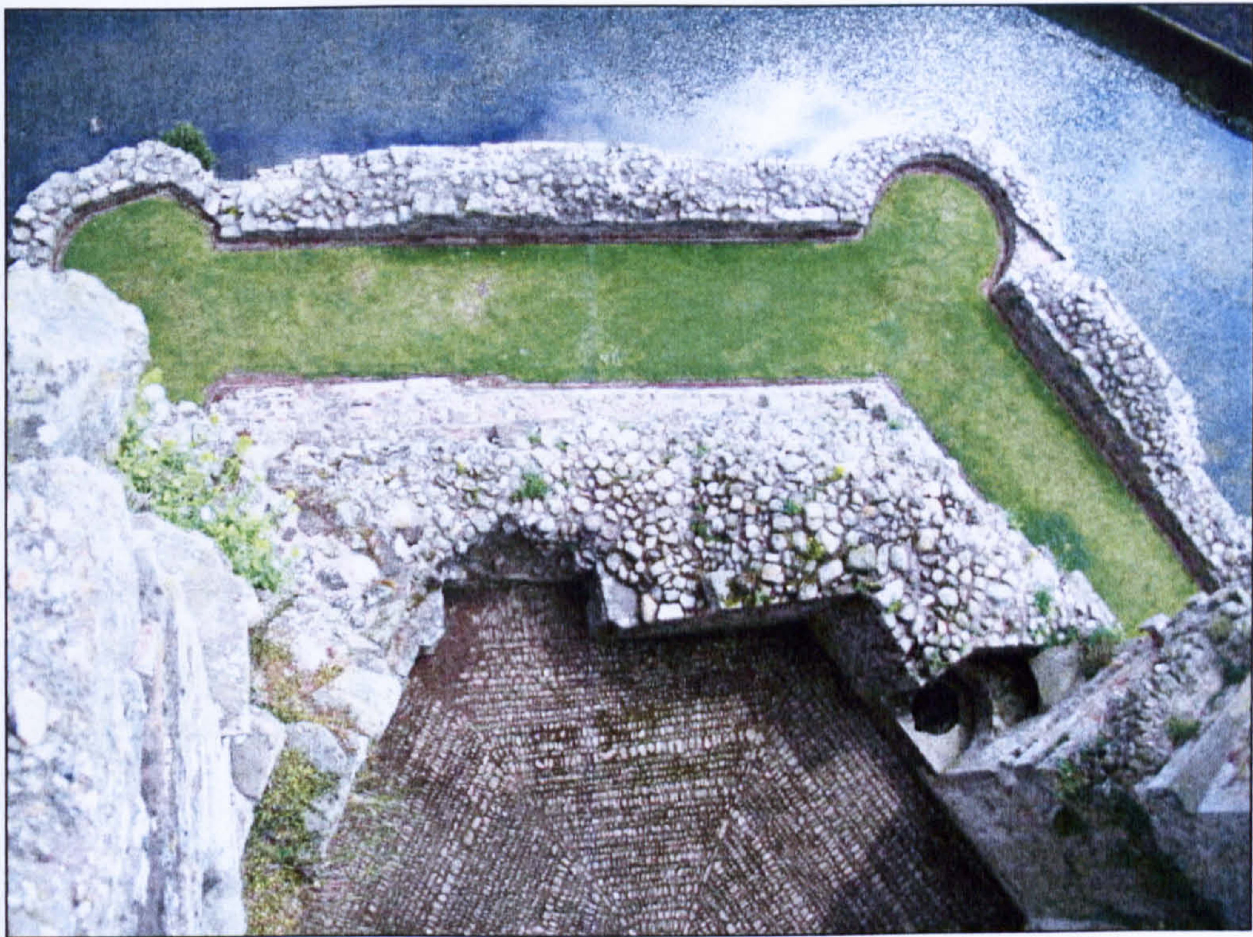
Figure 5.43 The damaged wall viewed from above, showing the variations in wall thickness.
