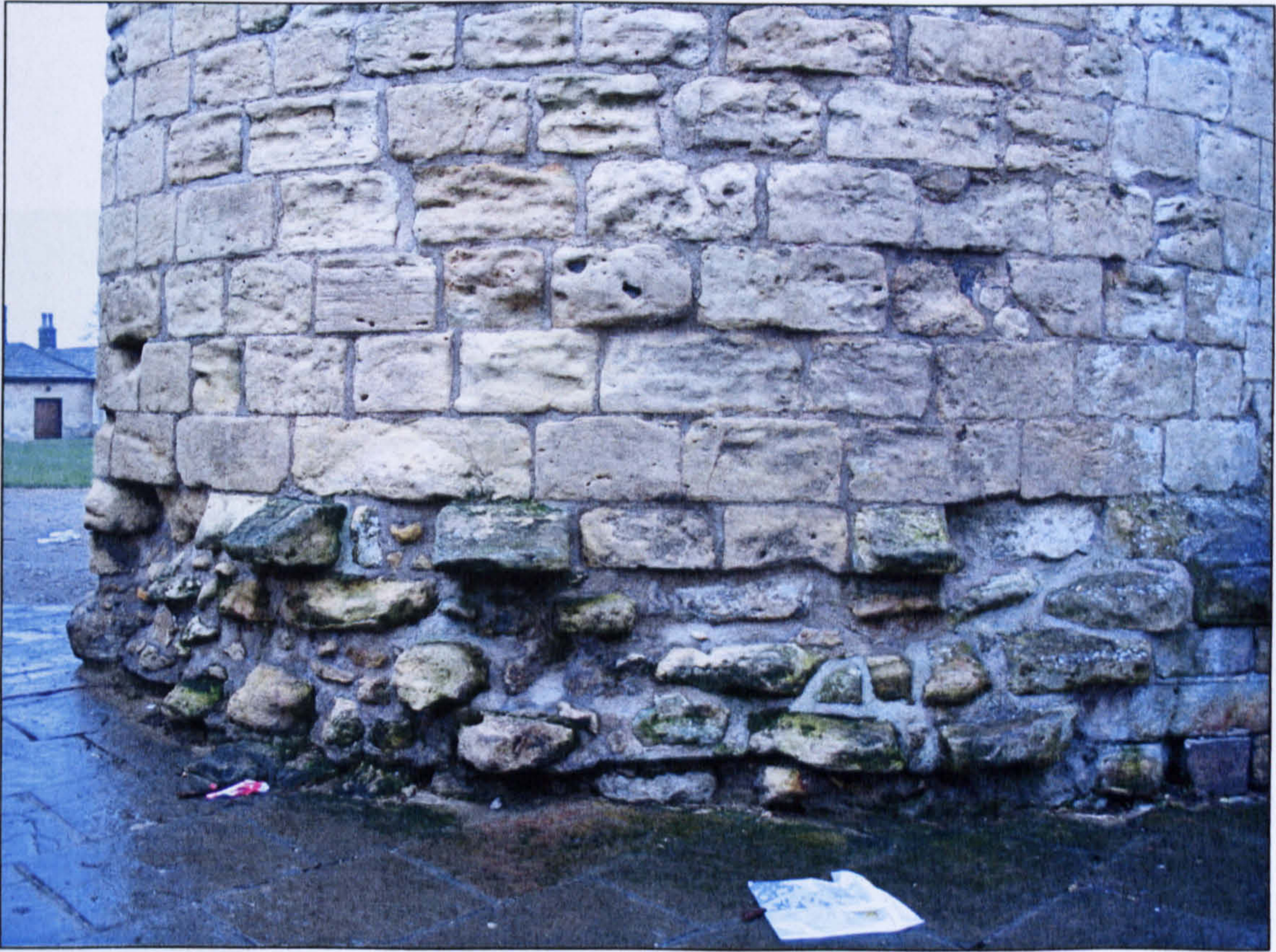
Figure 4.9 Close-up of base of G2.
