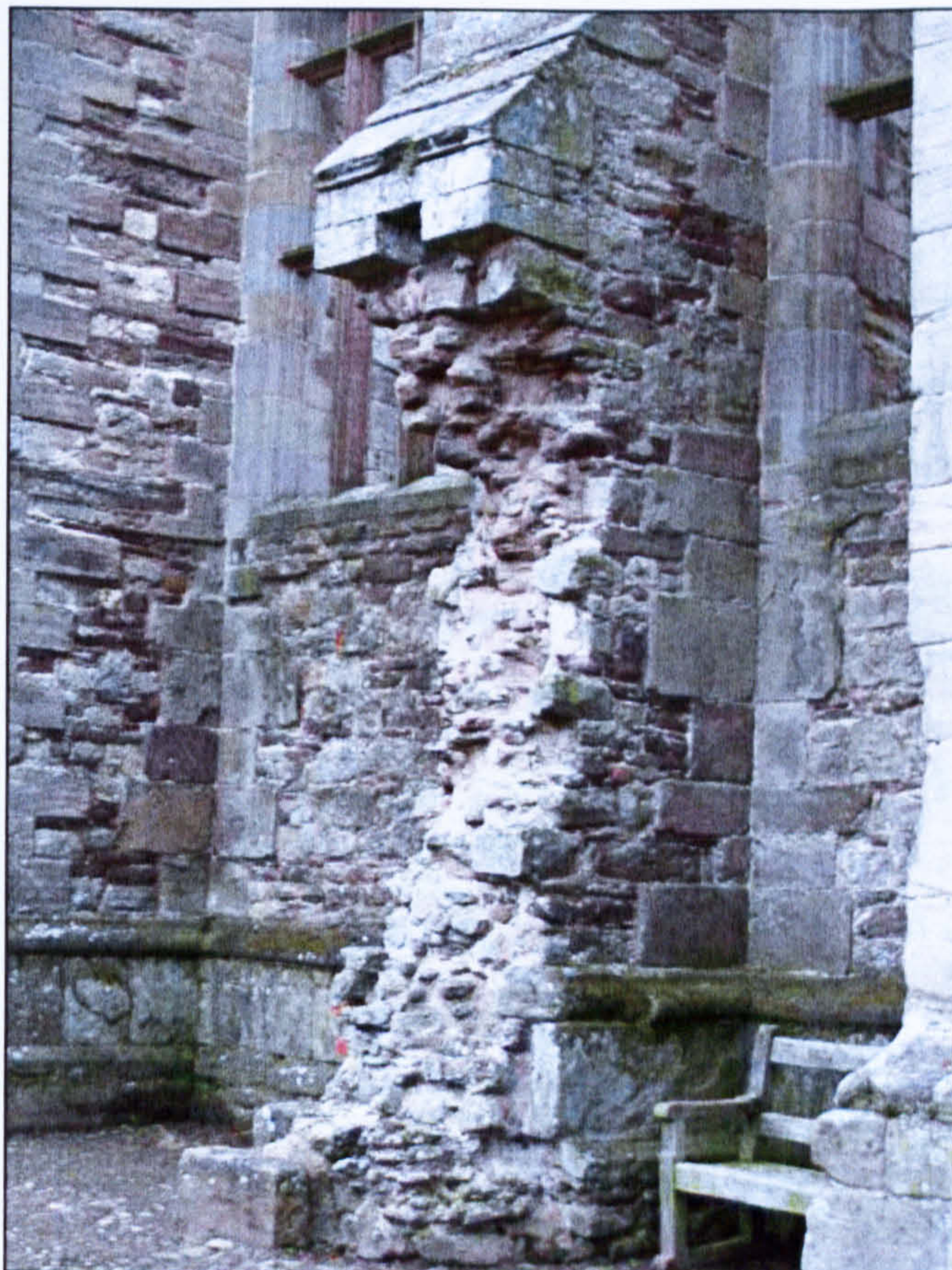
Figure 4.56 Close-up of secondary damage in Pitched Stone Court at Raglan Castle (Wales).
