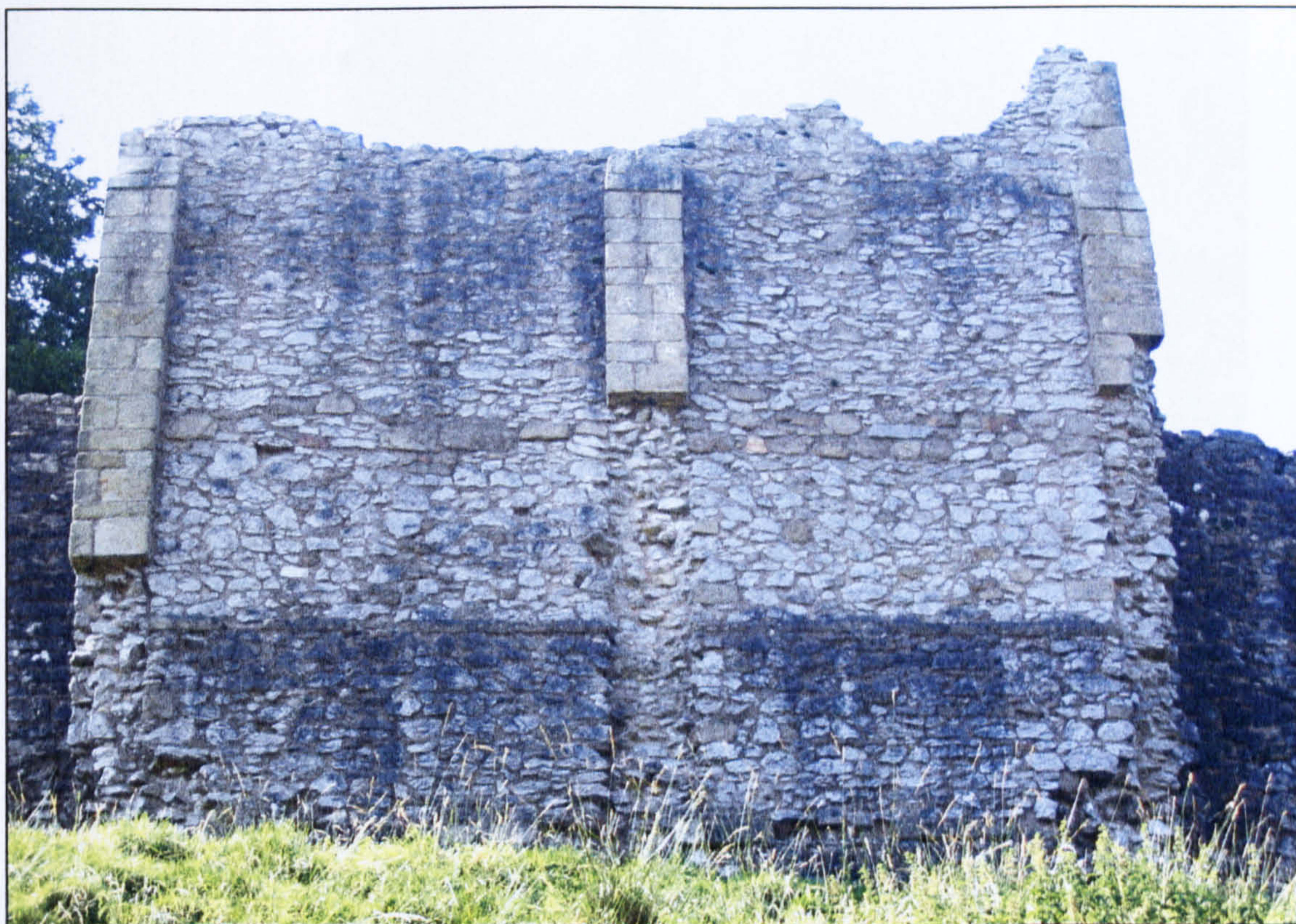
Figure 4.38 Secondary damage at Peveril Castle in the form of removed Quoins.
