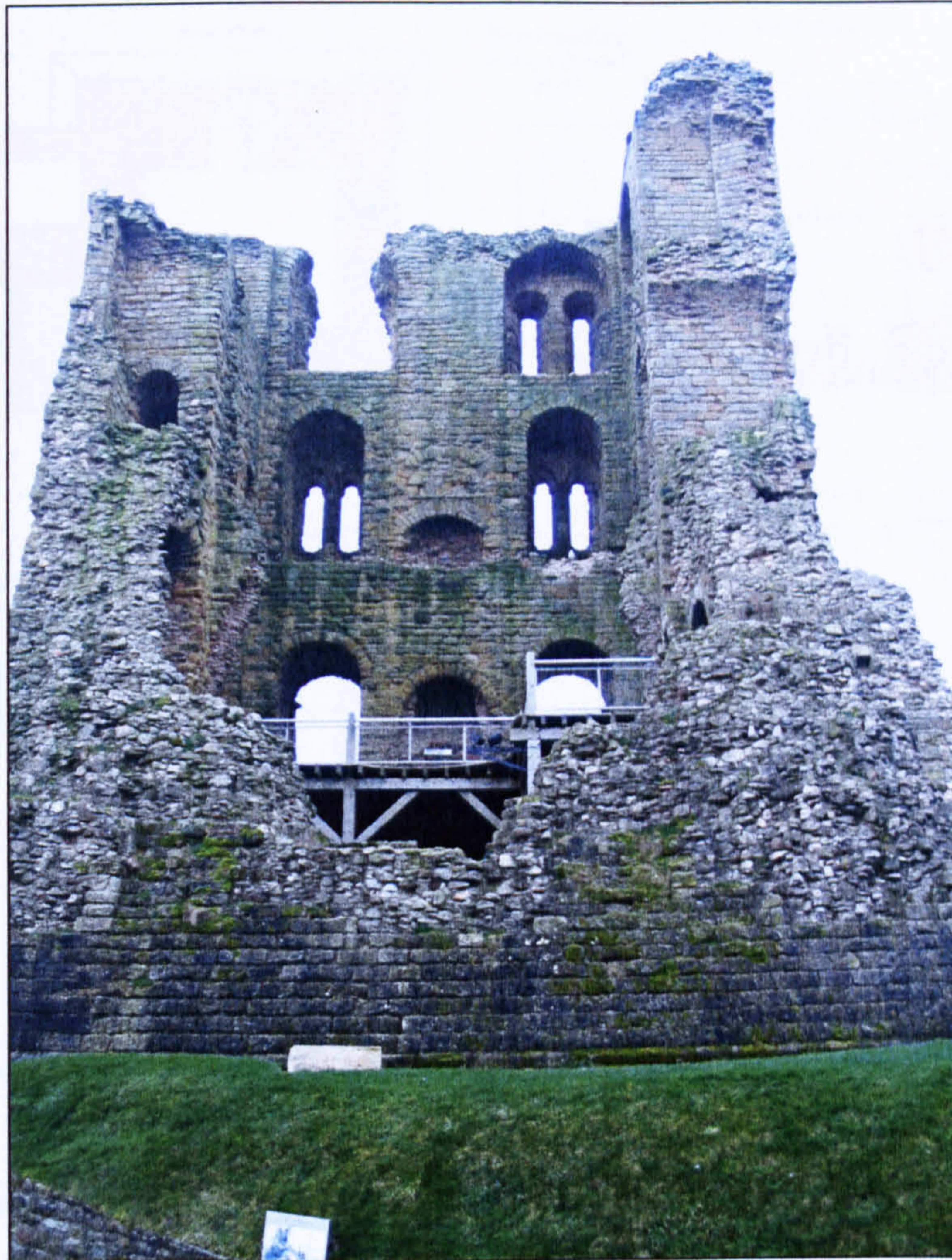
Figure 5.67 The damaged west wall of Scarborough Castle Keep, looking east.
