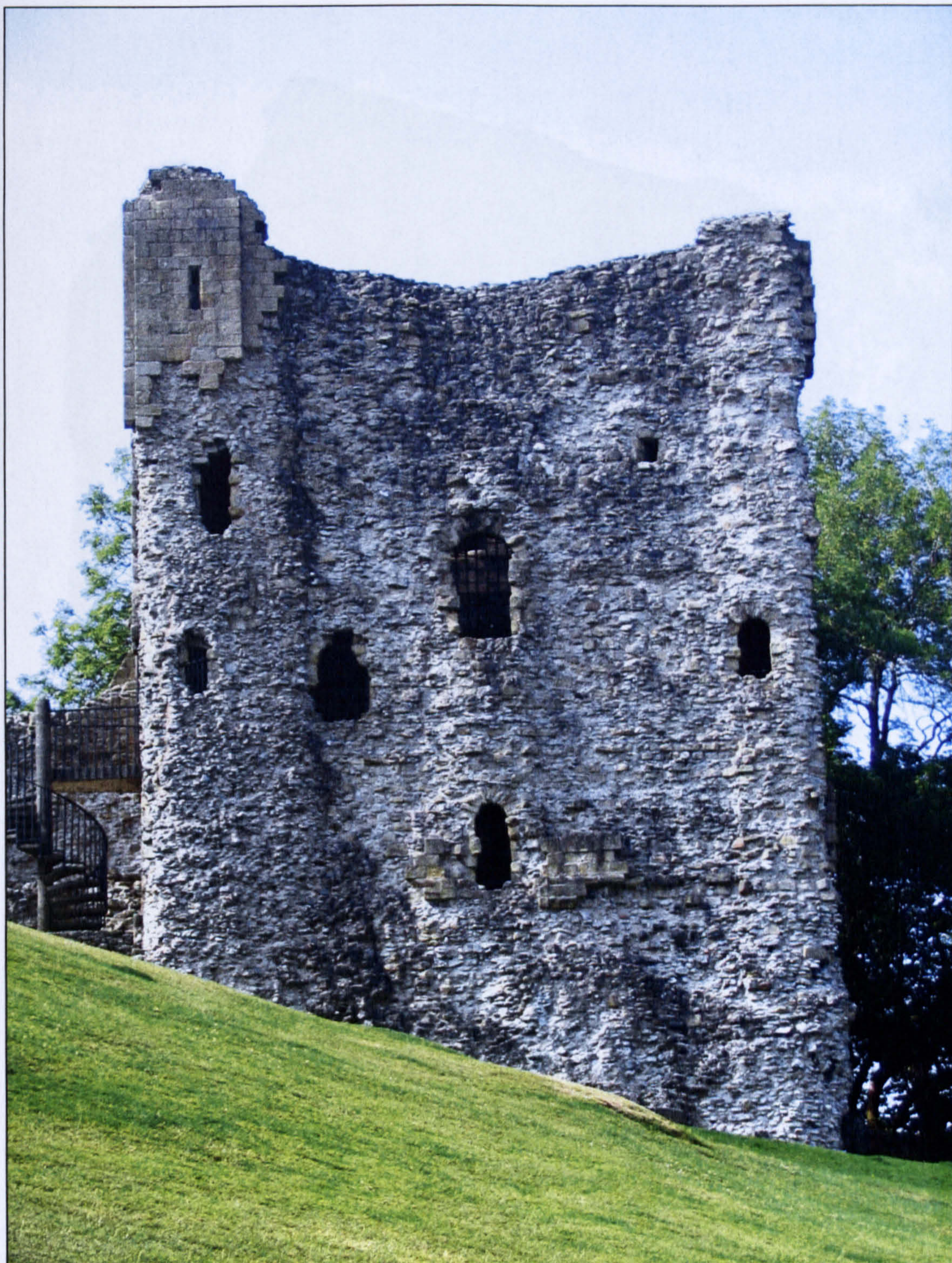
Figure 4.35 Peveril Castle Keep, looking southeast, showing the scale of secondary damage.
