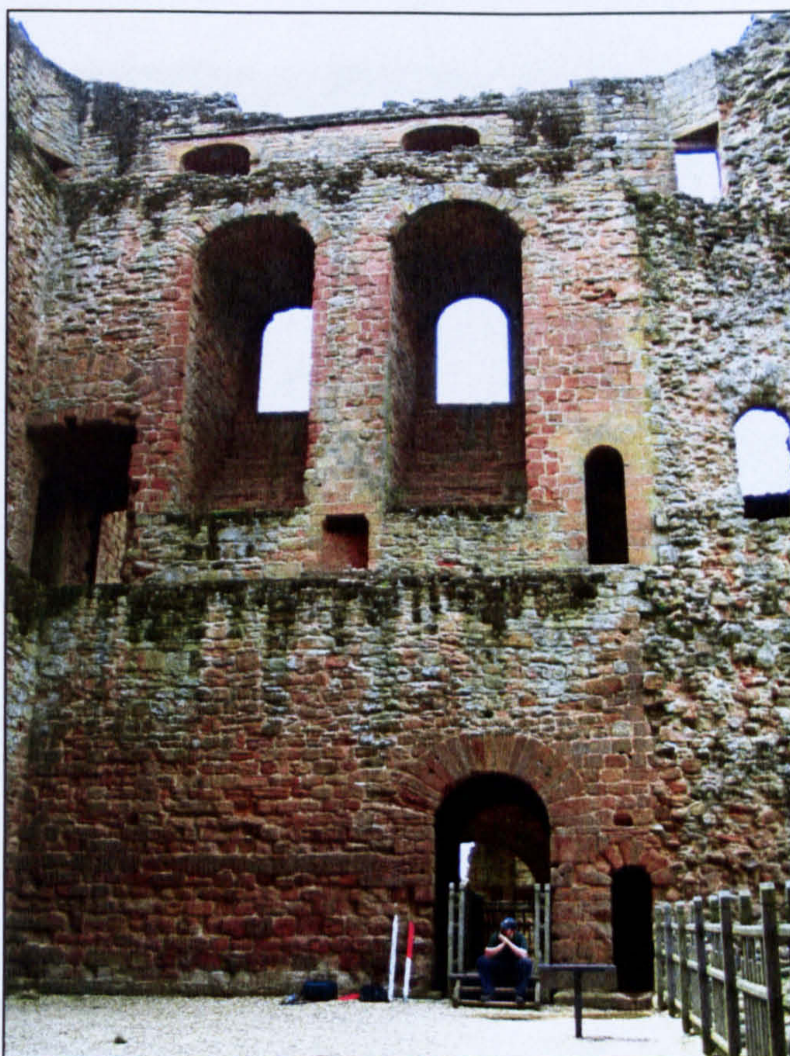
Figure 6.24 Clockwise from top left: The internal elevations of the east, south, and west walls, all showing a substantial amount of original, undamaged stonework.
