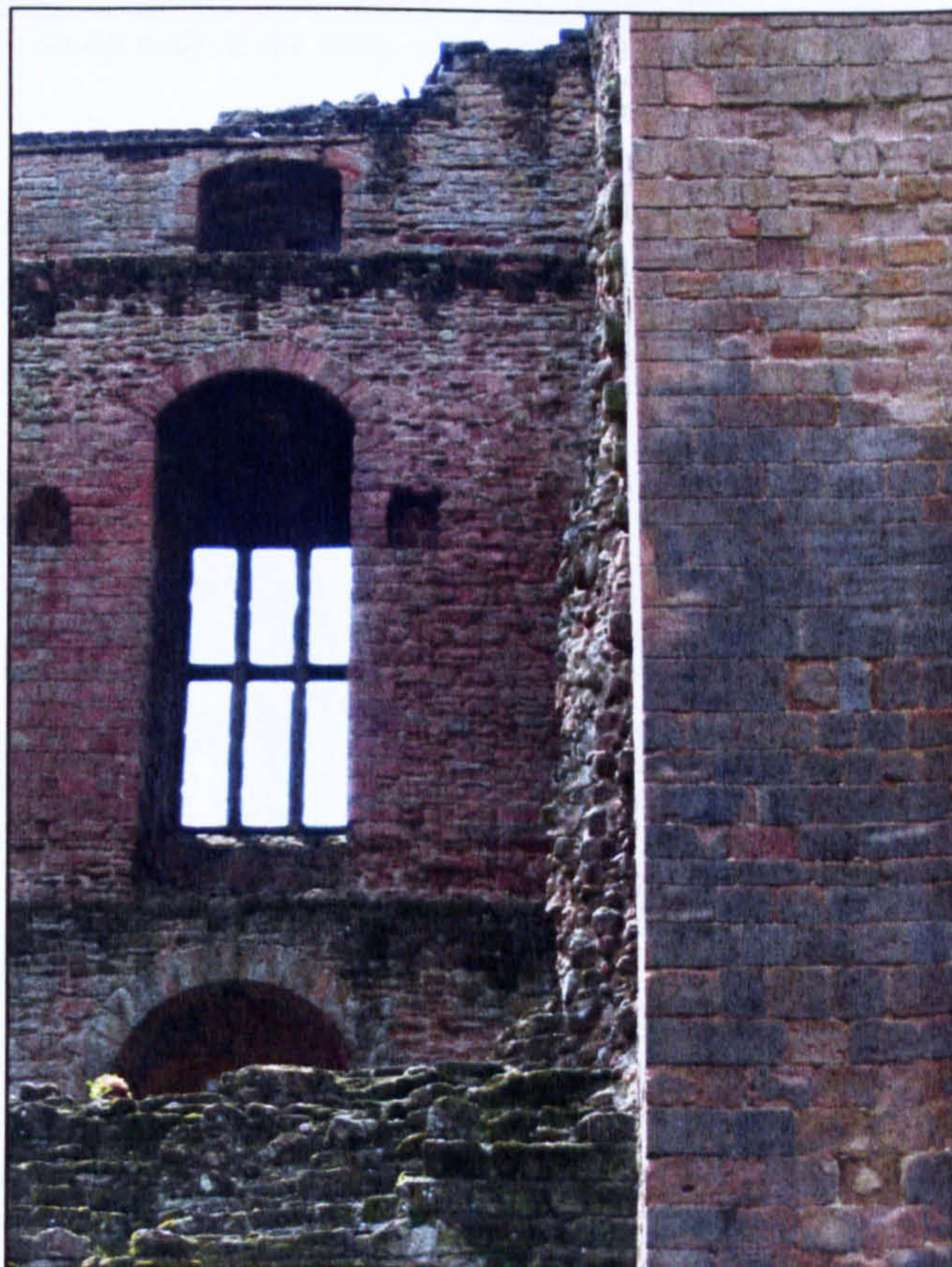
Figure 6.33 The northwest corner, looking south. Although some rubble core stands out, the right angle of the profile clearly shows that—if picked—the north wall was picked completely down to base level.
