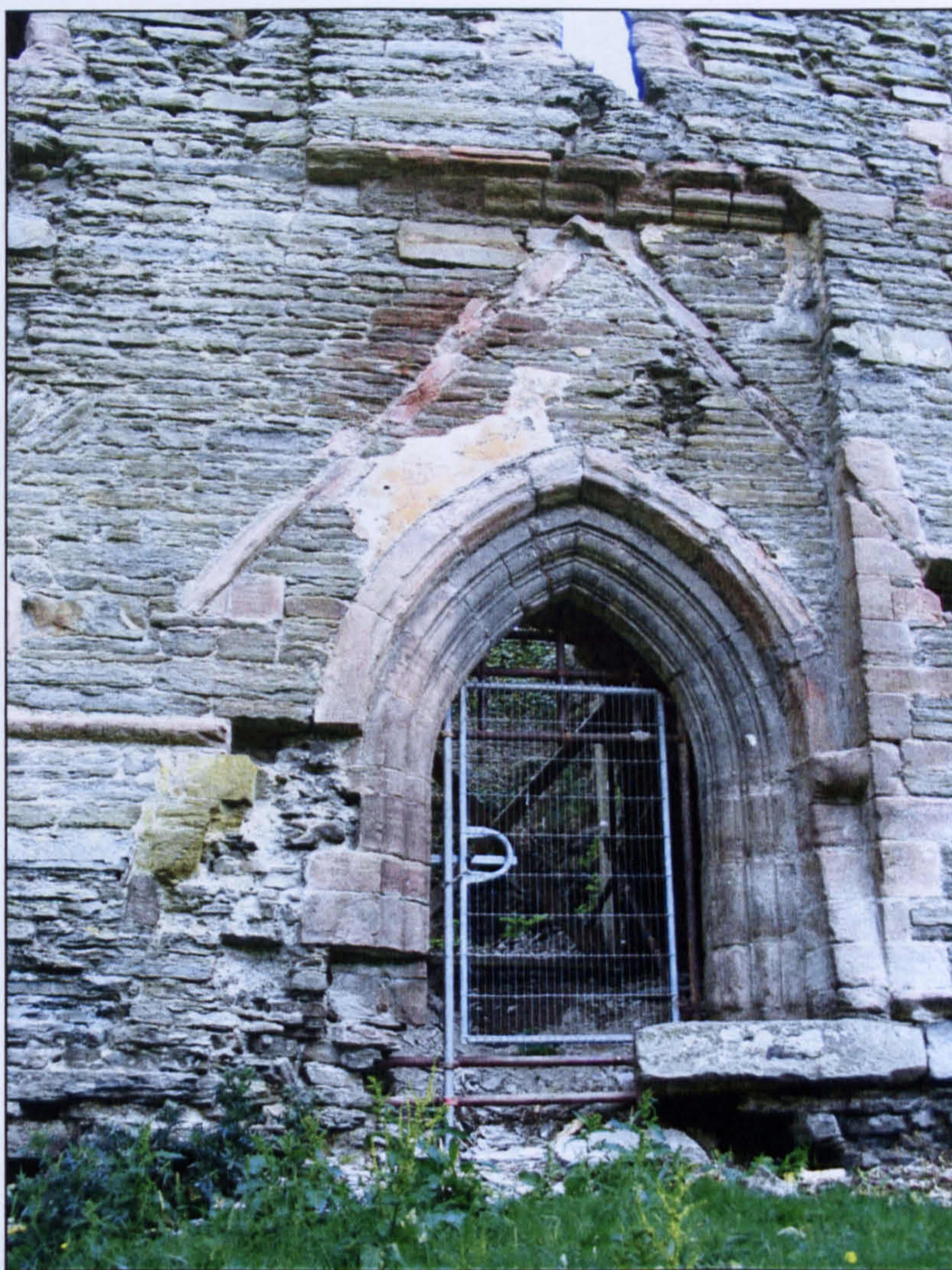
Figure 3.4 Porch area of Hopton Castle with alleged fire damage in upper left area of entranceway.
