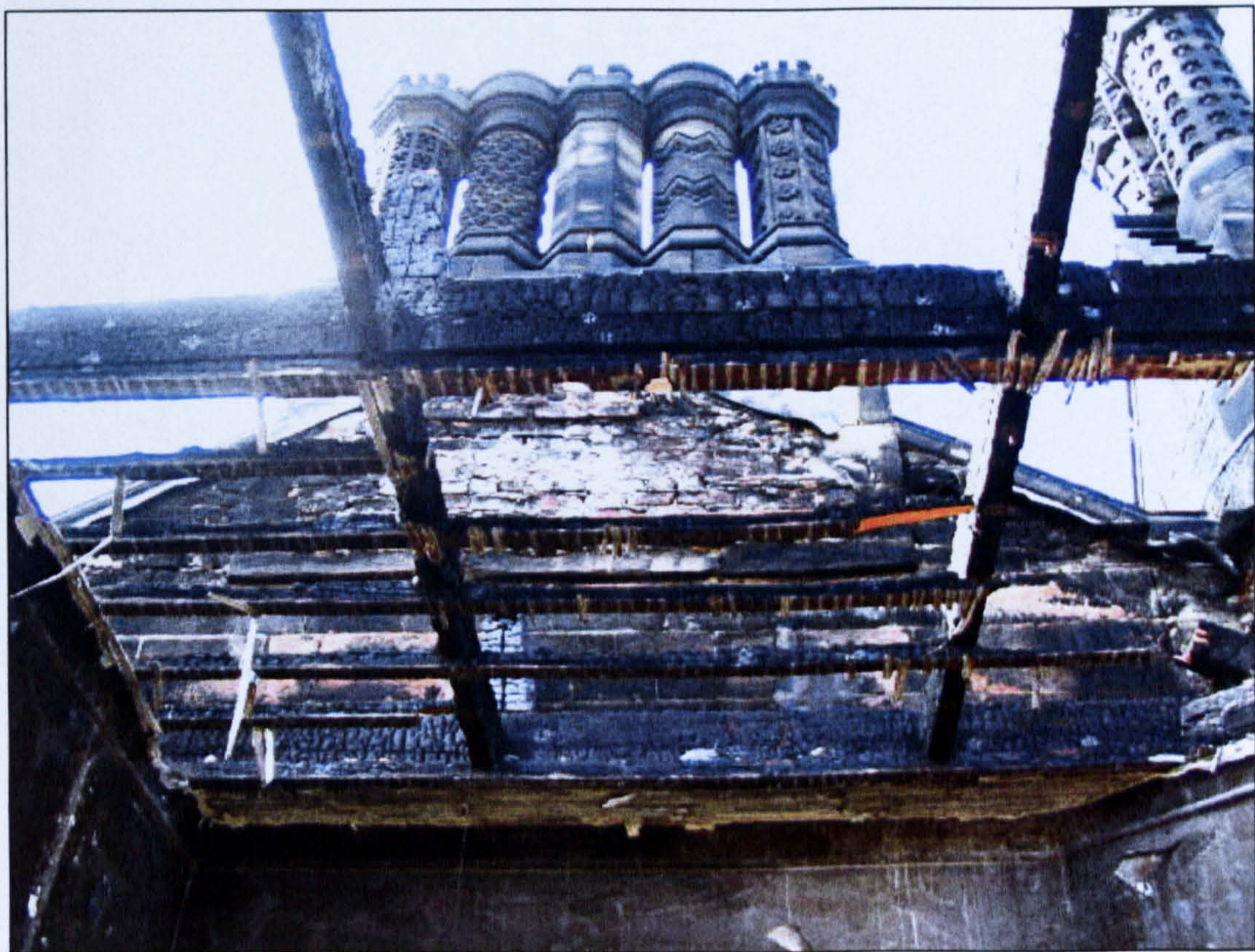
Figure 3.11 Roofing timber beams still in situ , showing signs of surface charring (Allerton Castle).
