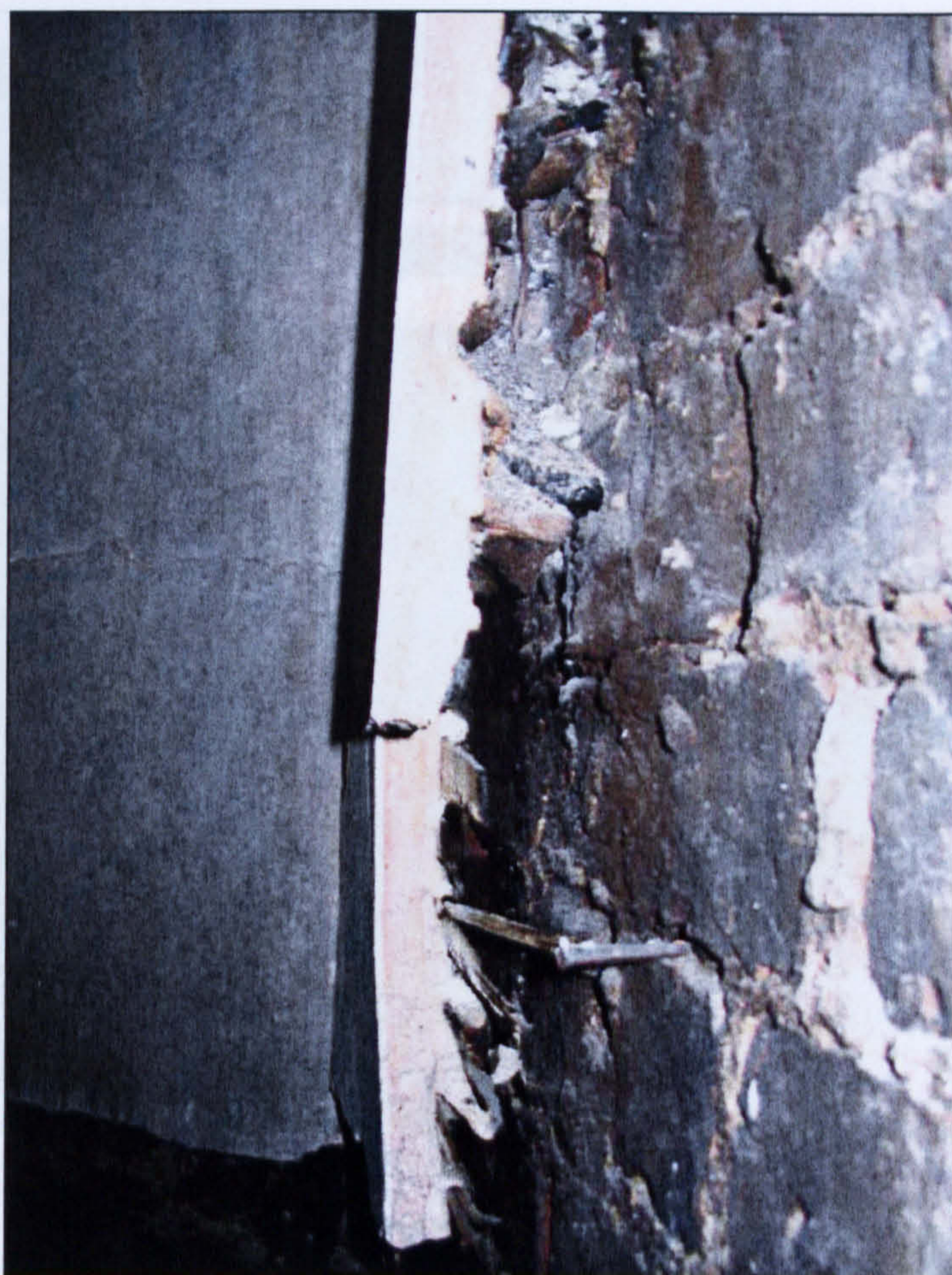
Figure 3.6 Panelling nailed into the wall at Allerton Castle, showing the air space that fed the fire.
