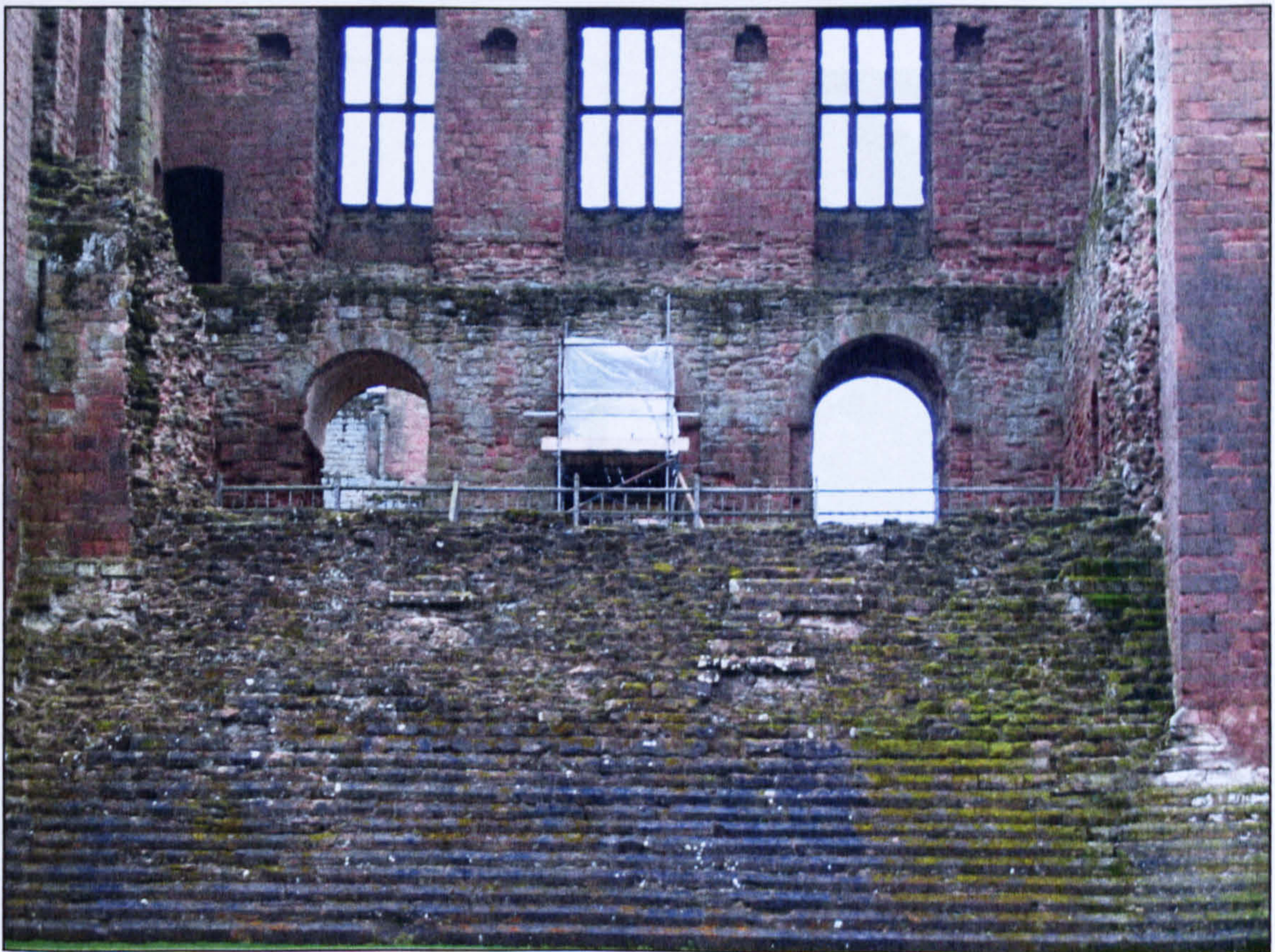
Figure 6.26 The north plinth, showing the damaged upper courses.
