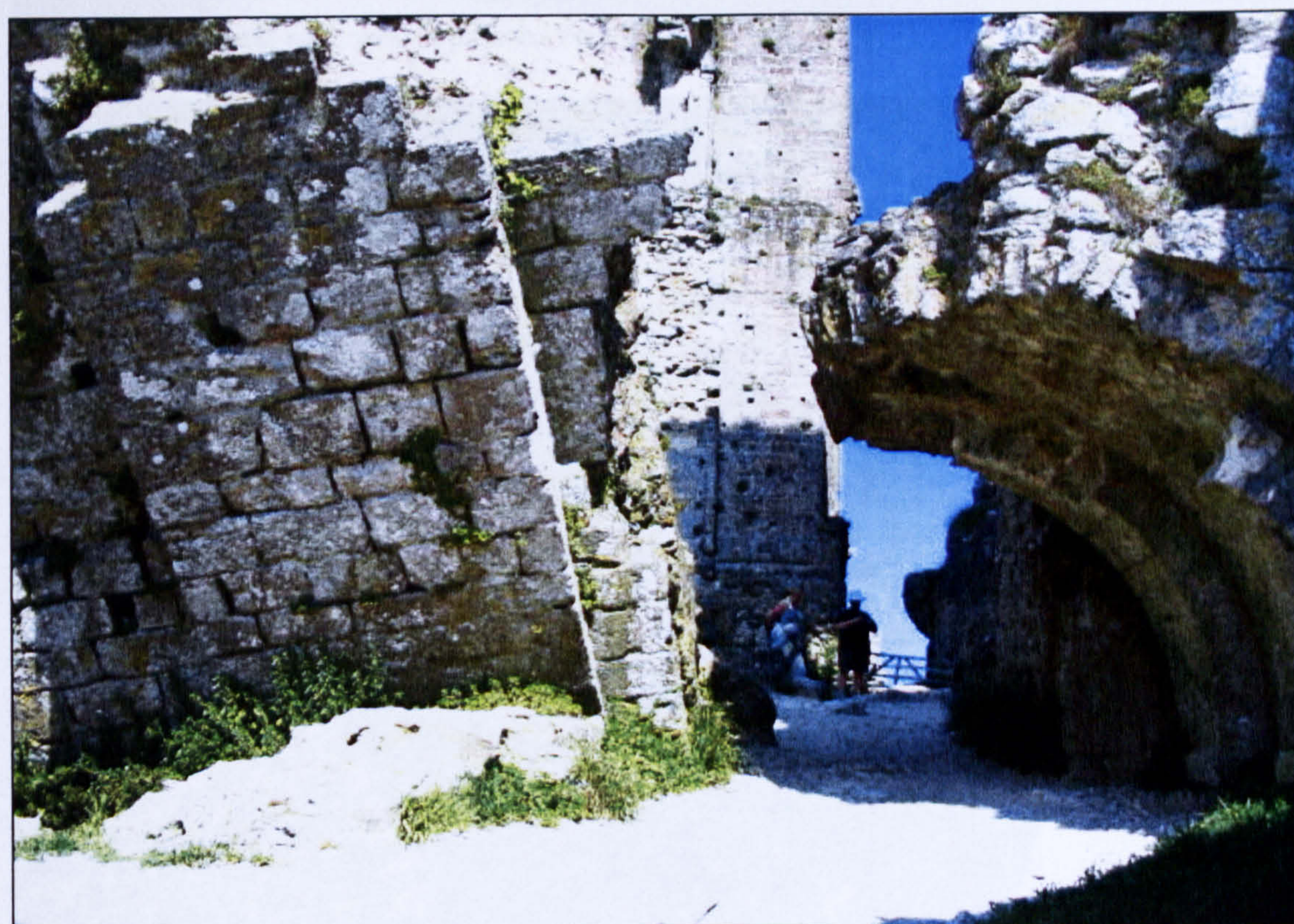
Figure 5.32 Leaning wall, west approach (View 1).
