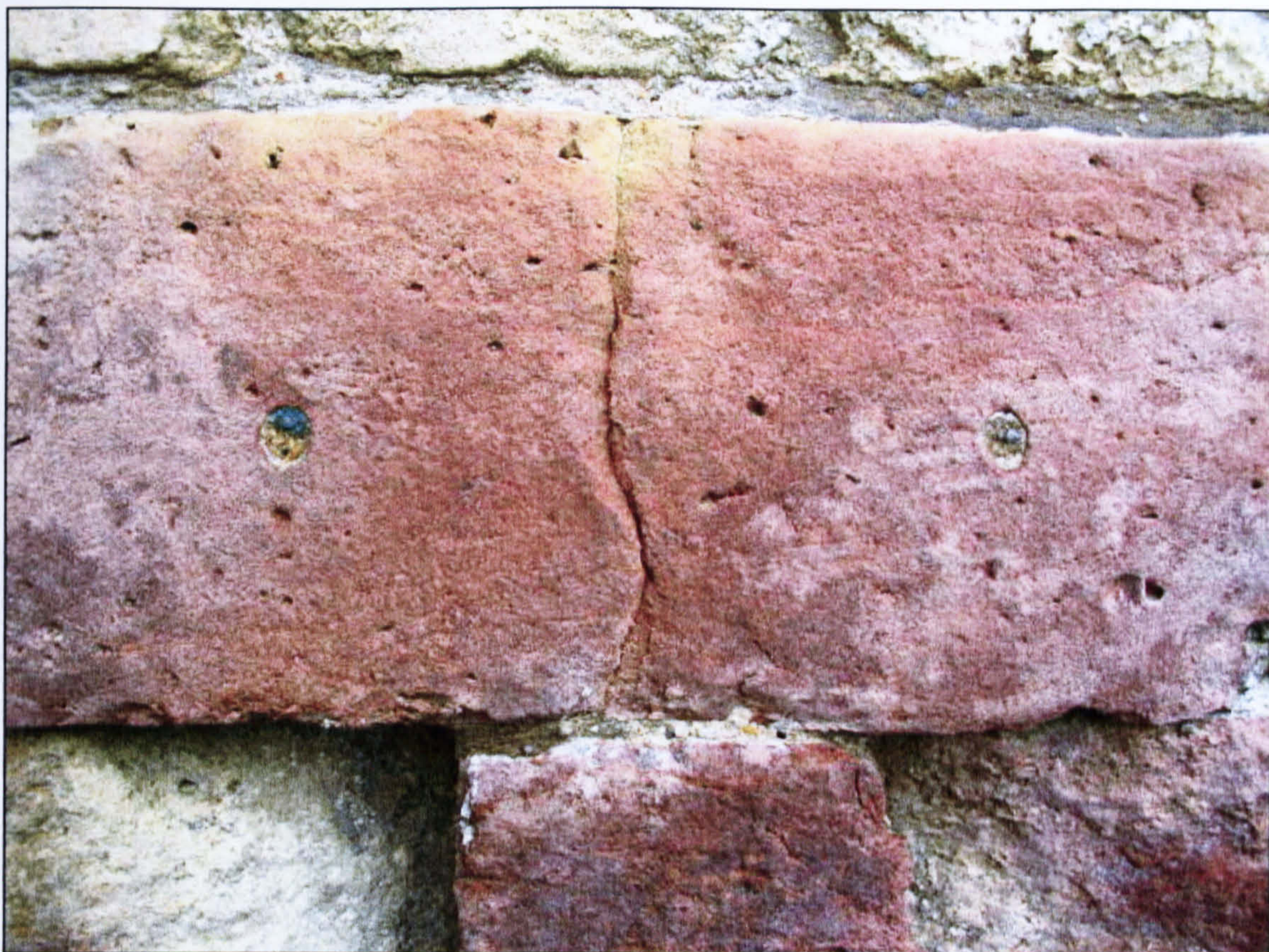
Figure 3.13 Close-up of the Knaresborough keep damage pattern, showing the twin bore holes on either side of the centre crack.
