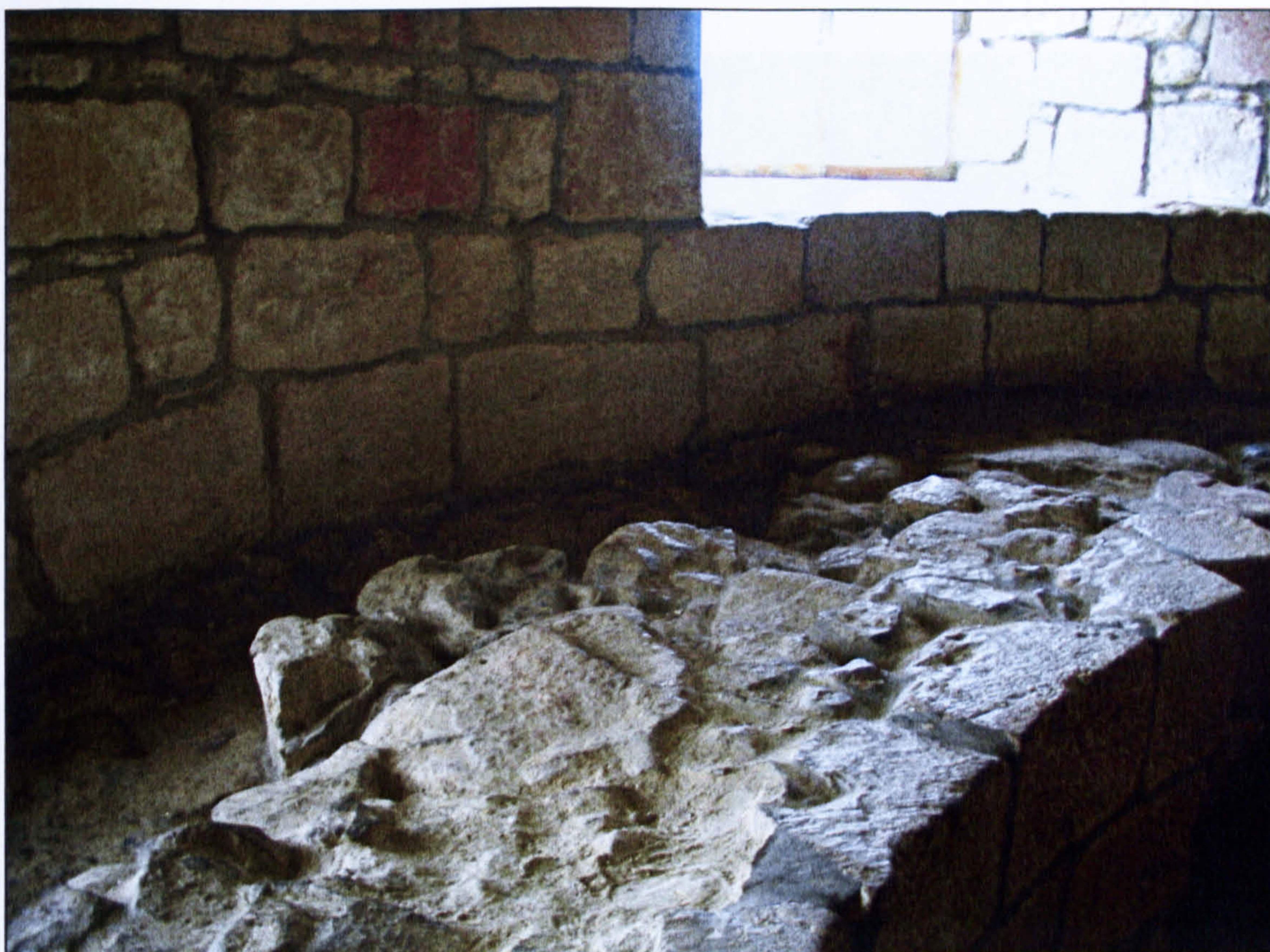
Figure 4.5 Close-up of the wall junction between pre and post slighting building phases, Skipton Castle.
