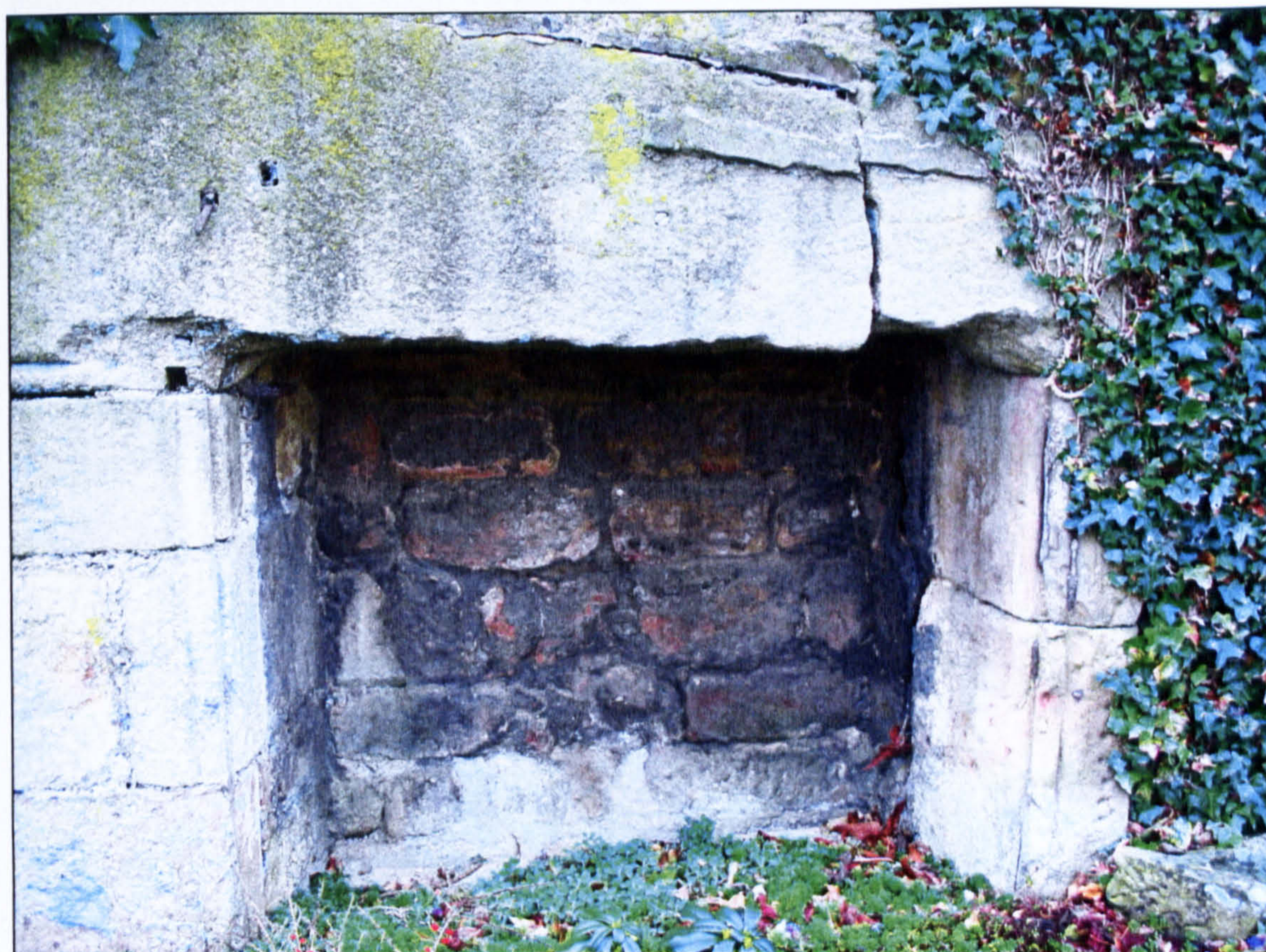
Figure 4.54 Close-up of ‘fireplace’ showing angle roll mouldings and geological difference of stones.
