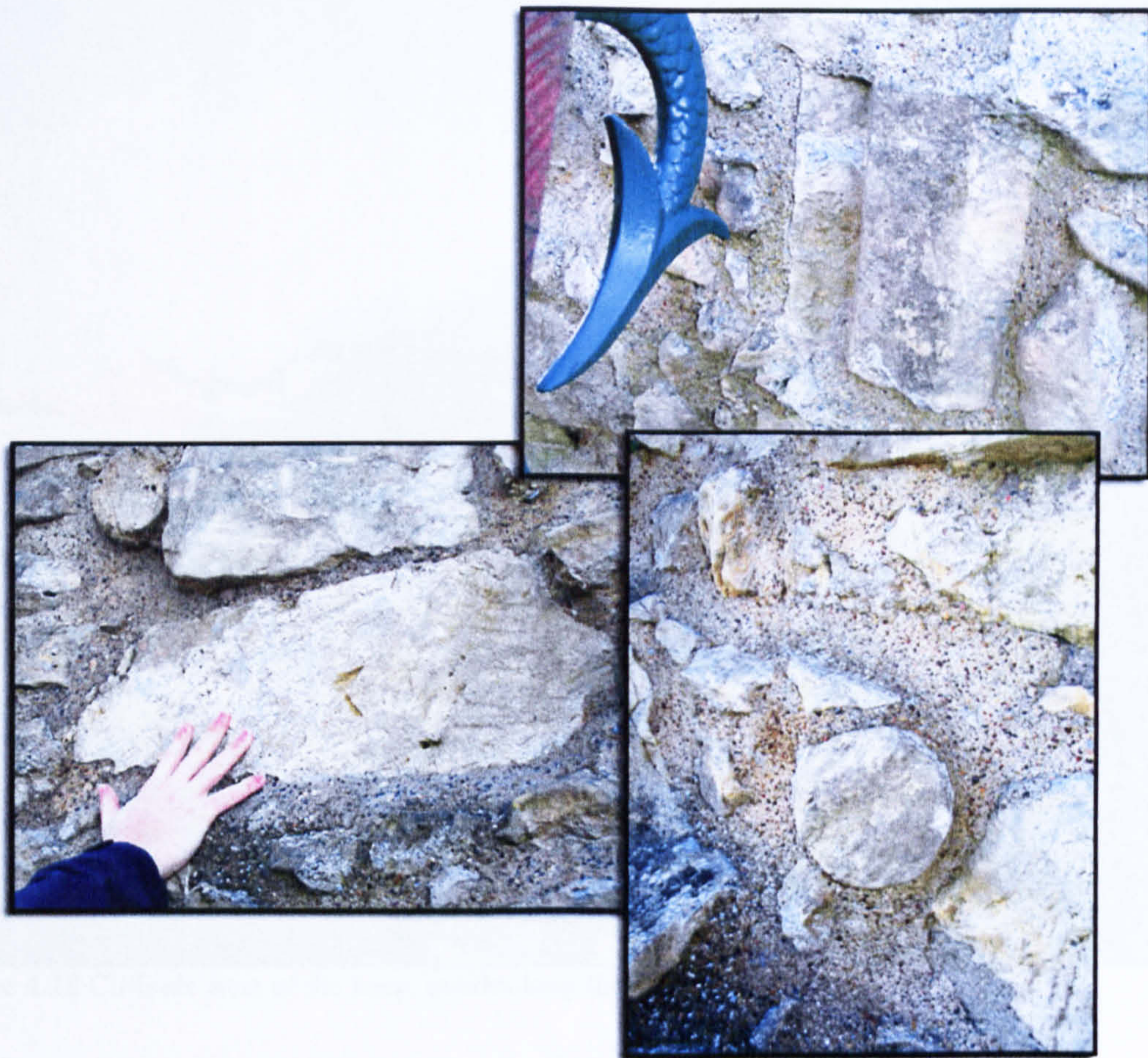
Figure 4.26 Clockwise from left: ashlar with claw tooling, architectural fragment with chamfered moulding, and a nook shaft from a window or door, all located in the rubble core of T2.
