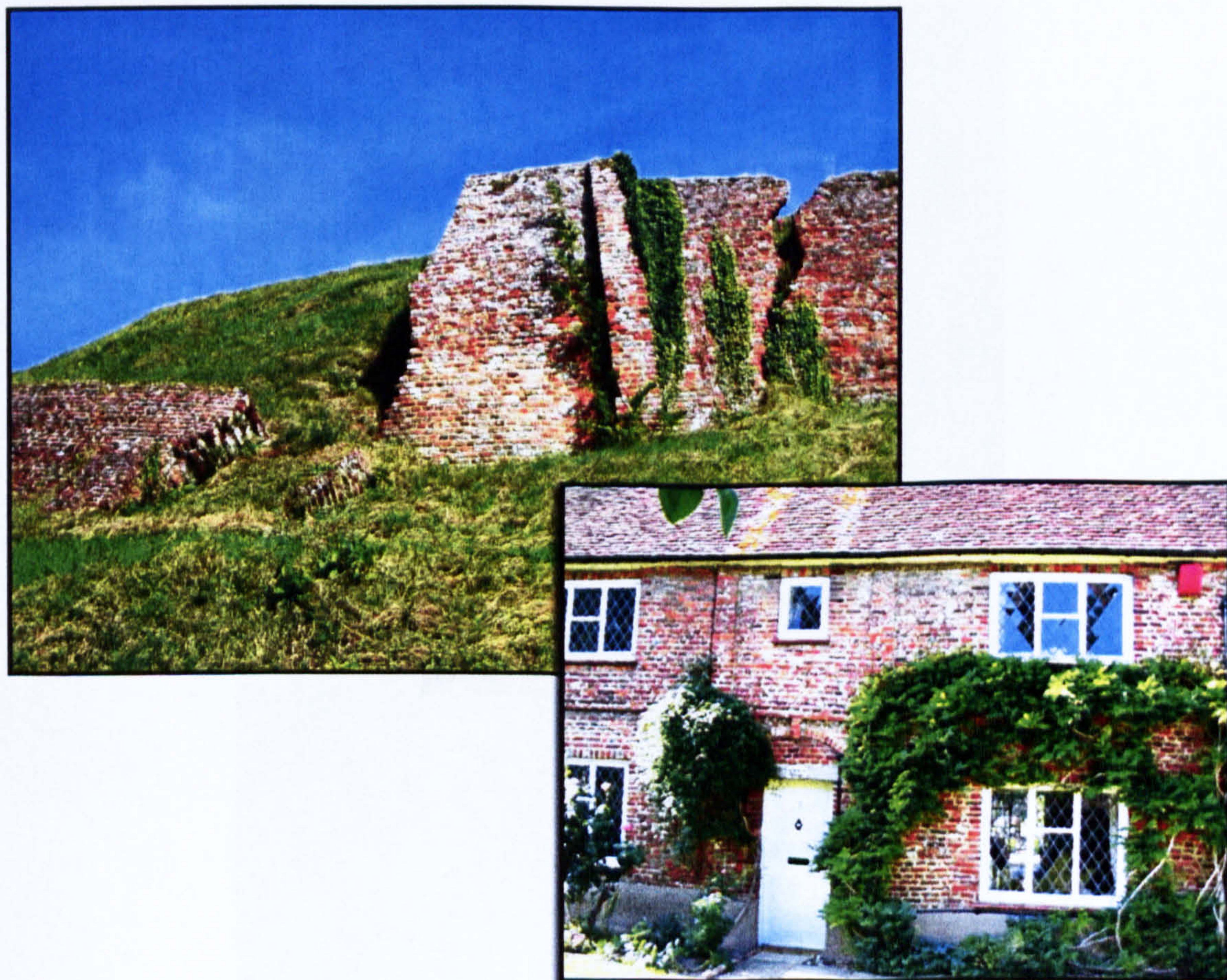
Figure 4.39 Left : Damaged curtain wall at Basing House. Right : House built from castle brick in Old Basing.
