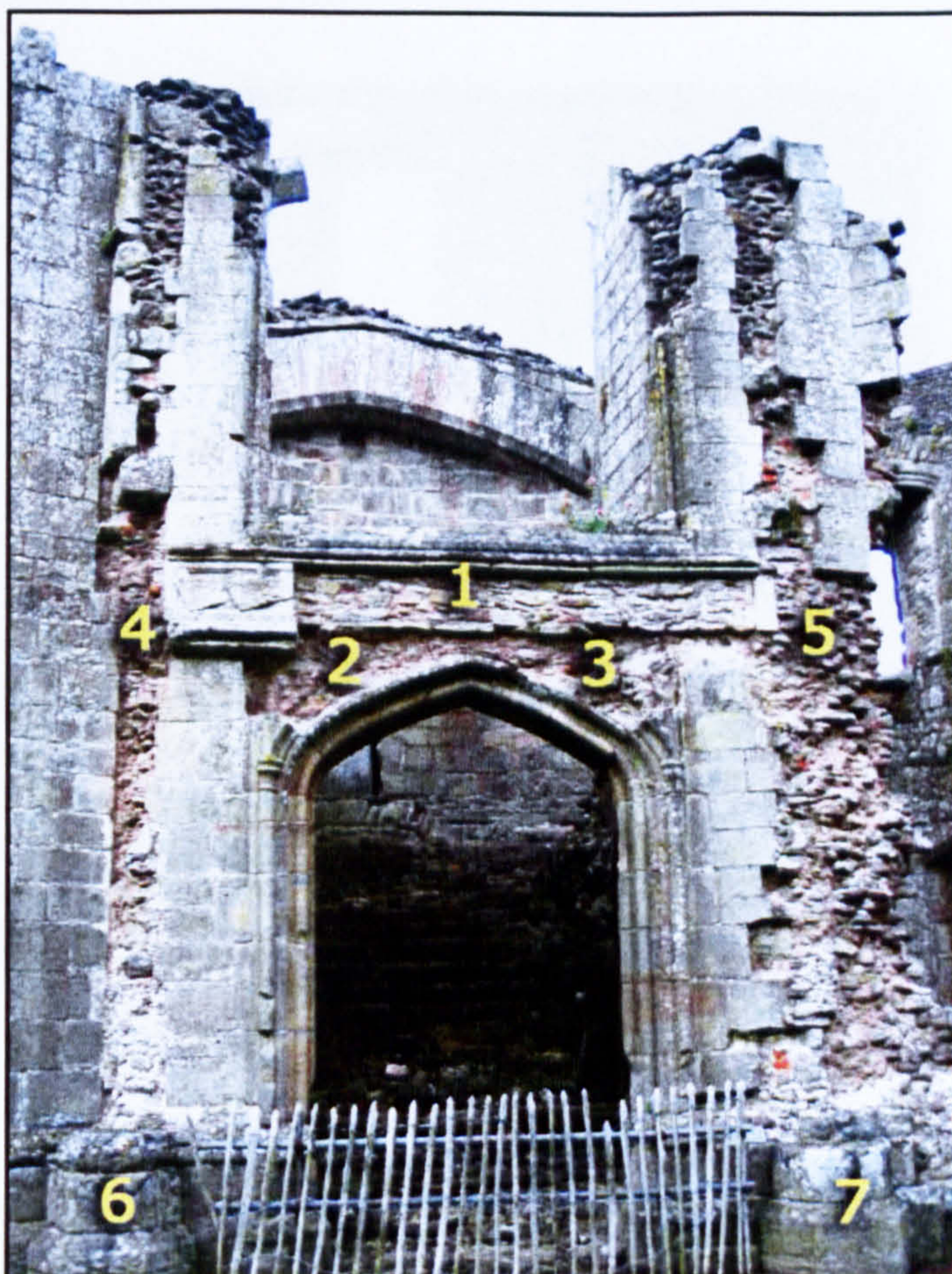
Figure 4.58 The Grand Stair leading to the apartments in the Fountain Court, with areas of secondary damage and various features numbered.
