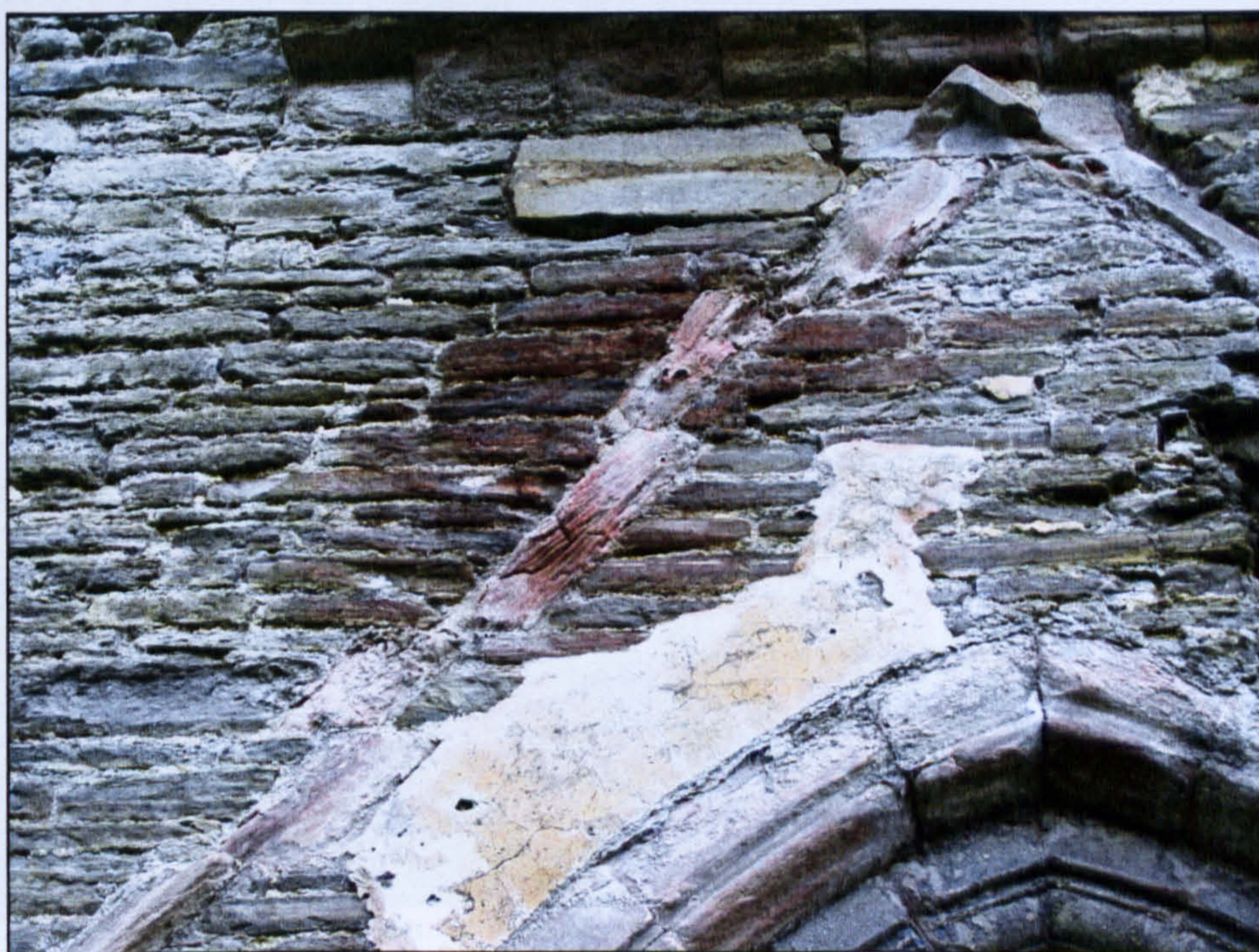
Figure 3.5 Close-up of fire damage area, Hopton Castle.
