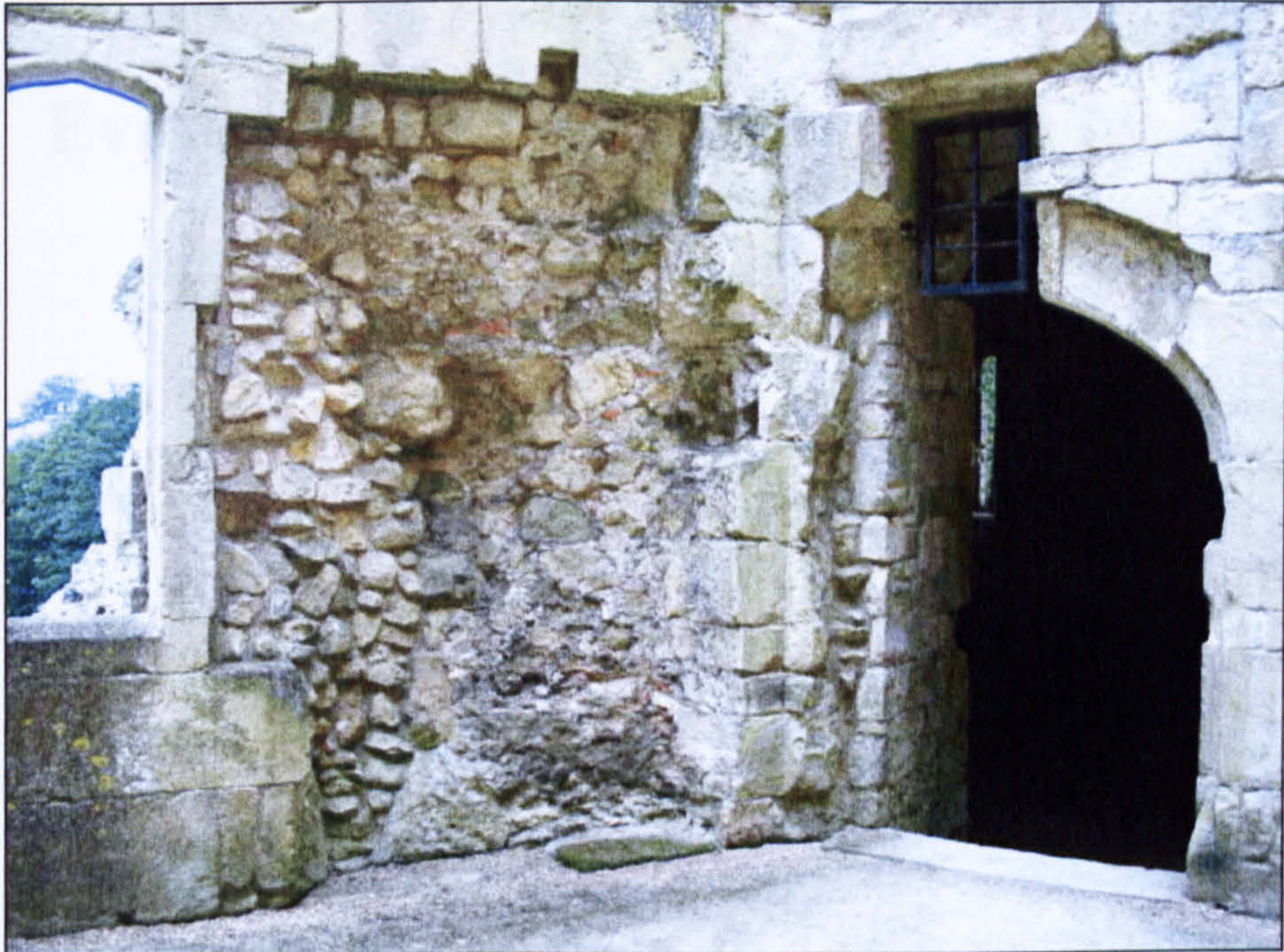
Figure 4.61 Close-up of secondary damage pattern across from the Great Hall staircase at Old Wardour (Wiltshire).
