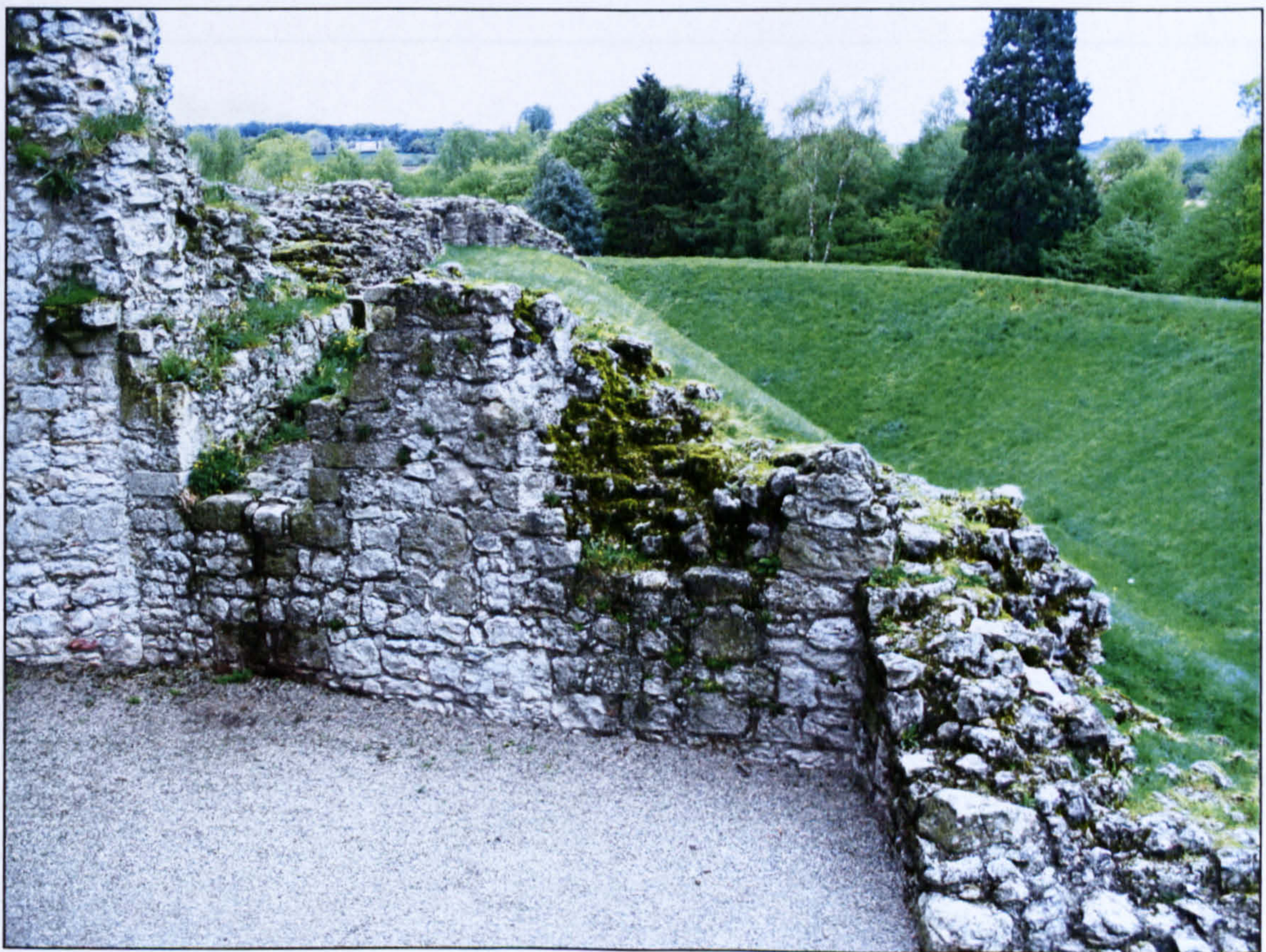
Figure 5.55 The internal north wall of the keep, showing the gradations of wall height, the postern gate (left), and corner recess (right).
