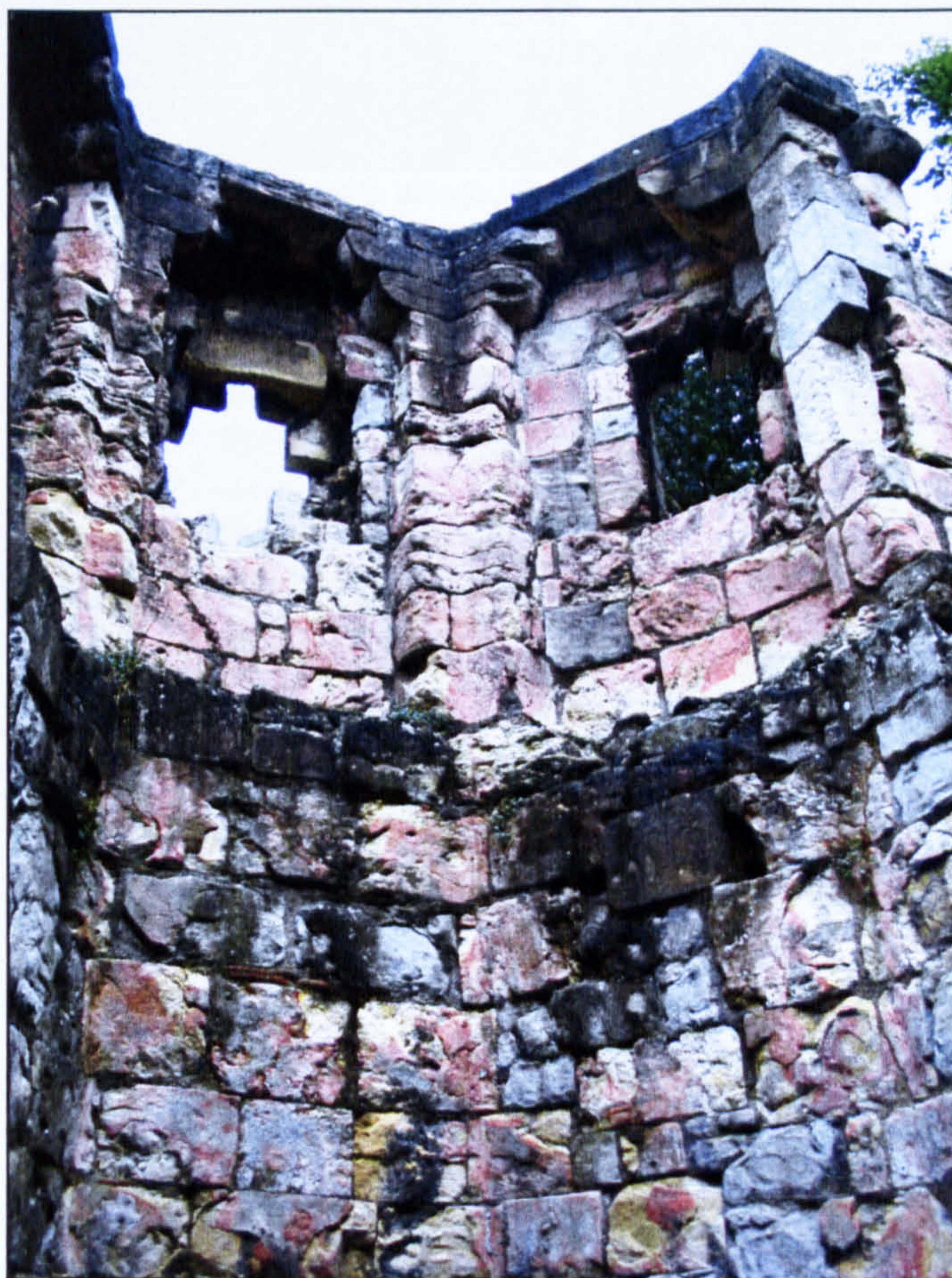
Figure 3.3 Extensive reddening and surface degradation of fire damaged wall, St. Mary's Abbey.
