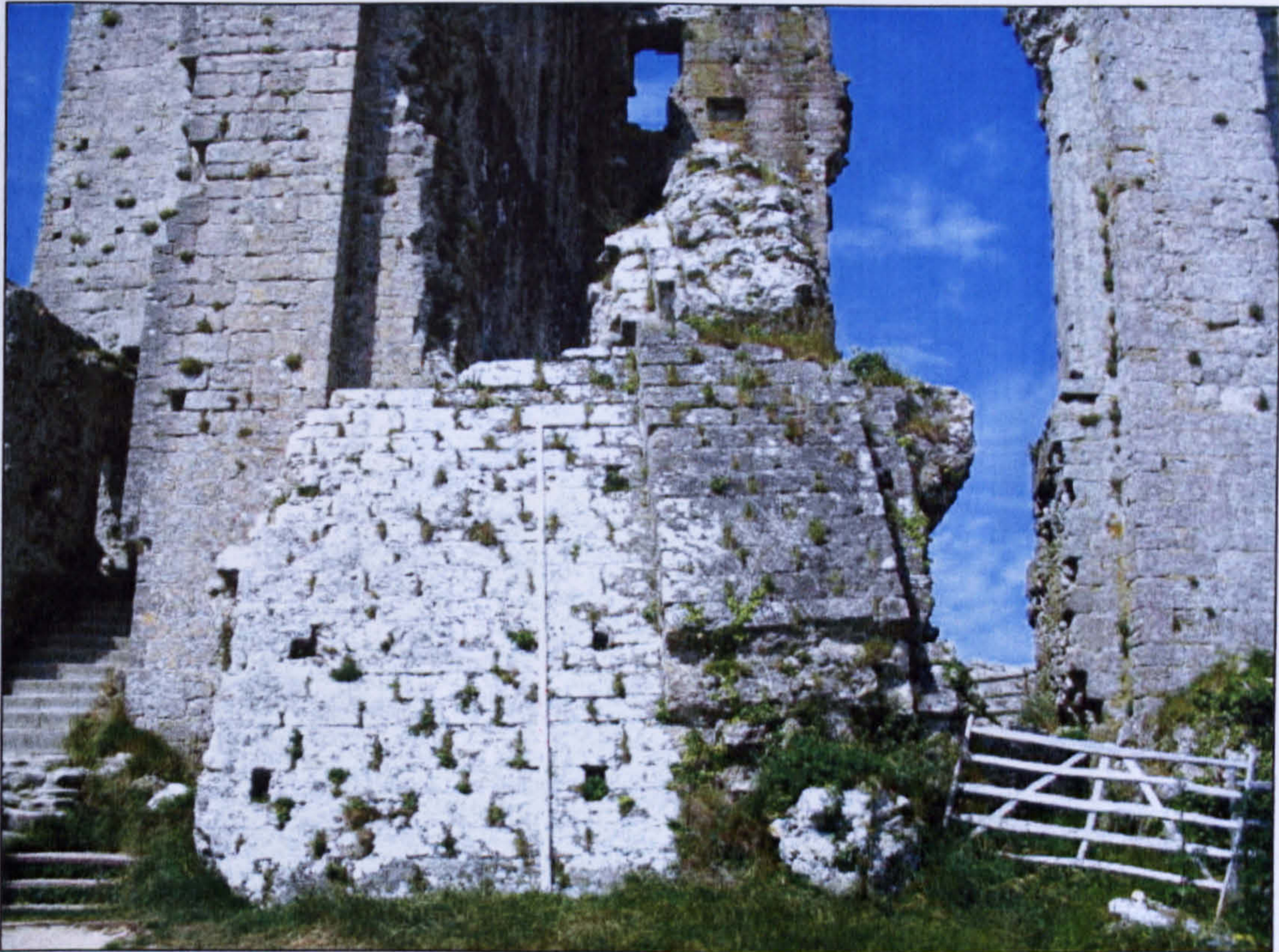
Figure 5.27 Close-up of east elevation and fallen part of wall
