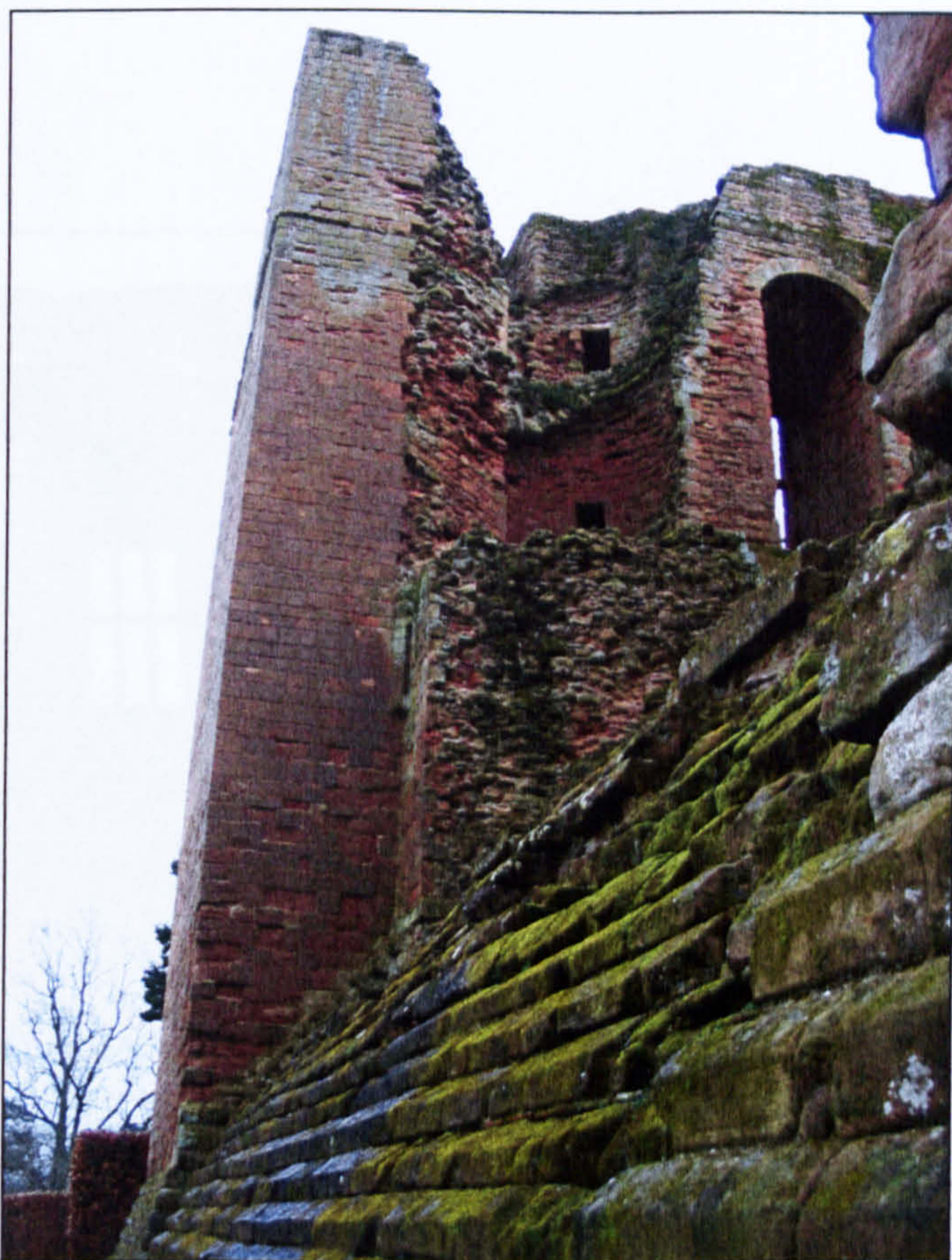
Figure 6.22 The northeast corner, showing the former point of connection with the north wall.
