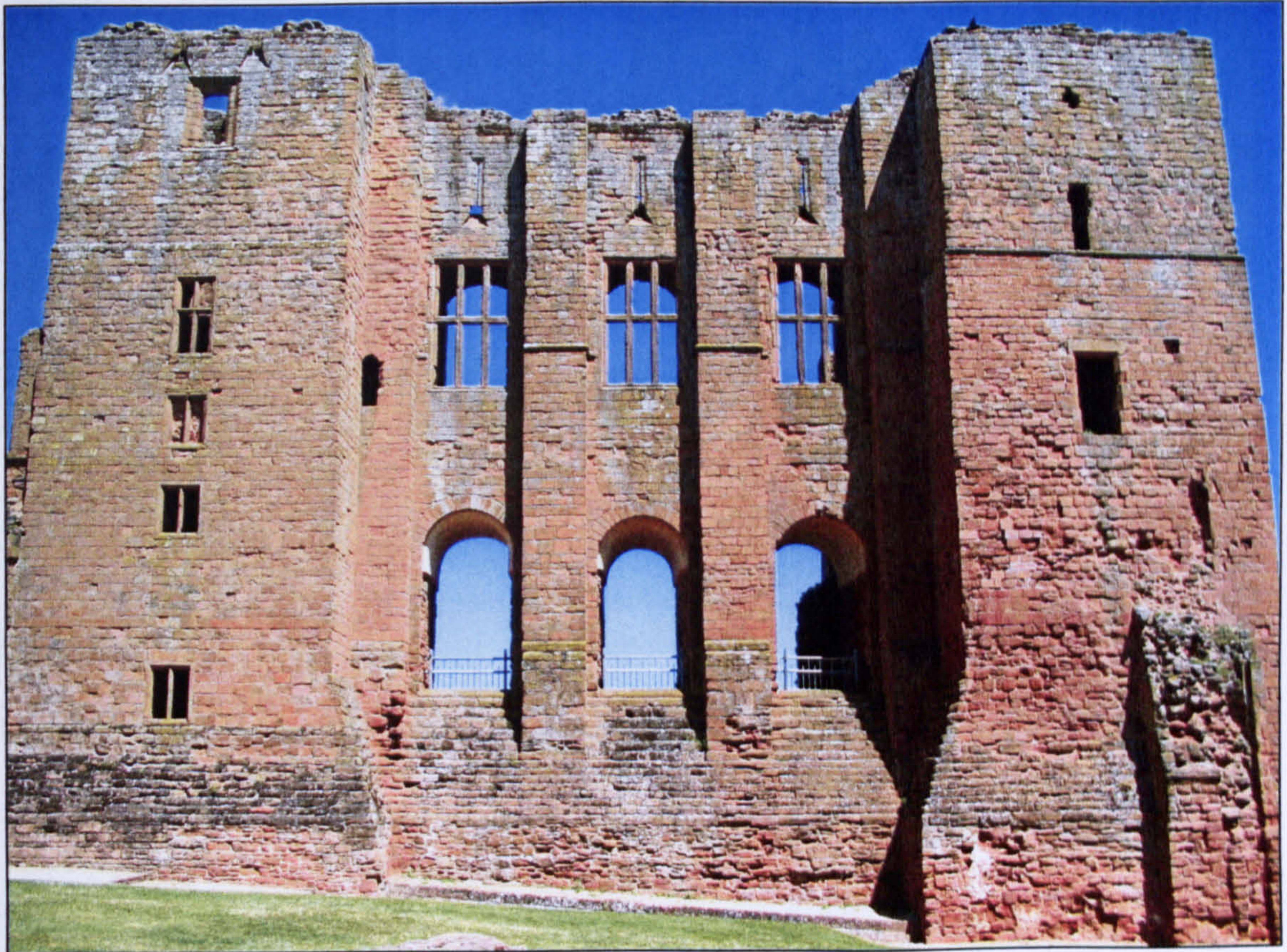
Figure 6.34 The intact south wall of the keep, showing Leicester's inserted Tudor windows.
