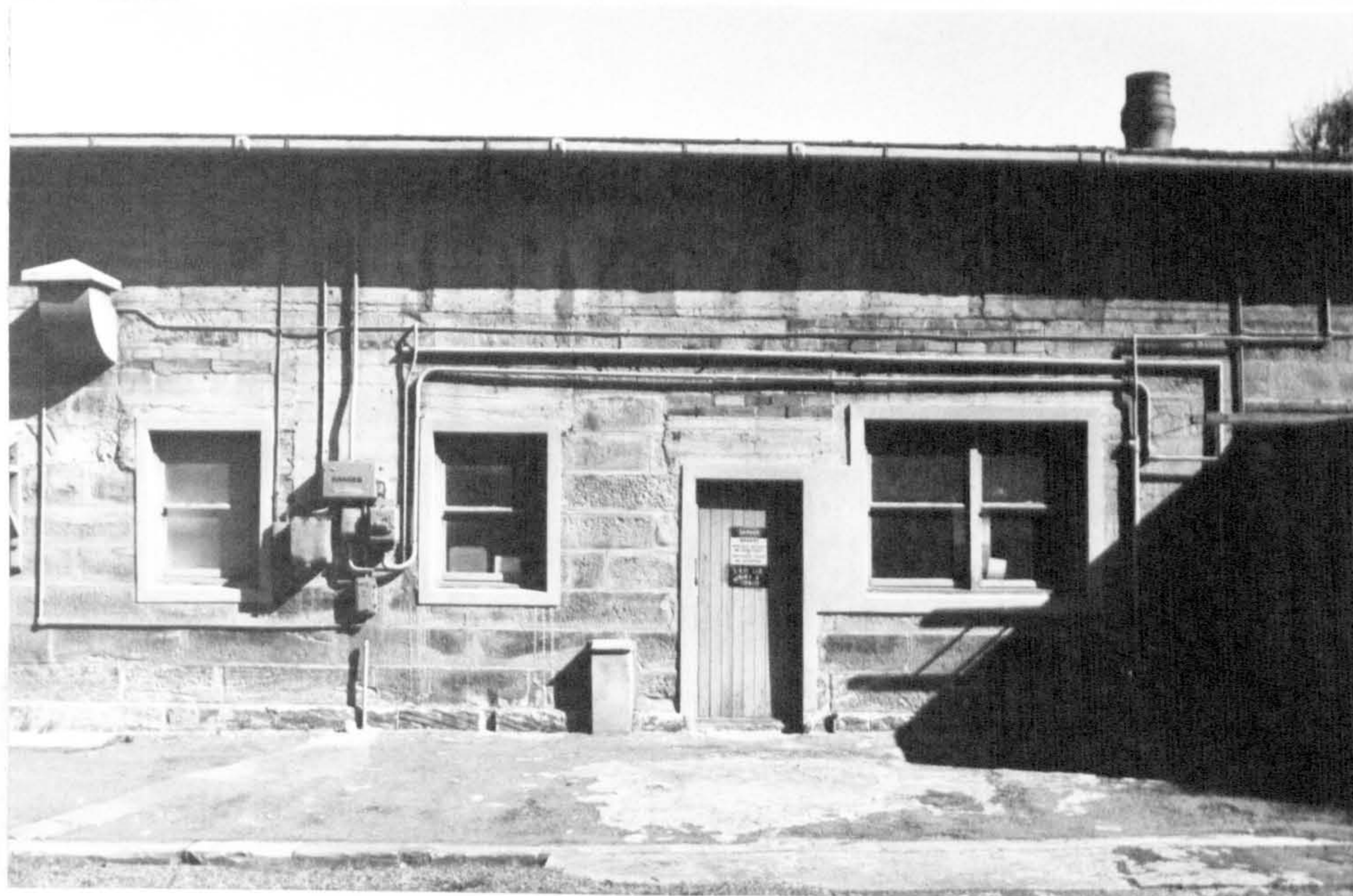
Plate 8. Cockatoo Island, NSW. Centre section of barrack in plate 6, 1974, under Australian Government ownership. Neg. No. JSK 74-19-18
