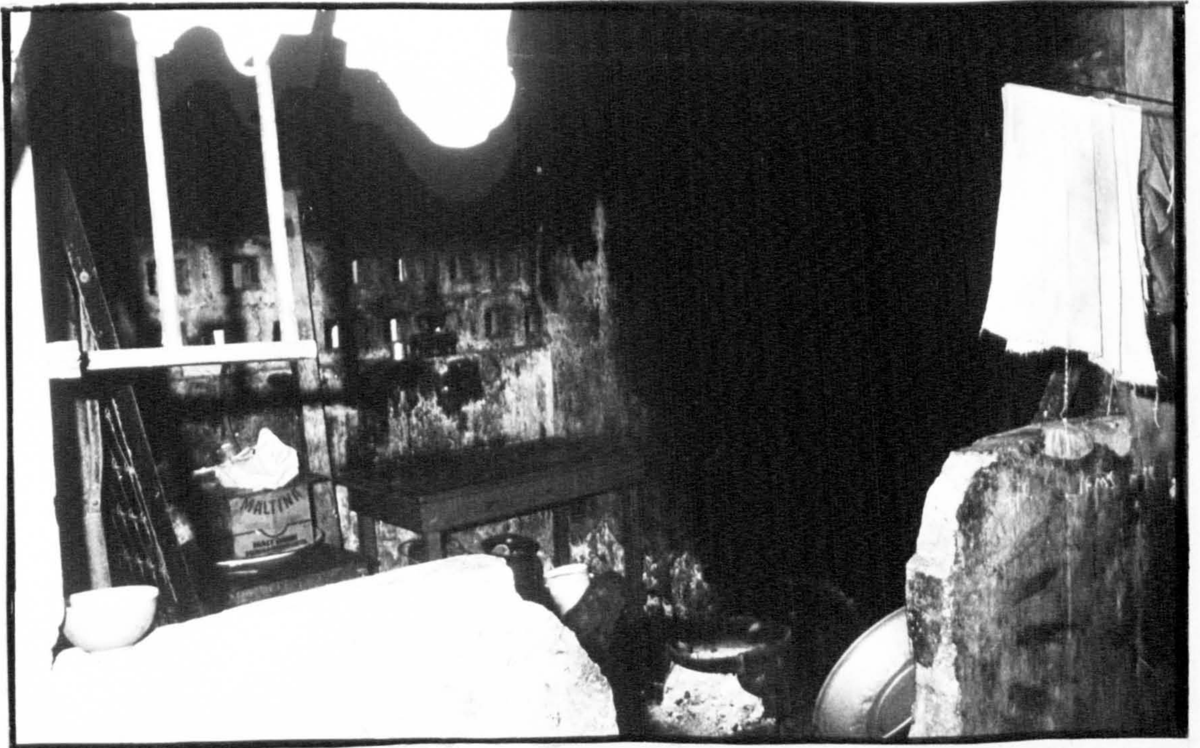
Figure 051. Firewood Cooker in Shared Kitchen off Courtyard at the rear of the Rooming House, Maroko.
