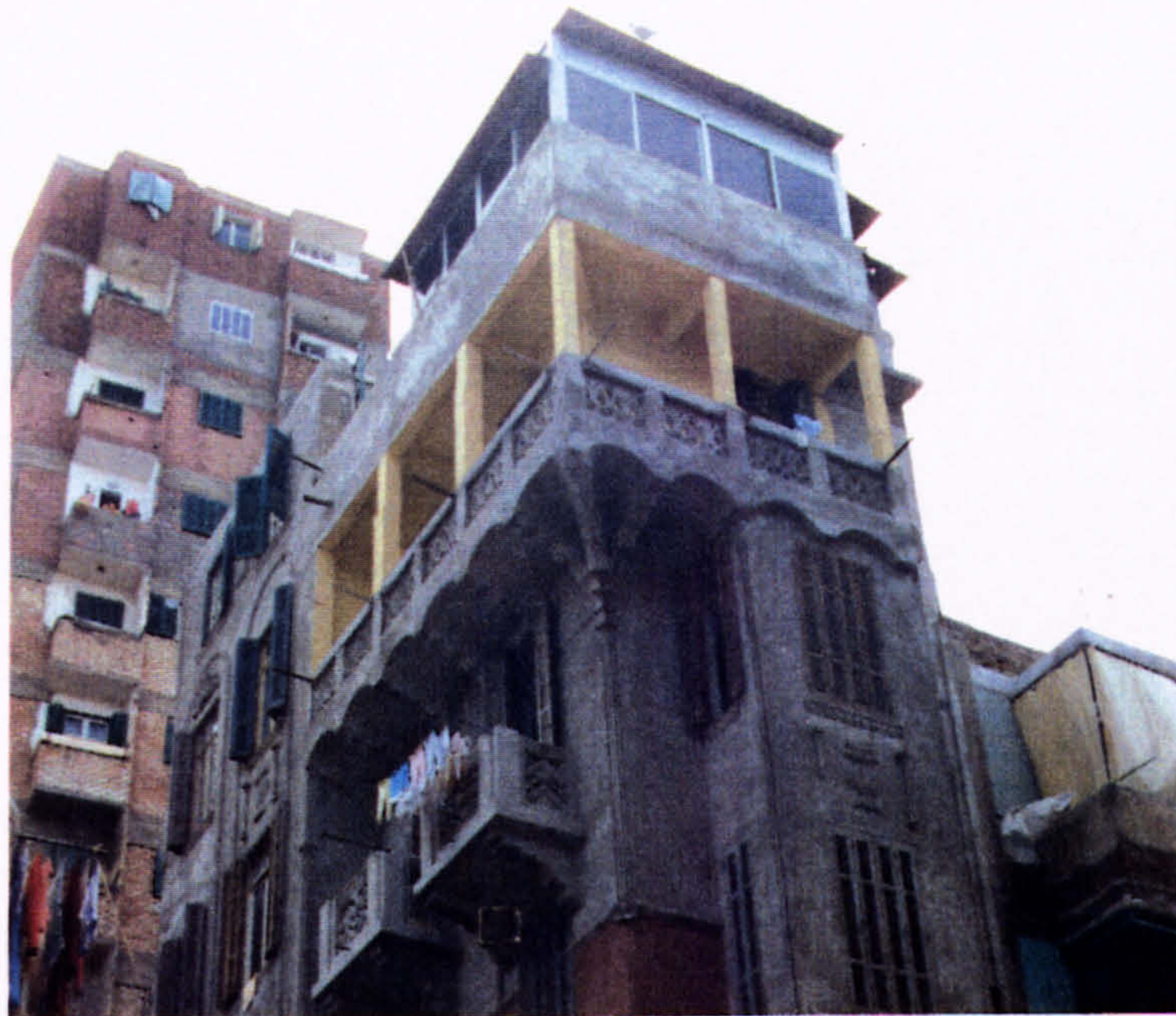
Fig.6-2 , alterations and extensions to existing buildings; the quality of these extension, not only the aesthetics, but the structural as well is very much in question. A result of increasing land prices and shortage in housing supply.
