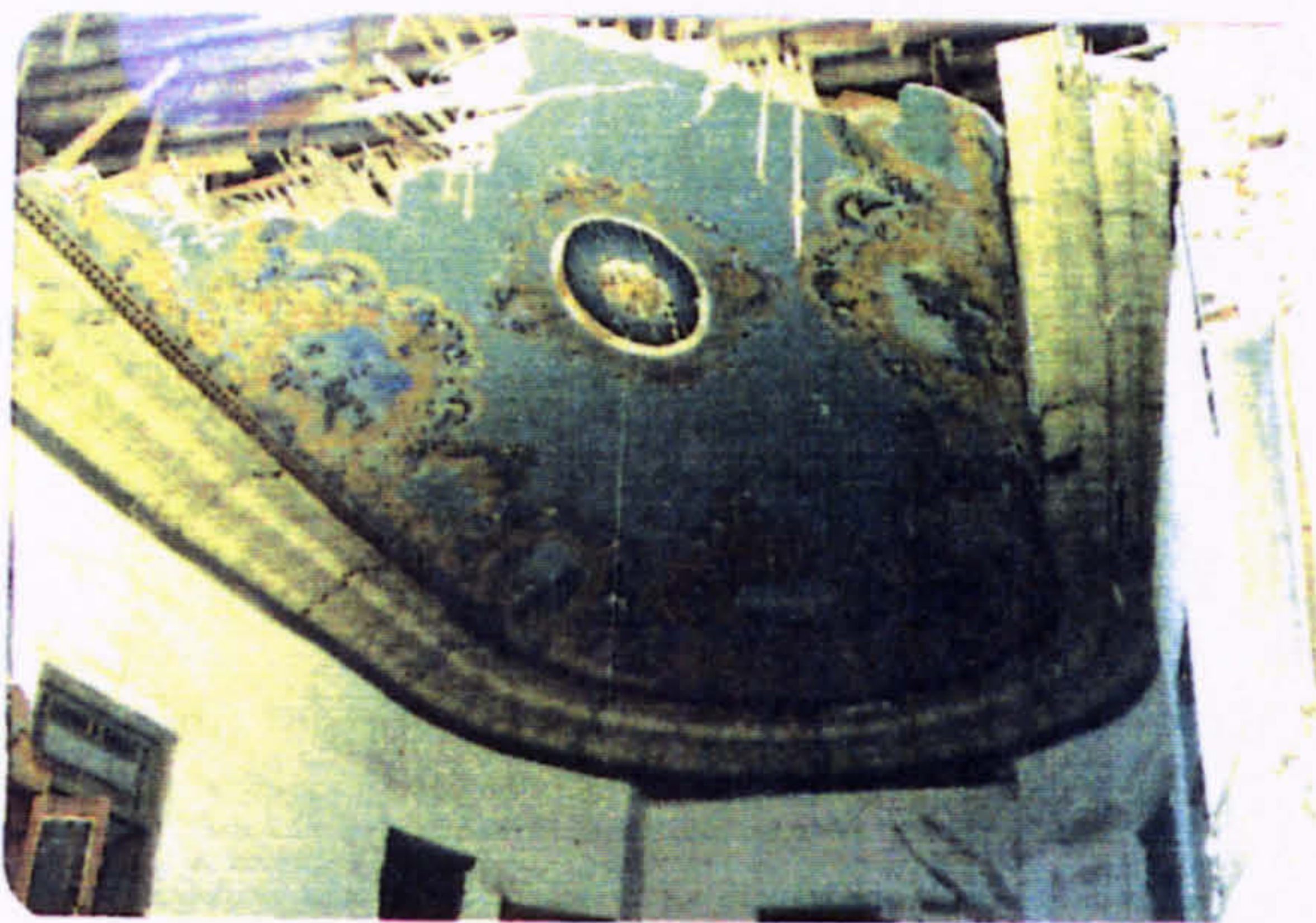
Fig.3-9, Hallabo house, Alexandria; a non listed building, which dates back to the early 19 th C. is falling down because of neglect.
