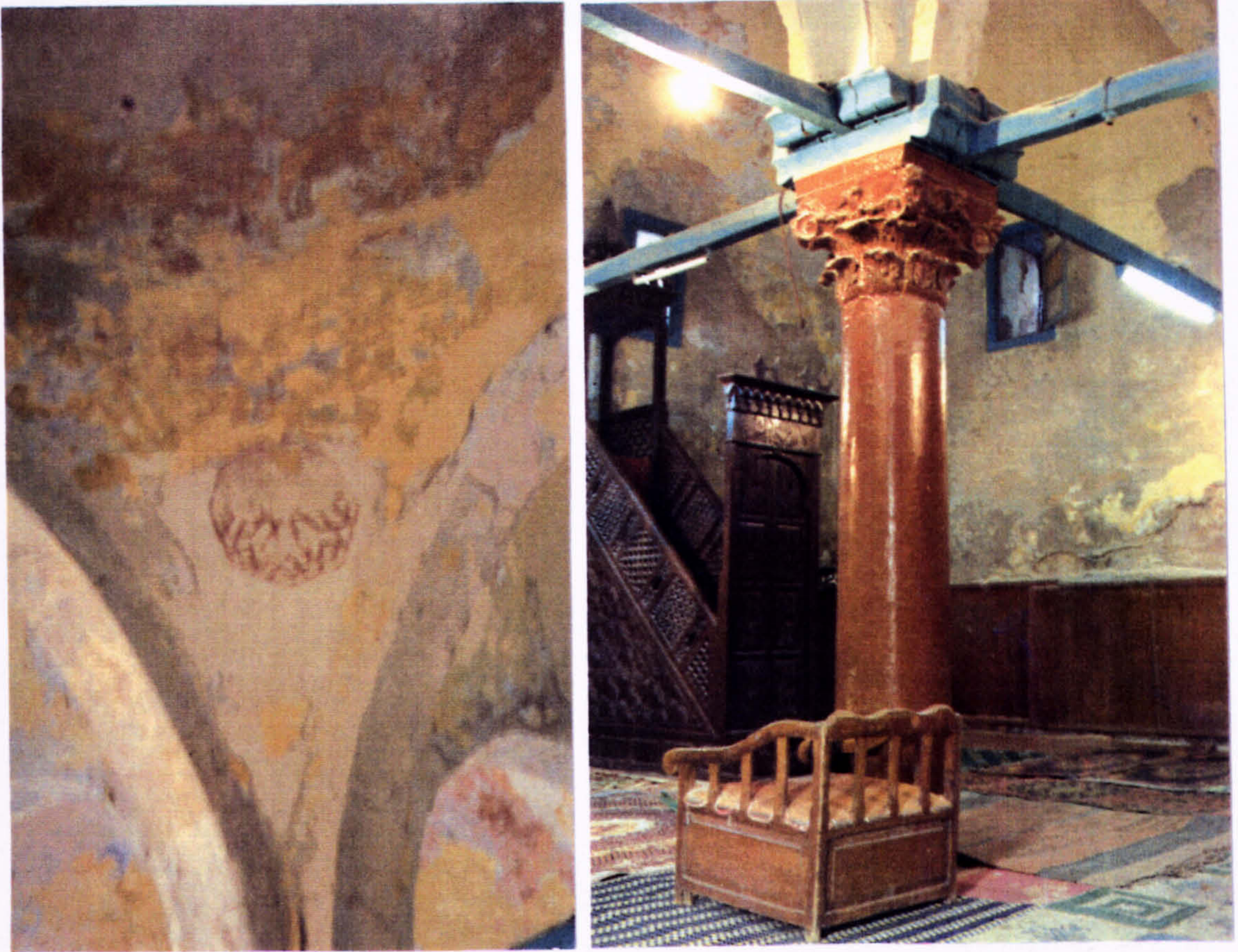
Right, the interior of the mosque, note the Minbar and the Corinthian capital; Left, the decay and deterioration of plaster and render work.
