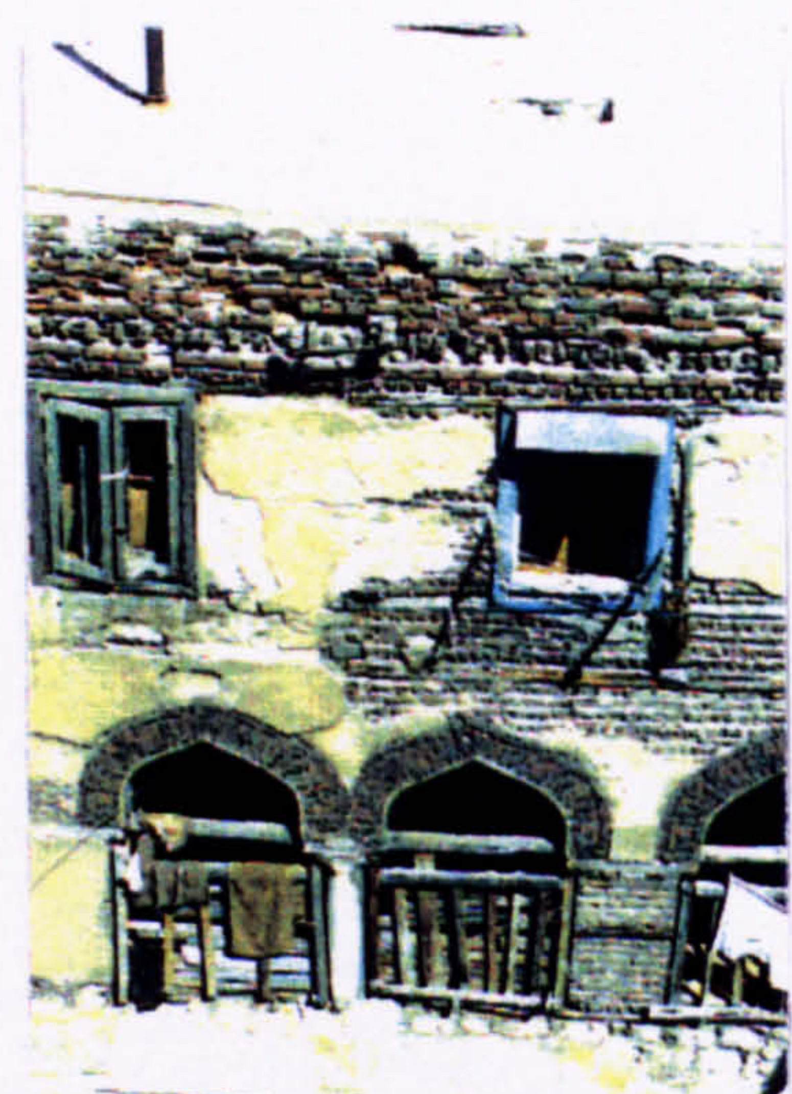
Fig.8-13, Right, inadequate rain water system causing dampness to the masonry, plaster, tiles and timber; Left, the courtyard facade; the use of brick and timber tie-beams; are in a very poor state of repair.
