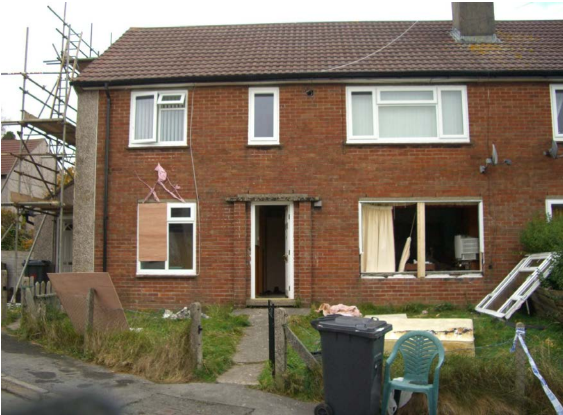
Figure 2-18 Accidental gas explosion where early failure of the window has provided adequate vent relief and prevented structural damage to the property
