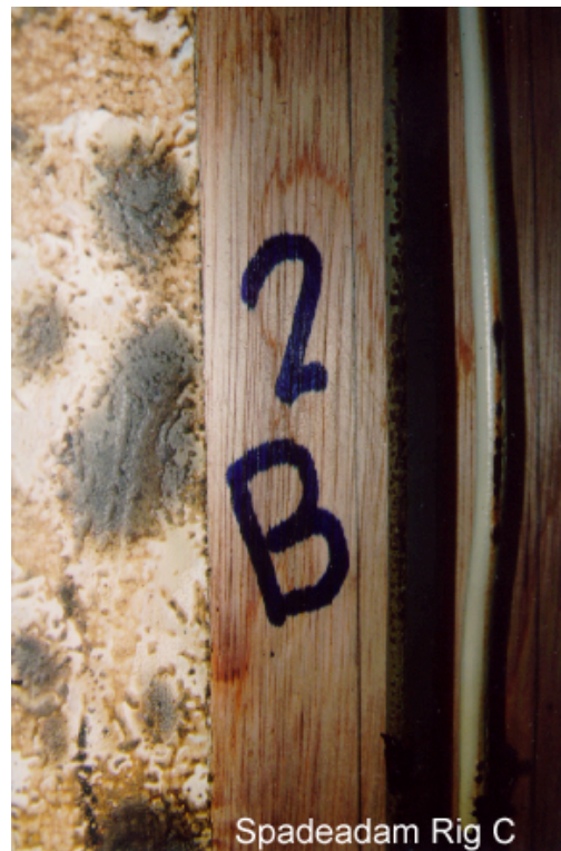
Figure 6-1 Typical mottled pattern of thermal damage (Rig C)
