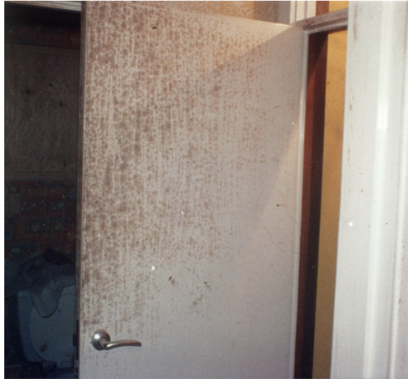
Figure 6-21 Evidence of scorching on the upper section of an internal door (taken from DNV GL archive)
