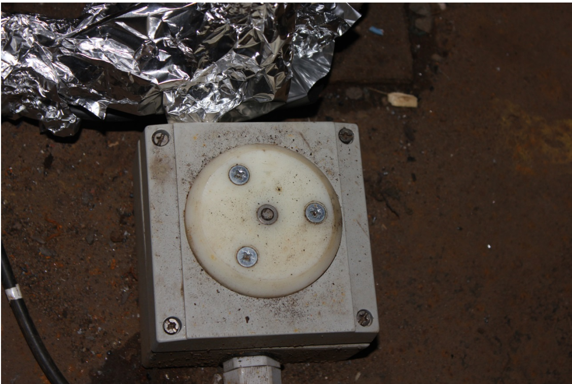
Figure 3-39 Piezoelectric pressure transducer in weatherproof box
