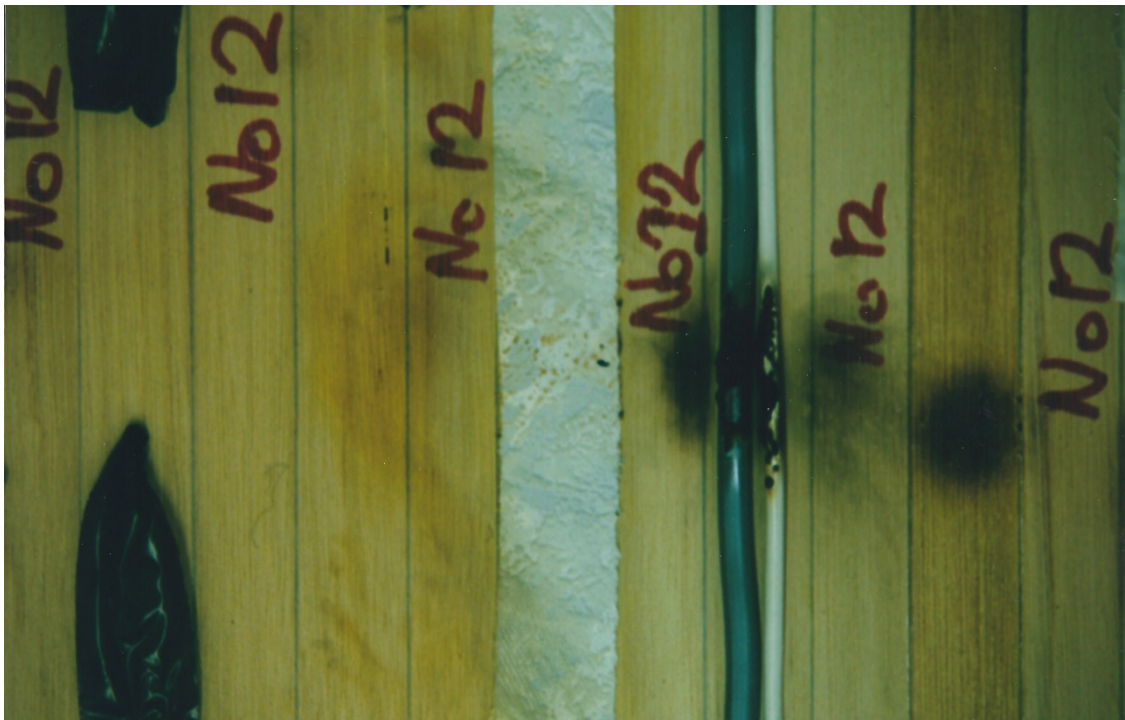
Figure 6-13 Thermal damage to electrical cable (Spadeadam, Rig C)
