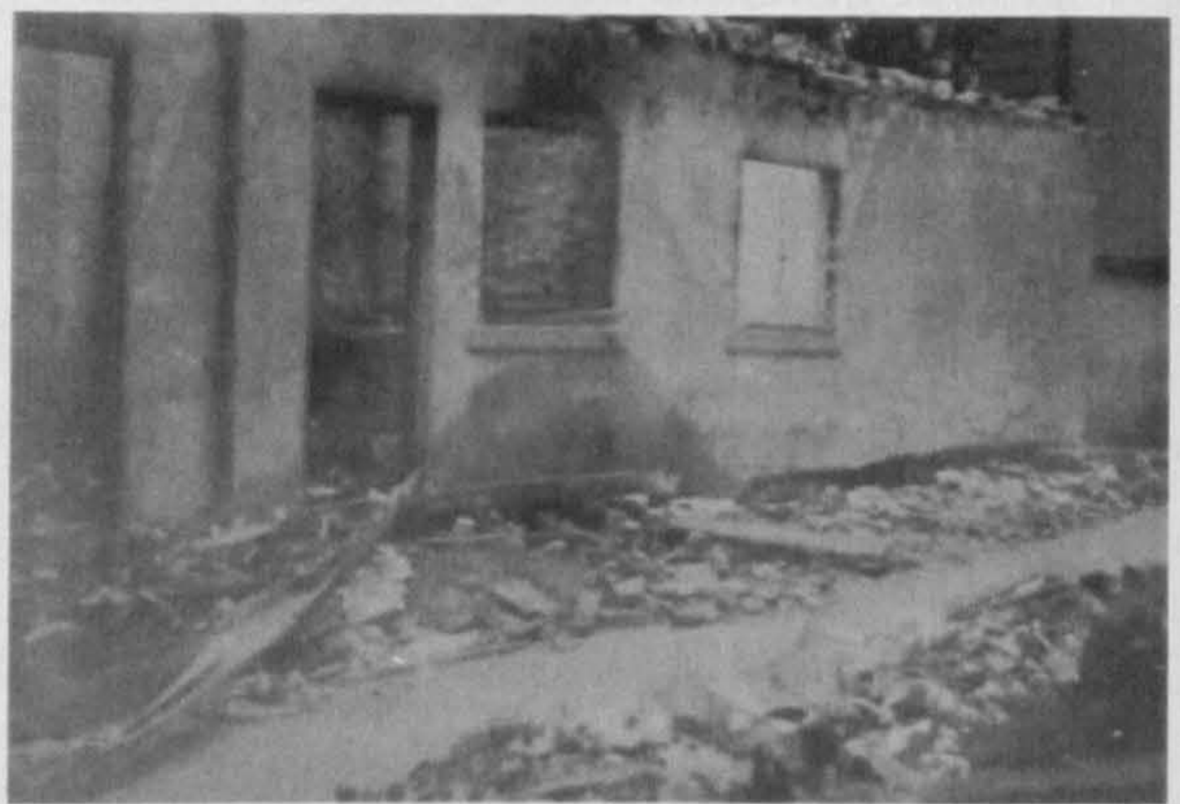
[ill.6: 27] CanTon Consulate, damaged Consul-General's house. Interior. Source: 1948-1949, WORK 10/301, date: 1948
